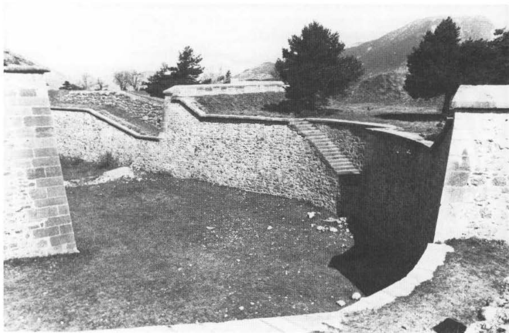
51 Redoubt in a place of arms at Mont-Dauphin, showing 'mouse steps' leading from the ditch
