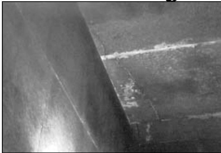
Cracks in granite beams in ceiling of King's Chamber 1992
