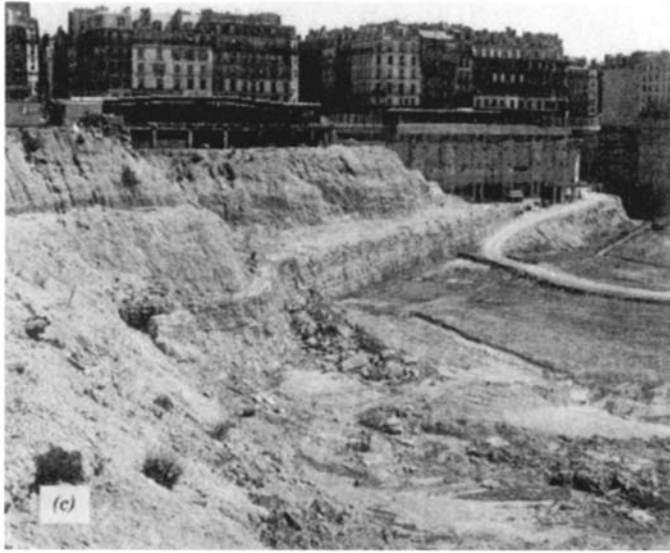
Fig. 1-18 The Halles Forum Project, Paris: (a) soldier piles and concrete lagging; (b) buttress-type slurry wall on piles; (c) slurry wall on piles. Anchorages were used for lateral bracing. (Bachy)
