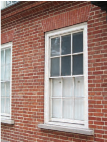
Timber window flush with brickwork of terraced houses at Newington Green, London built in 1658.
