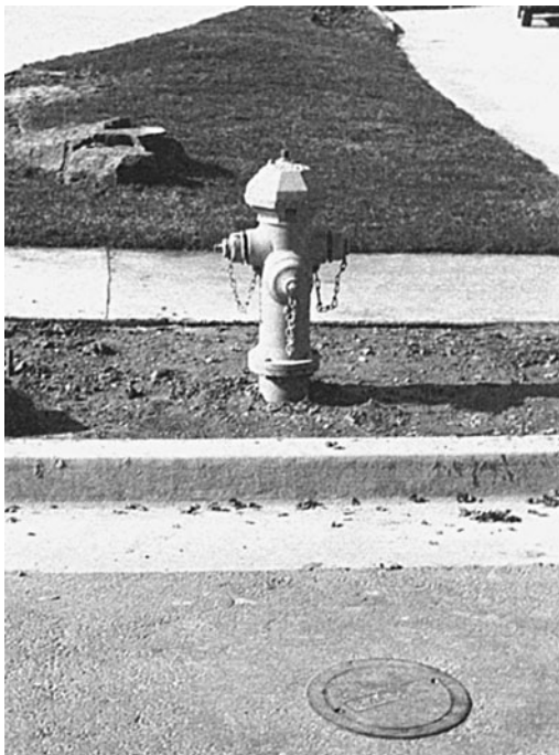
Figure 11.8 Fire hydrant with gate valve.
