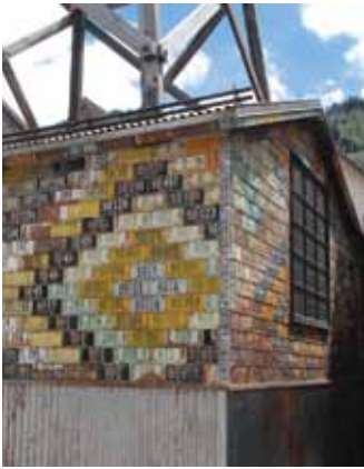
License plate shingling in Telluride, Colorado. This follows an older practice by miners of using tin cans for shingles.
