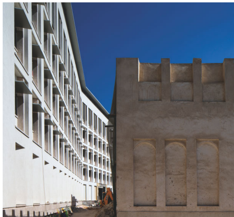
Interface between new construction and an existing heritage structure at Msheireb Downtown Doha. A new urban space is created in between the buildings.
