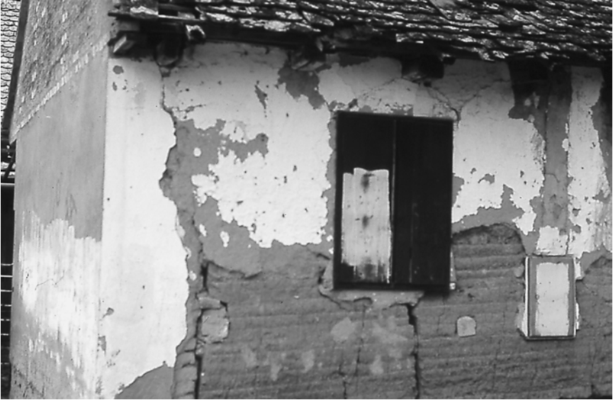
8-10. With little or no bell casting, the stucco wall plaster of this cottage near Osieja, Croatia has deteriorated and washed away because of the ground splash of rain. The adobe layers of the wall are exposed, and if not plastered again will begin to erode (photo by the author, 2004).
