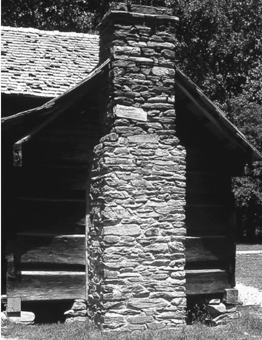
11-2. Good example of an exterior stone chimney attached to a log house. A variety of boulders and flat fieldstones have been used. A lime mortar binds the stone. Note also the large boulders upon which the sills of the house rest. Located in Cades Cove, TN (photo by the author, 1972).
