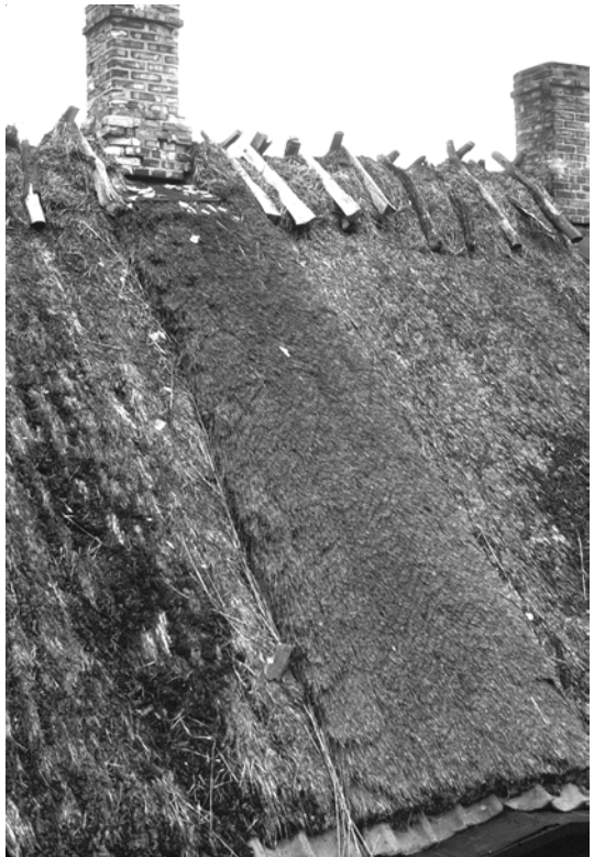
8-4. Pairs of roof trees hold down the critical thatch over the ridge of a cottage in the Jutland peninsula of Denmark, near Ringsted (photo by the author 1978).
