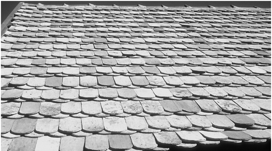
8-6. A "fish scale," flat shingle, tile roof in Holloko, Hungary. Rounding off the butt end of the tiles reduces the danger of wind lifting (photo by the author, 2002).
