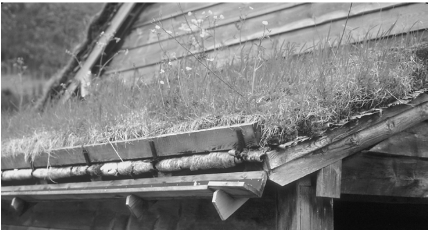
8-7. The cross-board helps to keep the upper sod layer of this roof firmly in place. The birch bark layer can be seen clearly above the lowest, sawn board layer, near Trondheim, Norway (photo by the author, 2001).
