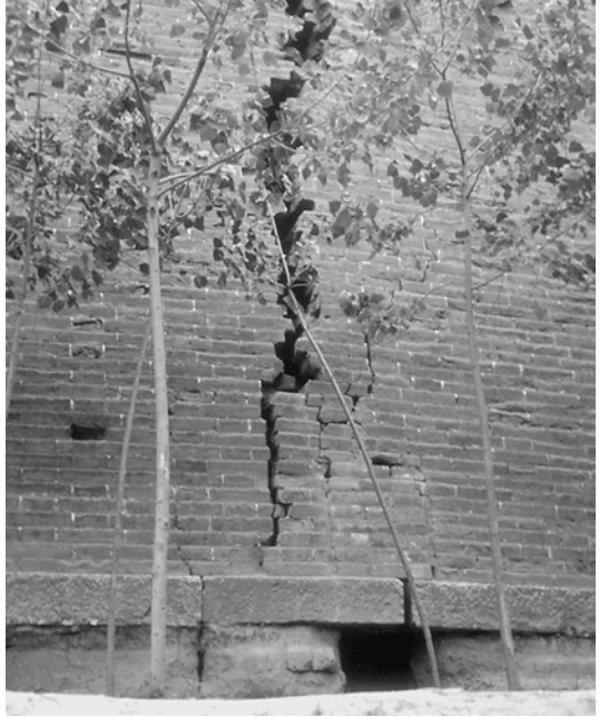
9-5. Damage to a compound wall, resulting from a severe earthquake in the 1970s in Sian, China (photo by the author, 1977).
