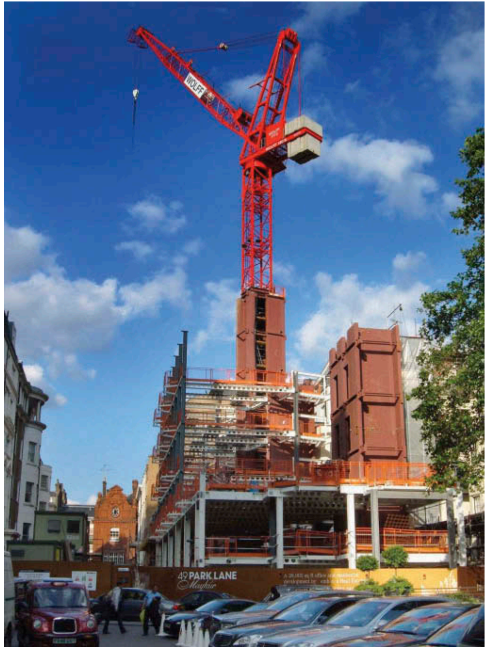
26.5 Innovative use of a tower crane mounted on top of a prefabricated steel core, used on an extremely confined inner city site
