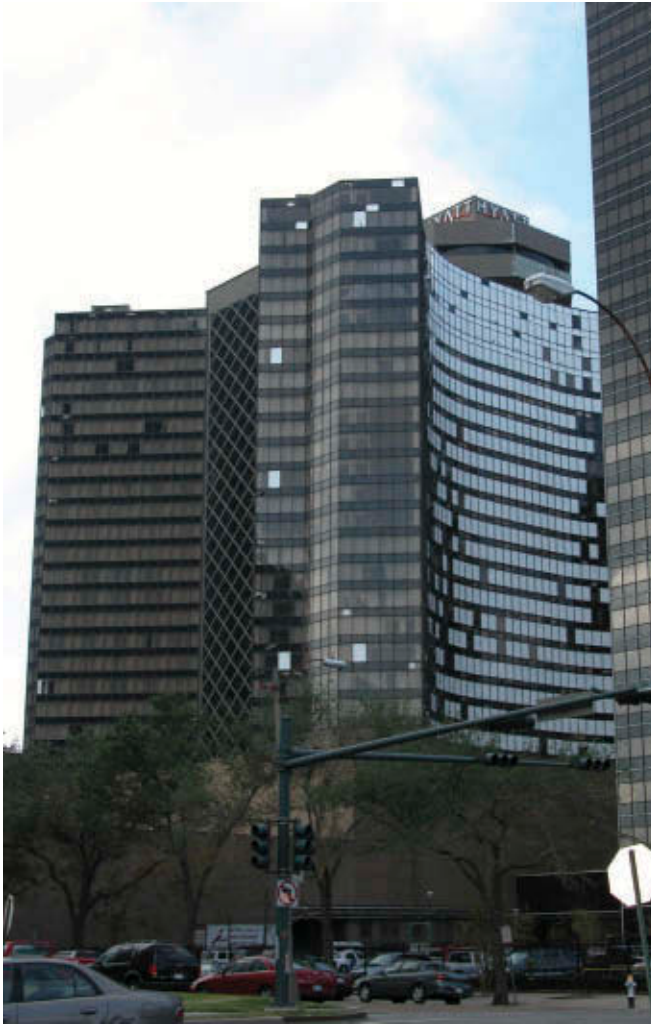
15.3 Damage to the building envelope of the 26-story Hyatt Regency Hotel in New Orleans Business District caused during the 2005 hurricane Katrina. Broken windows allowed rain and debris into the building resulting in additional damage
