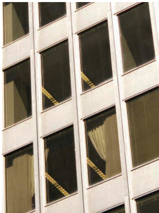
5.4 Mid-century modern facades such as this one have large, single-pane, dark-tinted glass
