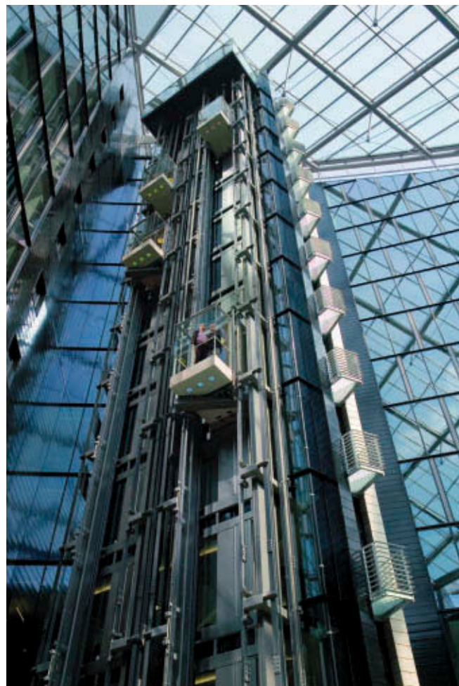
25.4 Although not yet in widespread use, ThyssenKrupp's TWIN™ system offers designers a unique alternative to more traditional solutions Image: ThyssenKrupp
