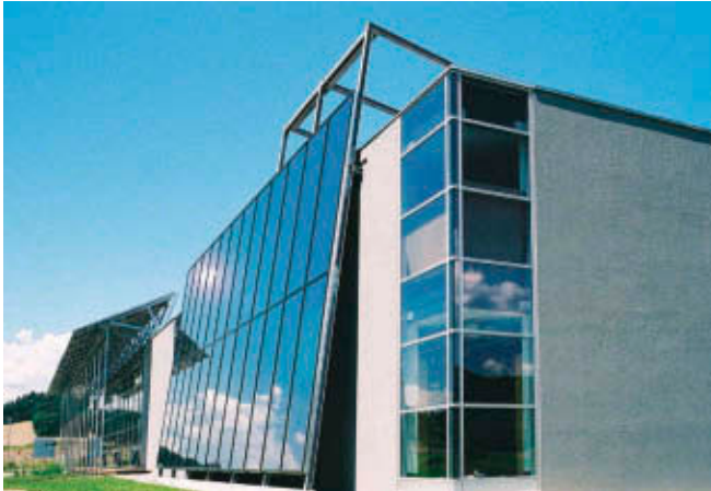
13.3 Solar thermal collectors are now available as facade-mounted systems Image: © Sonnenkraft
