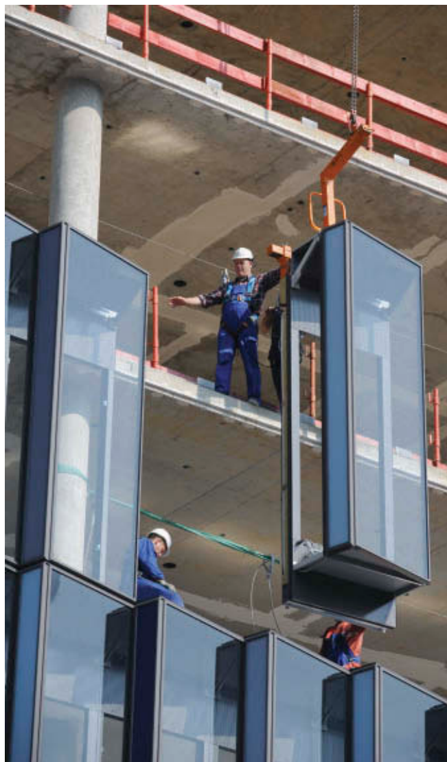
22.6 Mounting of prefabricated facade panel with a monorail crane at the KfW Westarkade building in Frankfurt am Main, Germany.
