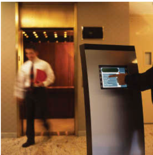
25.1 Destination-based dispatcher systems have revolutionized circulation design in modern high-rise buildings
