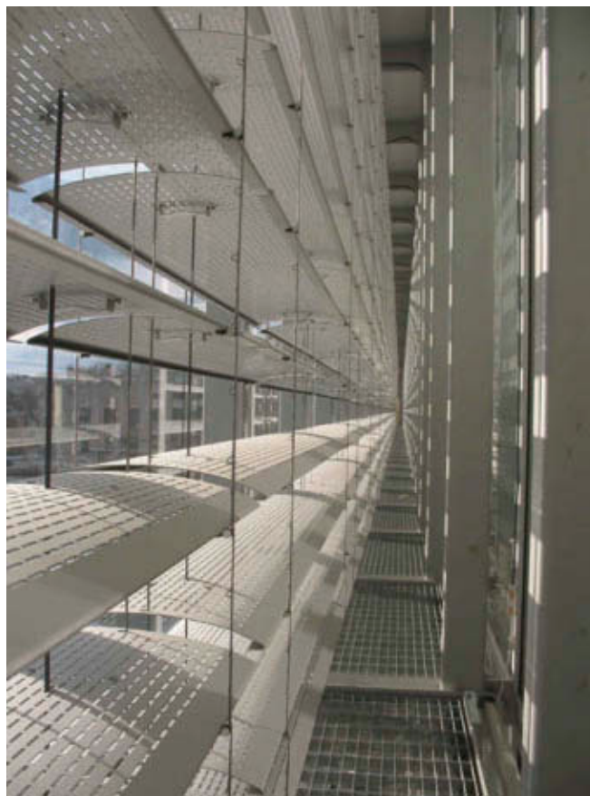
12.1 Cambridge Public Library facade interior. In a double-skin wall, dynamic climate control devices can be integrated with MEP strategies to improve building energy performance, daylighting, and exterior views Image: © William Rawn Associates
