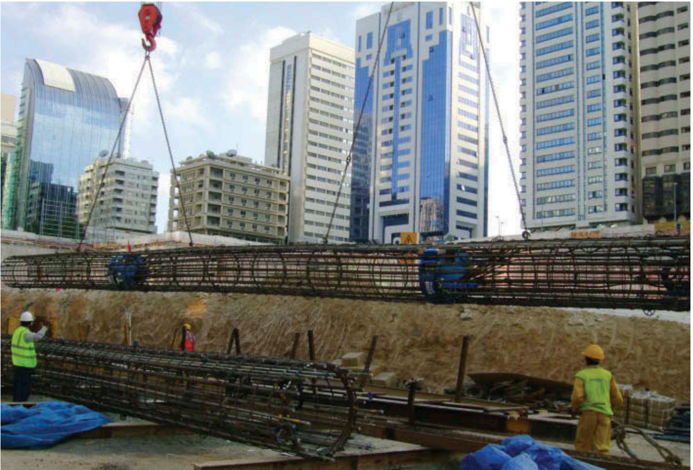
18.4 Reinforcing cage with four bi-directional load cells embedded at two levels for a 96 MN load test at the Central Market project in Abu Dhabi, United Arab Emirates
