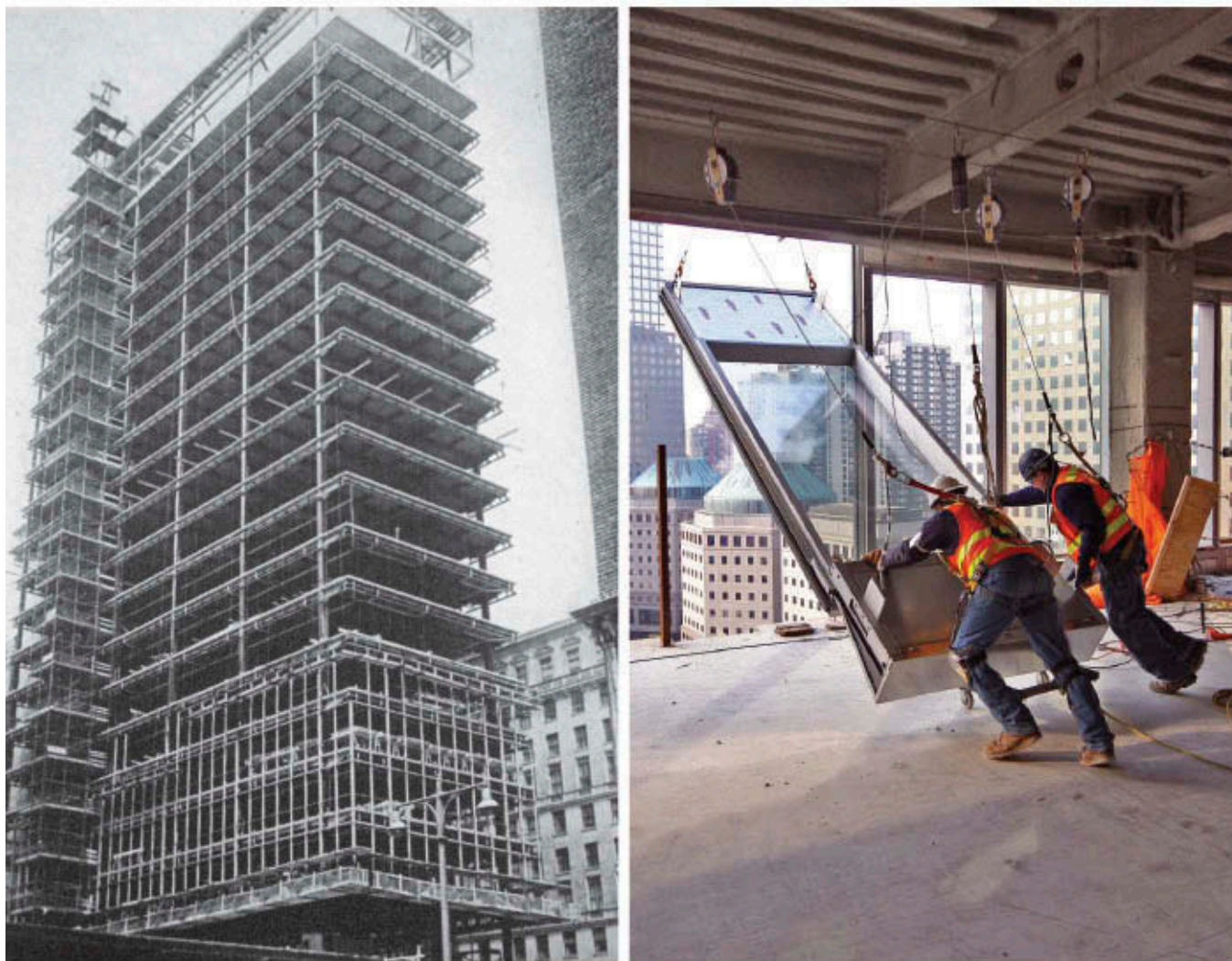
21.3 The two most basic curtain wall systems, stick and unitized, differ in the ways they are manufactured, assembled, and installed. A stick system was used for Lever House (left), while One World Trade Center (right) has a unitized curtain wall system
