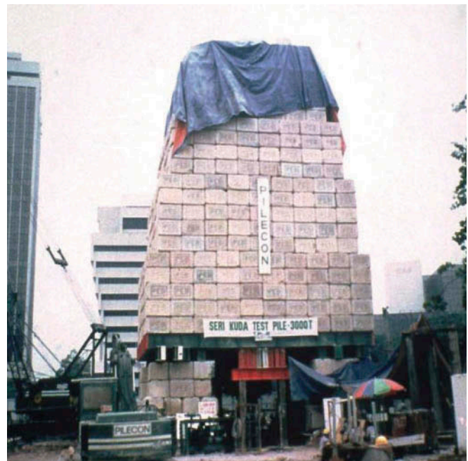
18.3 A 30 MN kentledge load test conducted for the Petronas Towers in Kuala Lumpur, Malaysia
