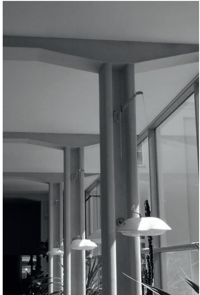
Illustration 4.23 Gothenburg Law Courts, Gothenburg, Sweden (1937). Column-to-beam connections in central hall. Steel structural elements are encased in concrete. This is an example of a fixed connection. Architect: Gunnar Asplund.
