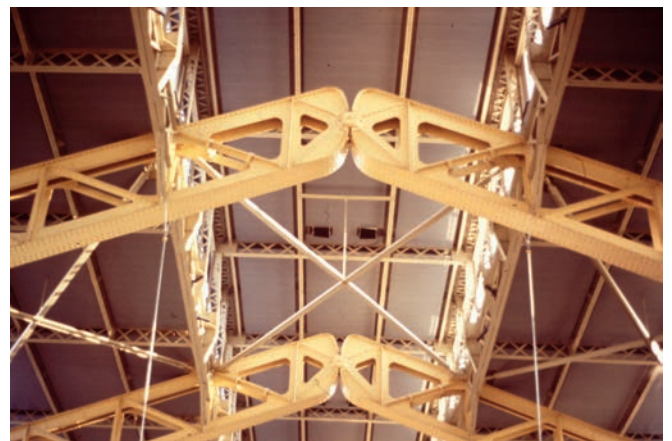
Illustration 12.24 Abattoirs de la Mouche. Hinge detail at apex of the arch that expresses ability of structure to rotate freely; trussed form of arch elsewhere expresses its ability to resist bending as well as compression.
