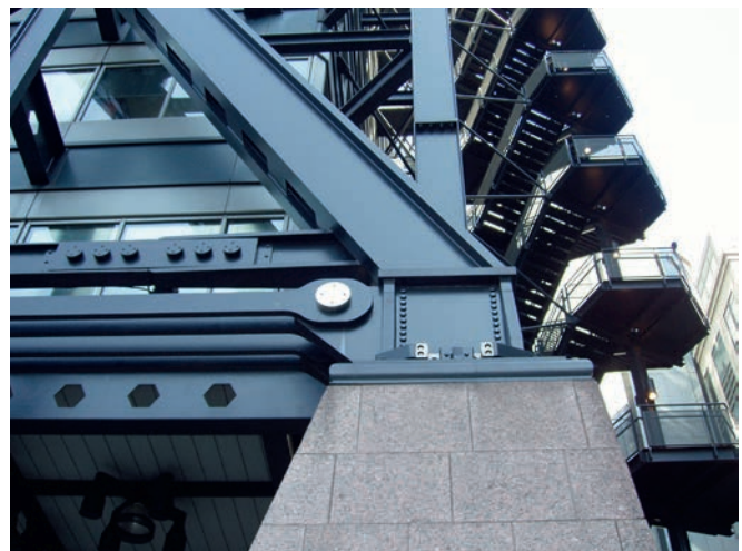
Illustration 6.29 Broadgate Exchange House. Detail of arch base support showing horizontal tension tie that counters arch's outward thrust.
