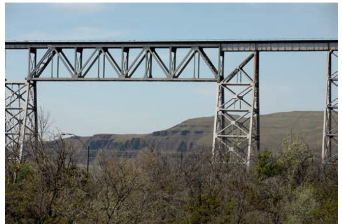
Illustration 9.9 Joso High Bridge over Snake River, between Franklin and Walla Walla counties, WA, USA, (1914). The similarities and differences between a truss and a beam with no openings in its steel-plate web are evident: both here have to carry the same transverse train loading, but the truss is able to use its strategic triangulated configuration of its component parts in order to span a much greater distance between supports.
