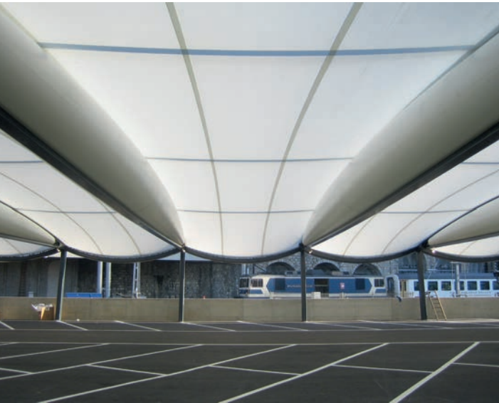
Illustration 11.52 Montreux Parking Garage. View from below canopy; series of air-inflated membrane beams span across space; doubly curved fabric membrane spans between them.
