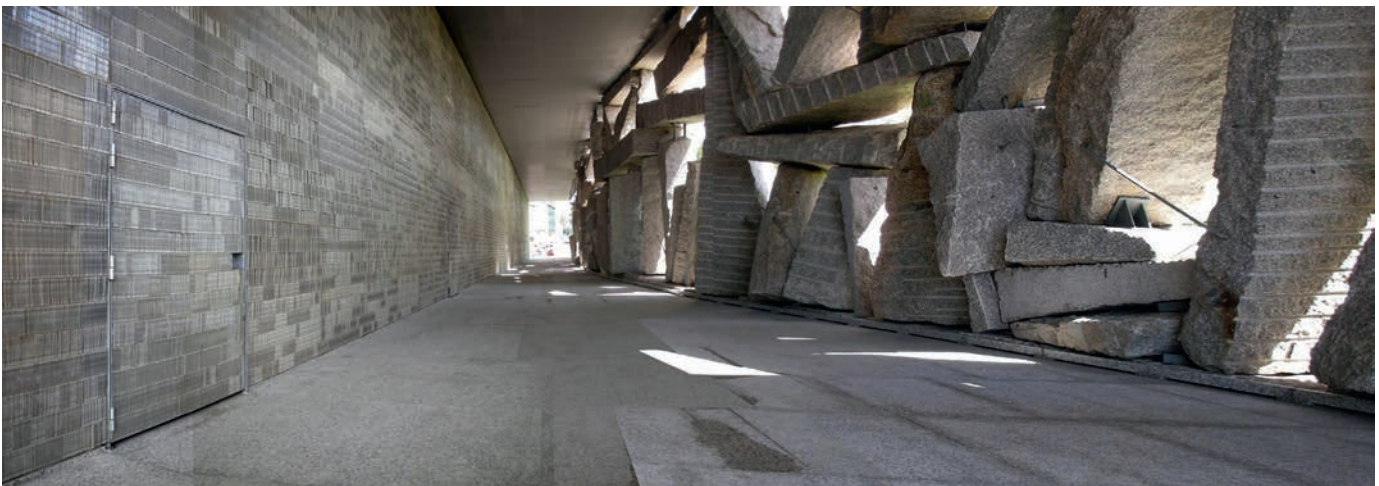
Illustration 5.24 SGAE (General Society of Authors and Publishers) Central Office, Santiago de Compostella, Spain (2008). Contemporary stone wall, forming outer edge of covered walkway. Seemingly “random” arrangement is actually carefully balanced, then held together by steel rods. Architect: Ensamble Studio.
