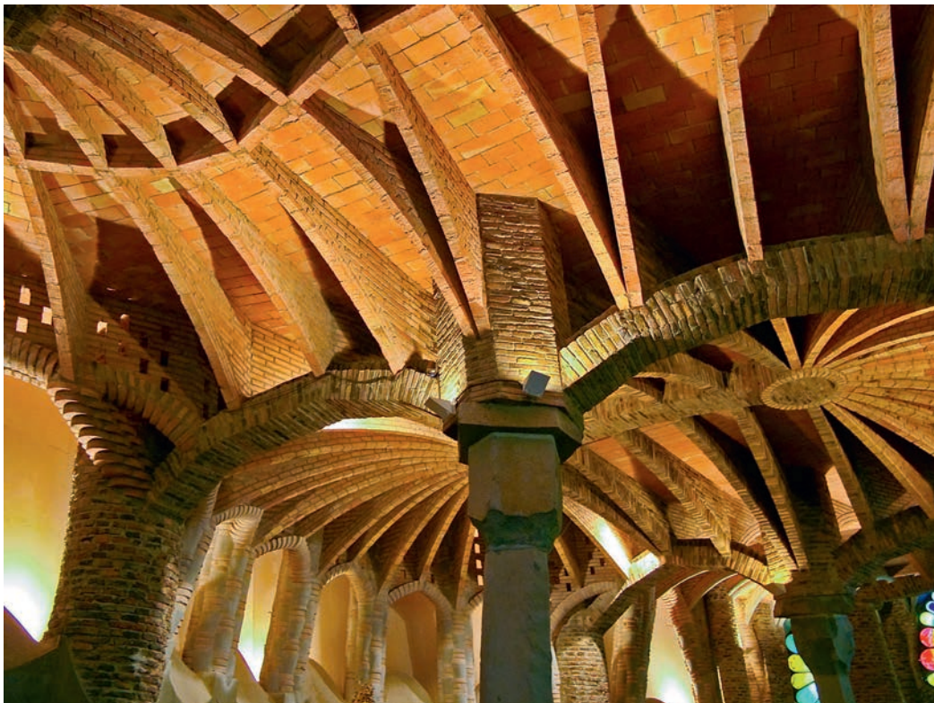
Illustration 12.18 Colonia Güell Chapel. Unusually angled arch forms established from hanging chain model so as to favor their being in "pure" compression and minimizing bending as much as possible.
