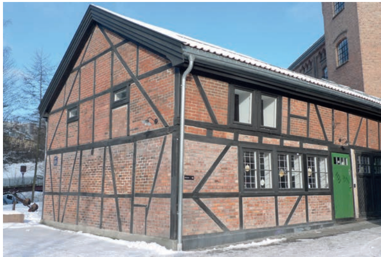
Illustration 3.26 Akers Mechanical Workshop and Factory, Oslo, Norway (1841). The sideways-displacement effect of wind pressures and suctions acting on a building has long been known, as is indicated by the presence of diagonal bracing members within frameworks of vernacular timber construction. The brickwork here is infill that is unconnected to the frame and is used only to create enclosure, rather than contributing to lateral load resistance.
