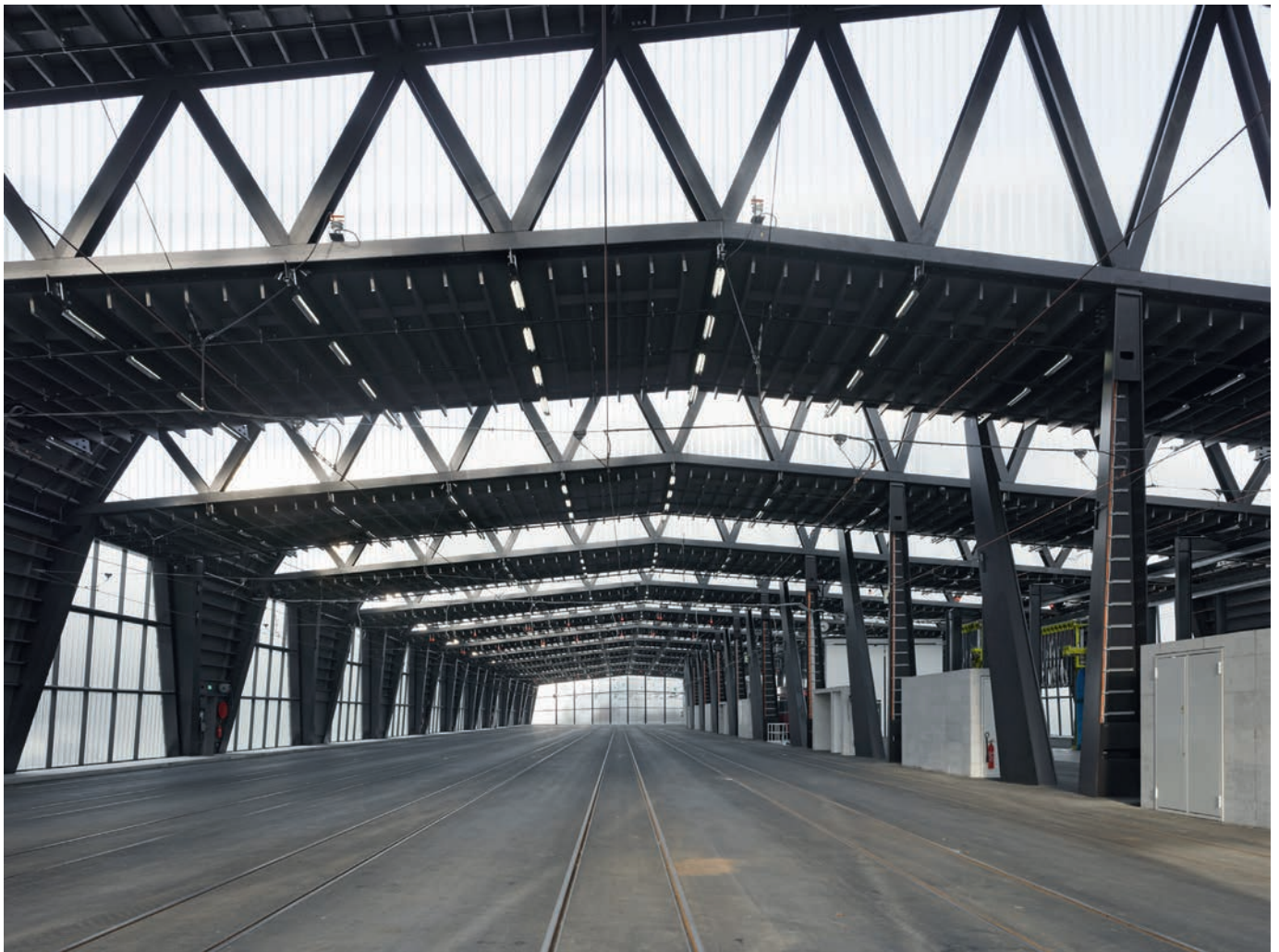
Illustration 9.32 Neue Tramdepot Bern. Interior view of space, with natural daylight penetrating through relatively open trusses.
