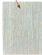
Figure 16.23 The “best” portion of the scored concrete material is captured in a rectangle.
