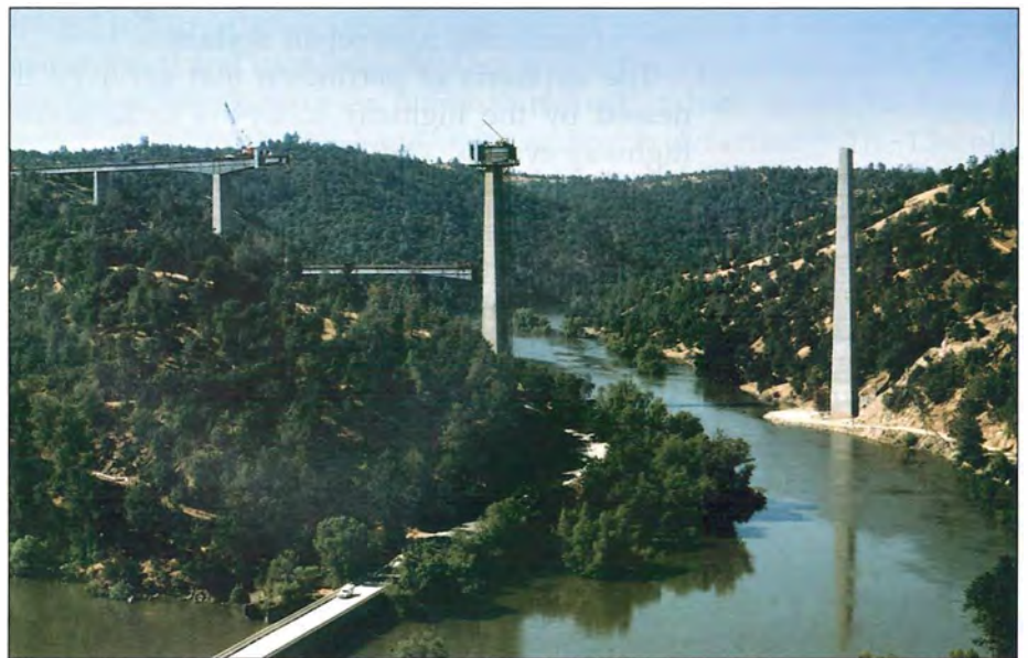
Figure 18.2 Along California’s Mokelumne River. Here the new road, now completed, soars above the valley as if to deny topography. Below, the old road winds where once ferries operated across the flood.
