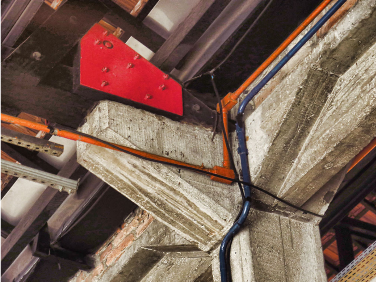
Cabling detail, SESC Pompeia ( Photo Calabrese )
