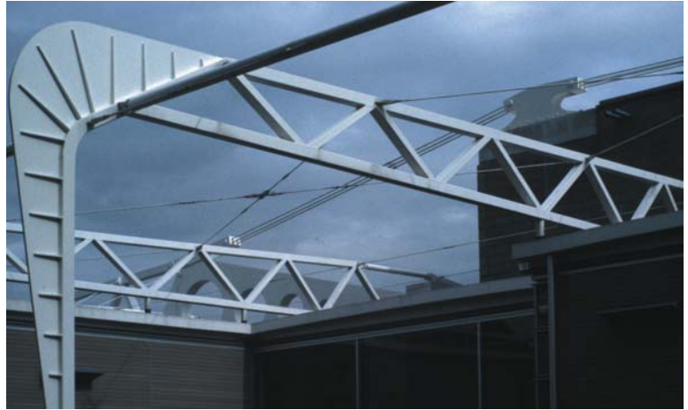
▲ 2.6 Innovatively detailed portal frame columns, with the core and an 'anvil' support for the trusses in the background.
