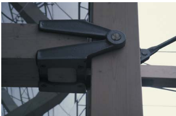
▲ 7.31 A beam-column connection where a horizontal gap between the castings allows for a down-pipe to pass through the detail where required.
