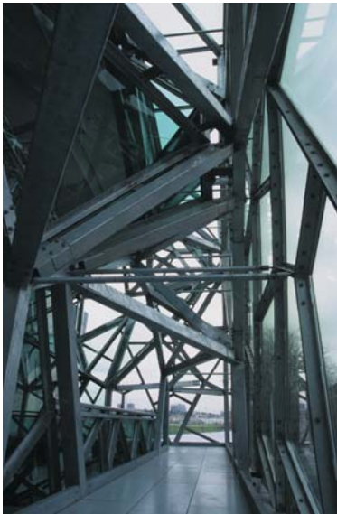
▲ 9.28 A perimeter walkway through the wall structure of the BMW Edge amphitheatre.
