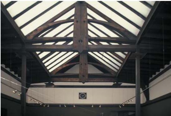
▲ 7.33 Glasgow School of Art, Scotland, Charles Rennie Mackintosh, 1899. Truss forms inspired by medieval construction.
