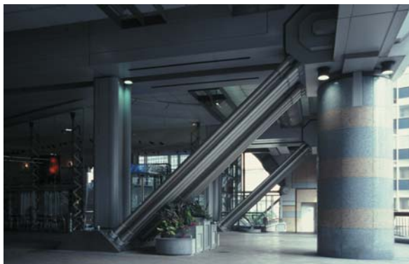
▲ 5.38 125 Alban Gate, London, England, Terry Farrell, 1992. A transfer-truss diagonal member poses a potential danger to passers-by.
