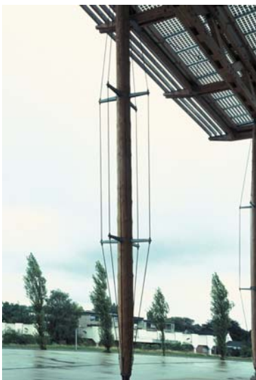
▲ 4.26 Mont-Cenis Academy, Herne, Germany, Jourda & Perraudin, 1999. The front canopy structure is almost identical to that of the interior.
