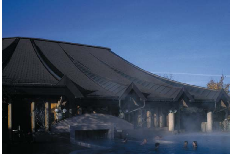
▲ 3.33 Sântispark Health and Leisure Centre, St Gallen, Switzerland, Raush, Ladner, Clerici, 1986. Creased and sagging roof.
