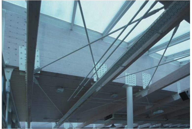
▲ 8.33 Business School, Öhringen, Germany, Günter Behnisch & Partner, 1993. A primary beam with the skylight above and the roof below.
