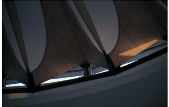
▲ 6.2 Refined timber struts connect to the steel rod tension-ring and the rafters with deepened ends.
