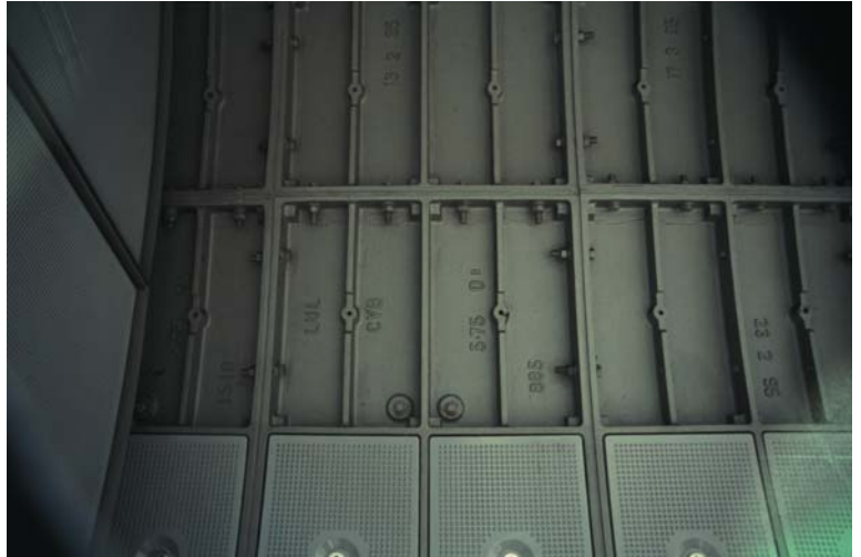
▲ 6.32 Westminster Station, London, England, Michael Hopkins & Partners, 1999. Tunnel lining exposed at a platform.
