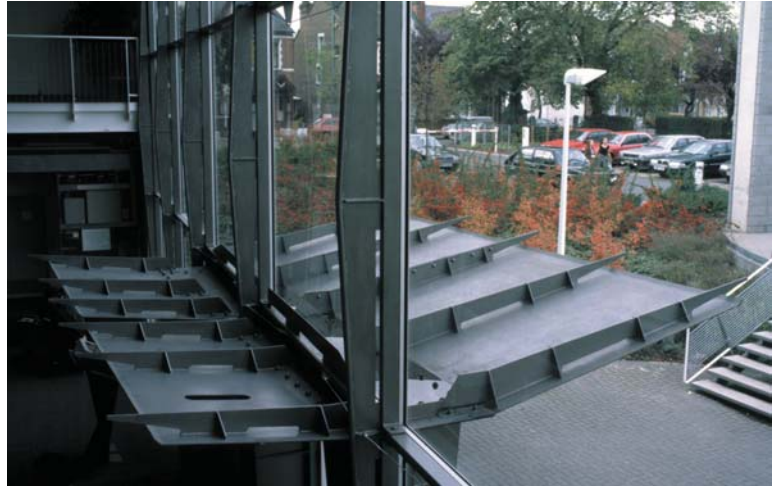
▲ 2.9 Refined structural detailing in the atrium and to the main entrance canopy.
