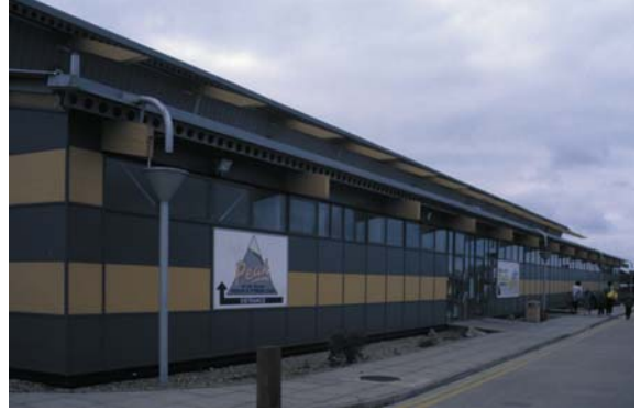
▲ 4.43 Splash Leisure Centre, Sheringham, England, Alsop & Lyall, 1988. Wall-to-foundation detailing conveys a lack of grounding.
