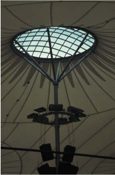
▲ 8.1 Stellingen Ice Skating Rink and Velodrome, Hamburg, Germany, Silcher, Werner + Partners, 1996. Daylight enters the junction between the flying-strut and the fabric membrane.
