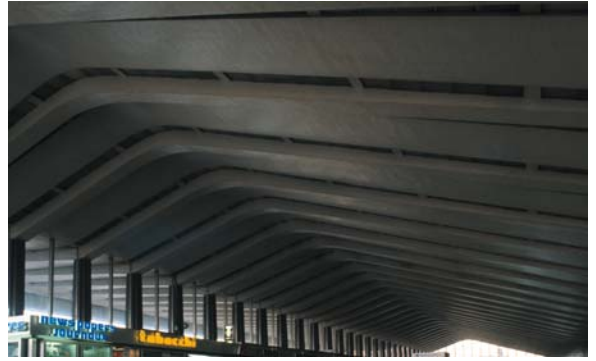
▲ 3.45 Stazione Termini, Rome, Italy, Montuori, Vitellozzi, Calini, Castellazzi, Fatigati & Pintonello, 1950. Curved roof beams over the main concourse.
