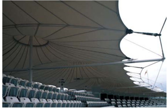
▲ 8.35 Mound Stand, Lord's Cricket Ground, London, England, Michael Hopkins and Partners, 1987. Underside of the fabric roof.
