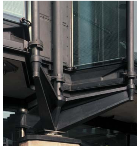
▲ 4.41 Metal columns, a cantilever bracket and a stainless steel rod behind a stone pier.
