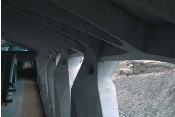
▲ 8.11 Recessed lights in stub columns.
