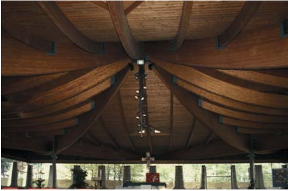
▲ 6.28 Notre Dame de la Duchère, Lyons, France, F. Cottin, 1972. Posts supporting the roof are barely discernible.
