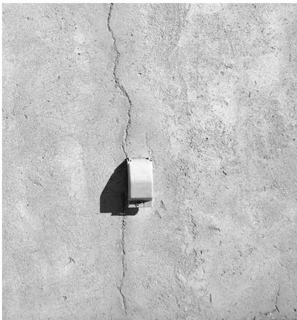
6-4a. Telegraphing crack.
