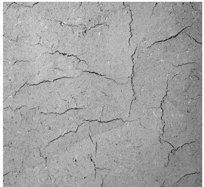
6-4b. Depth cracks.
