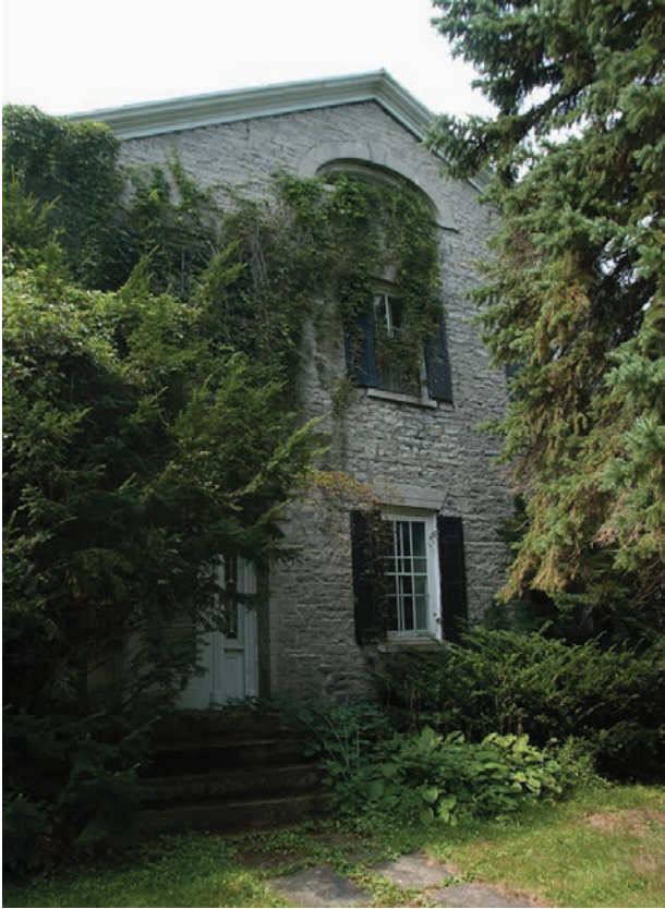
7.20. The Tisdale Mansion, built in 1832, has a front gable entrance that is well sequestered from the street.
