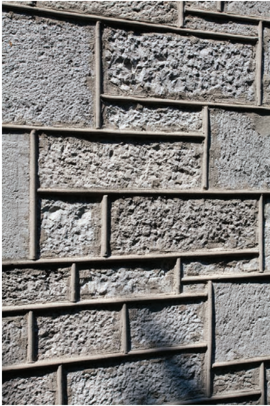
3.2. Hungerford Mansion. The stone on the side of the mansion is a mixture of rough cut with smooth cut around the windows.
