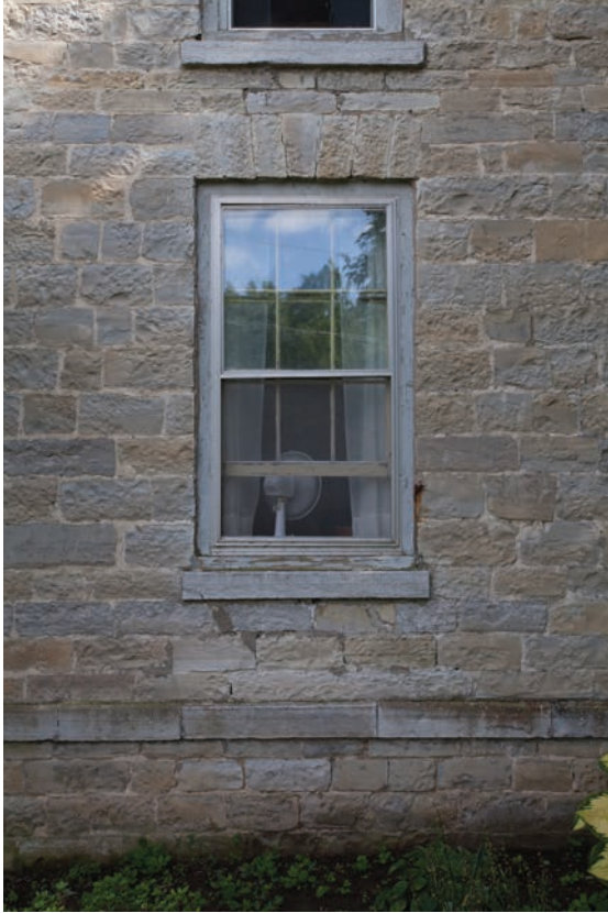
10.27. The side window of the David Dodge House is set in the well-laid stone wall with voussoirs and a water table.
