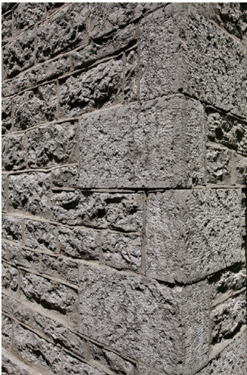
6.14. The corner quoins of the Oliver Bates House are particularly well cut and placed in the evenly coursed walls.
