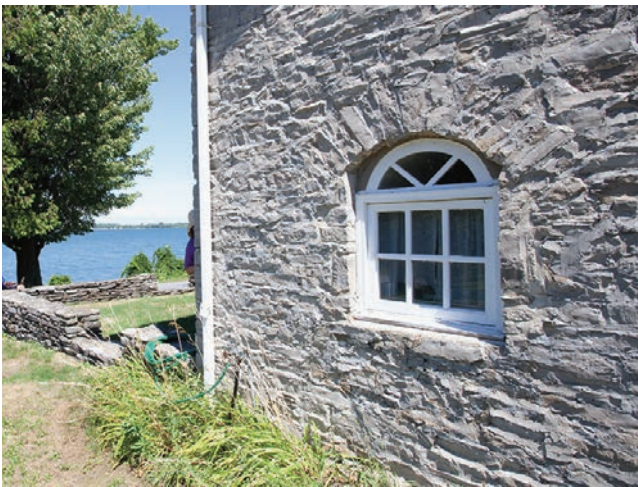
9.7. A coffin window was put into the side wall of the William Johnson House, probably because the tight interior layout demanded it.
