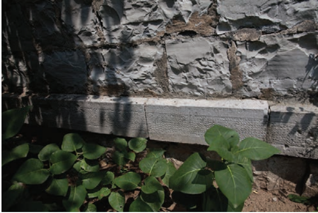
17.17. Harger Mansion. The smooth finished water table contrasts with the rough-cut stone of the wall.
