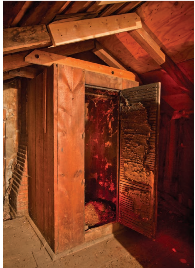
2.10. Felt Mansion. A smoke chamber for curing meats is attached to the second floor ell chimney.
