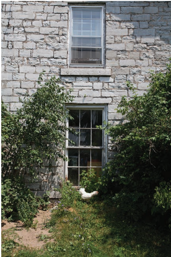
17.15. Harger Mansion: side windows with lintels and sills of Black River limestone of the Pamelia formation.
