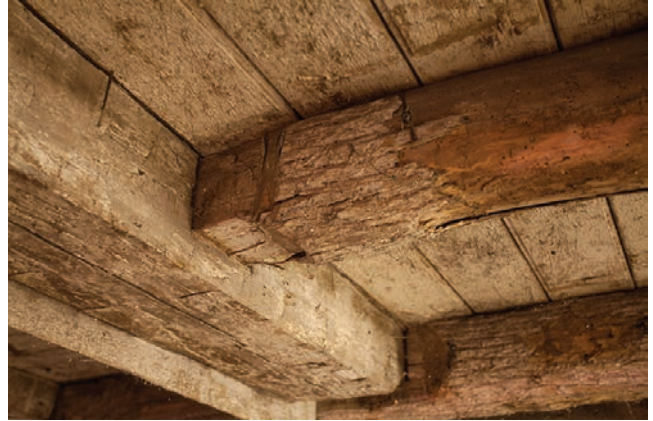
6.7. The cellar beams of the Burnham House are hand hewn, with much bark still in place.
