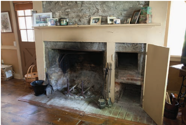
1.12. Asa Gates House. Kitchen fireplace, with a beehive oven on the right.
