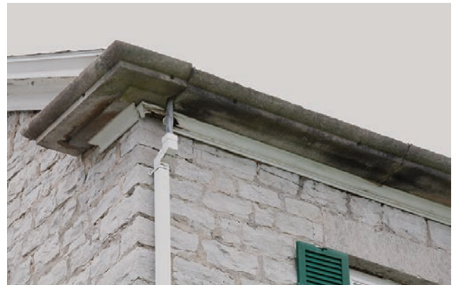
1.8. The limestone gutter of the Noadiah Hubbard House is held in place with iron pins.
