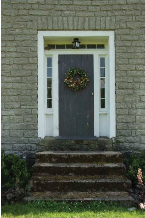
10.13. The front entrance of the Dezenegremel House shows off the even quality of Ignatius Wiley's stonework.
