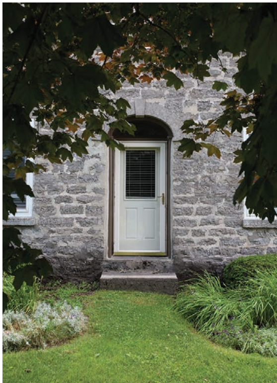
6.12. The narrow entrance to the Harvey Smith House retains its rounded arch and keystone set in the coursed rubble wall.
