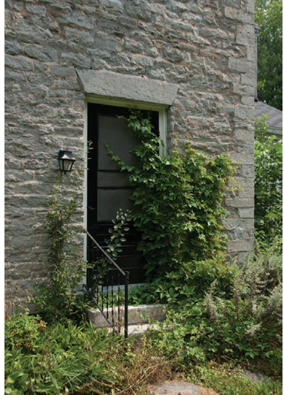
7.21. The rear wall of the Tisdale Mansion is of rubble with smooth quoins and lintel.
