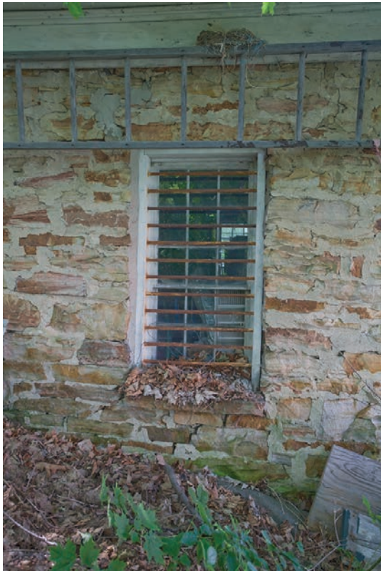
14.10. Window of the Theresa Jail, which is no longer used as a holding facility.
