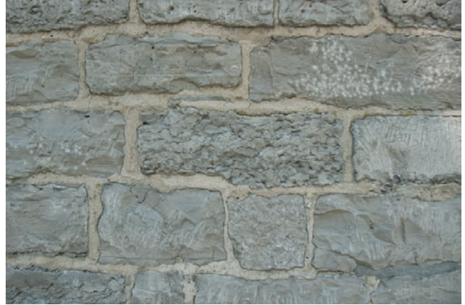
10.7. Limestone of the Trenton Group, Rockland Formation, on the front of St. Vincent of Paul Church. The mason's tool marks can be seen on some stones.
