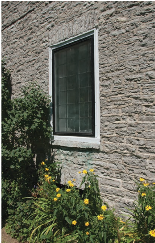
10.18. The side casement window of the Peugnet House is topped with voussoirs.
