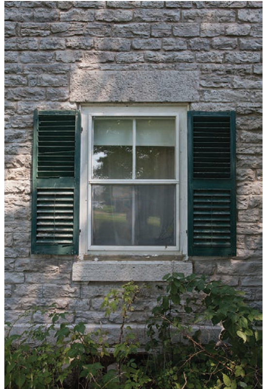
9.16. A side window of the Charles Wilcox House shows the smooth lintel and sill with the expressed water table below.
