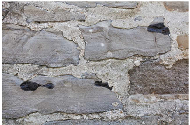
9.8. The William Johnson House was built of local limestone with black chert nodules.
