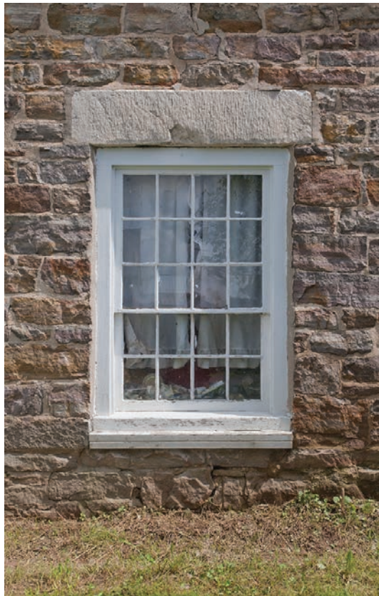
15.5. Like other windows of the Ira Hinsdale House, the 12/8 kitchen window has a large limestone lintel set in the sandstone of the wall.
