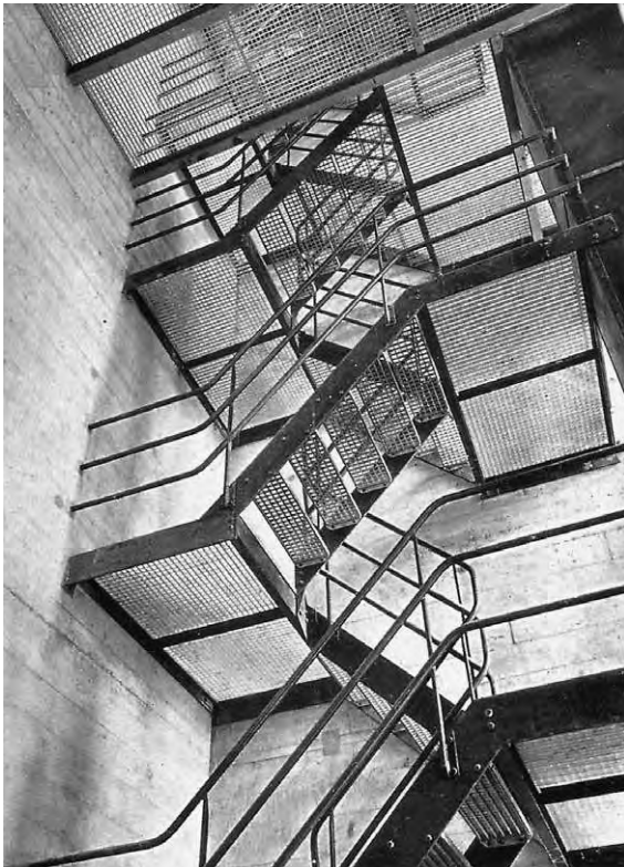
Figure 7.2d Typical RSJ framing: escape stairs, Technical High School, Basle, 1931, Architect: Otto Salvisberg (from Schuster, F., Treppen , Hoffman Verlag, 1949)
