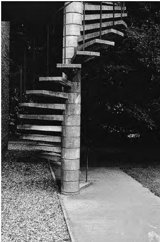
Figure 8.4c Artificial stone finish to spiral stair (courtesy of Cornish Spiral Stairs Ltd)
