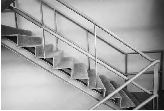
Figure 7.3a Folded steel stairs: Providing builders access as skeletal frame is erected and then used permanently
