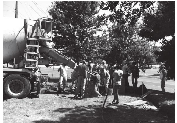
FIGURE 3 Pavilion earthwork and foundation installation by students and faculty (Credits: Hans Curtis Herrmann)
