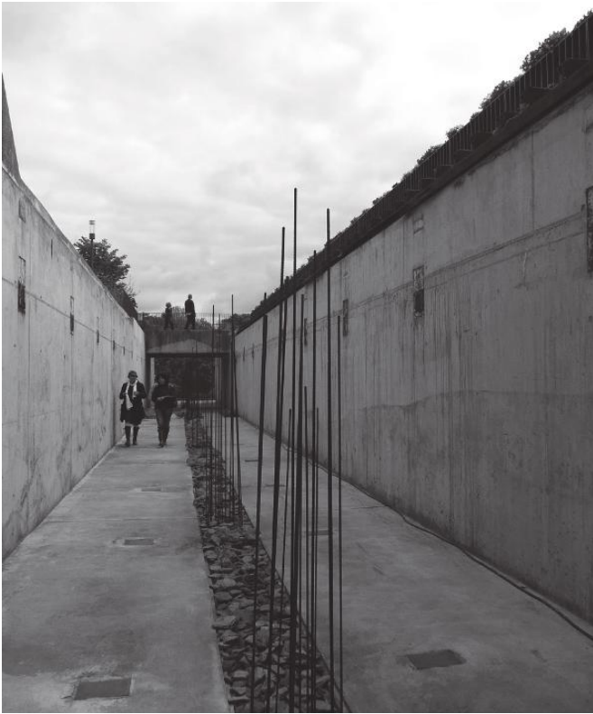
FIGURE 2 Built on sugar: sunken garden in the former channel with the conveyer belts
