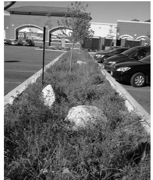
Figure 10-30 Bioretention swale collects and filters stormwater runoff from parking surfaces and facilitates groundwater recharge.
