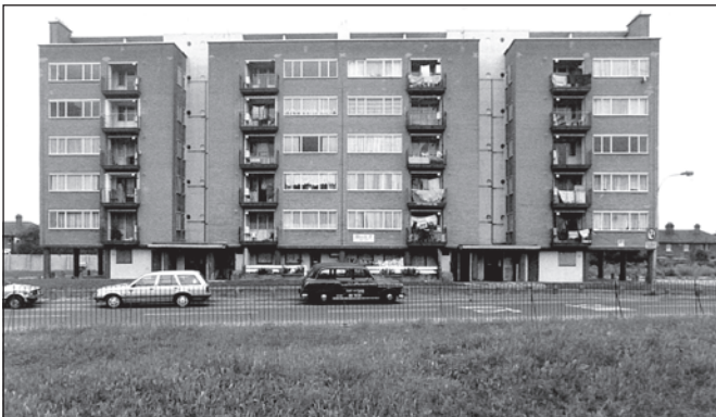
One of the unimproved blocks which had deteriorated into poor condition
