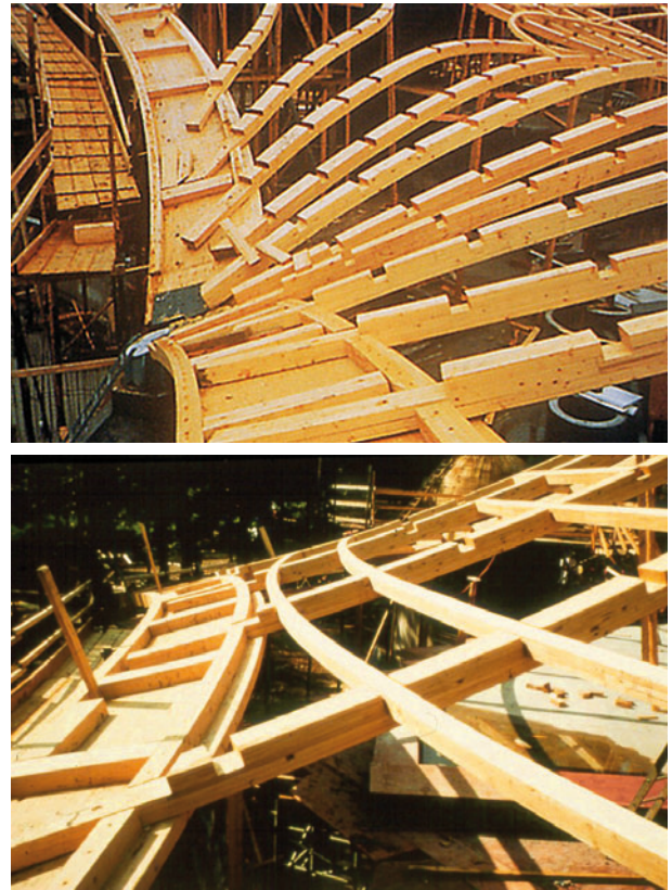
Figure 12.9 (top) Meridian ribs with cross lap joints, attached to the edge beam, and (bottom) overlaid with the annular ribs
