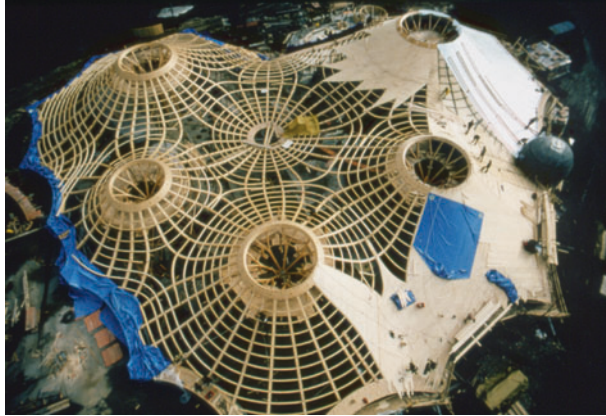
Figure 12.7 Construction site with all ribs assembled and placement of covering boards and sheeting
