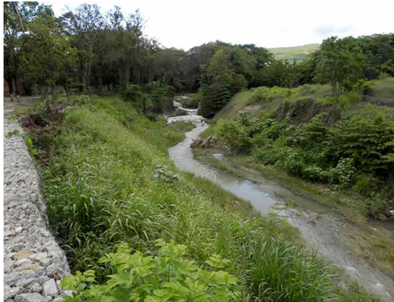
FIGURE 7.9 A stretch of the Rio Sabinal showing bank erosion and stabilization.
