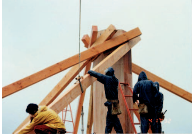
▲ 5.6 Friction connection – the New Farmhouse RF building by Yoichi Kan under construction. (Photo: Yoichi Kan.)
