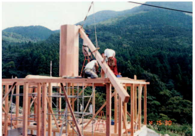
▲ 8.19 More beams are positioned around until a full circle is formed. (Photo: Yoichi Kan.)
