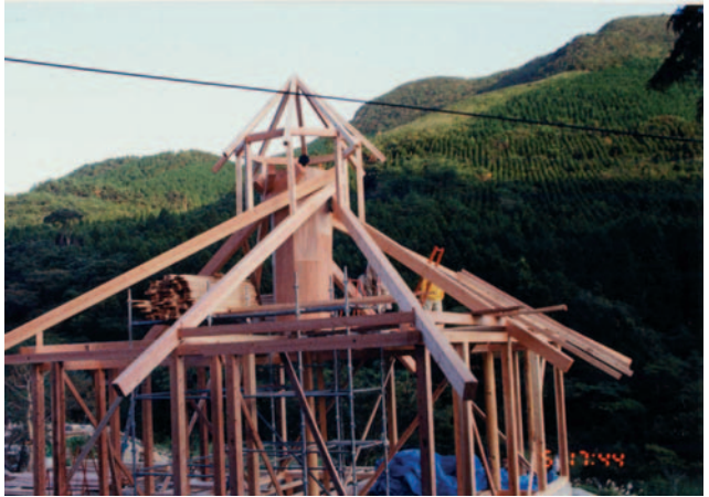
▲ 8.20 The RF structure becomes stable when all the beams are installed. (Photo: Yoichi Kan.)
