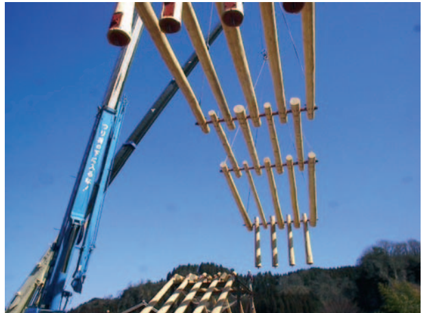
▲ 7.59 The pinned timber structure folds and is locked into its final position. (Photo: Kazuhiro Ishii.)
