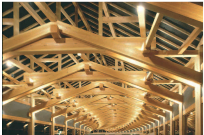
▲ 7.54 The roof structure of the shop and café building is a type of RF structure – internal view. (Photo: Kazuhiro Ishii.)
