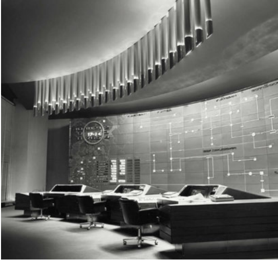
fig. 2 Control Center of the Electricity grid for the North-west regions of the USSR designed by Maris Gundars, Soviet Republic of Latvia, 1974–1976. Photograph by Laimonis Stipnieks.
