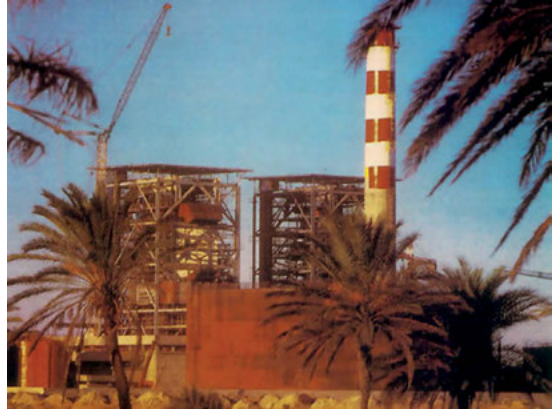
fig. 9 PARTERV company, power plant constructed within TESCO labor exchange framework in Sousse, Tunisia, 1970s. Photo courtesy of TESCO Archive.
