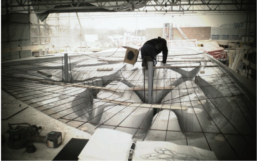
The Unikabeton project set out to explore the architectural and industrial potential in linking topology optimization of concrete structures with large scale CNC-milling of polystyrene formwork. Image illustrates assembling and reinforcing the full scale CNC-milled polystyrene mold. (Courtesy Per Dombernowsky and Asbjørn Søndergaard)
