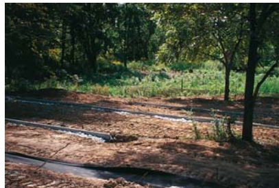
Trenches channel the water from streets and parking areas.
