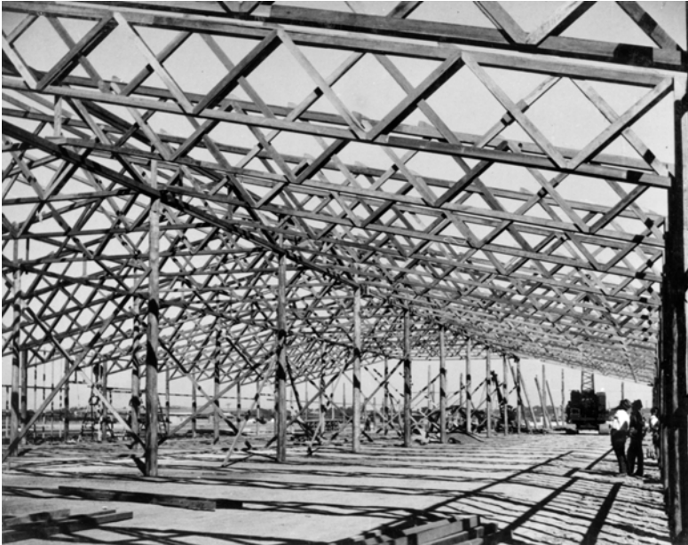
Figure 5. Erection of prefabricated framework. Three hundred feet of roof trusses were erected in six days by 12 men. Meeandah – Warehouse construction. July 1943. (Item 53.3/3.4, box 18, series B5281, National Archives of Australia.)
