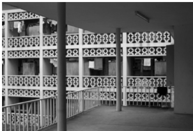
Figure 1. Fry, Drew and Partners University of Ibadan, Nigeria 1947–1951. Dormitory blocks in 2002 (photograph by Hannah le Roux).
