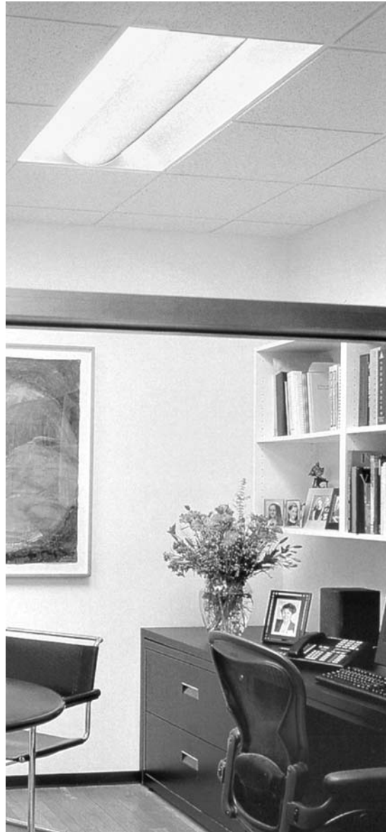
Figure 10-51. An upgrade to standard lay-in fluorescent fixtures. Although it has considerable brightness, it provides indirect light. This is the type of fixture indicated in Figure 10-50, Option A. (Photo courtesy: Focal Point, L.L.C., Chicago, IL.)
