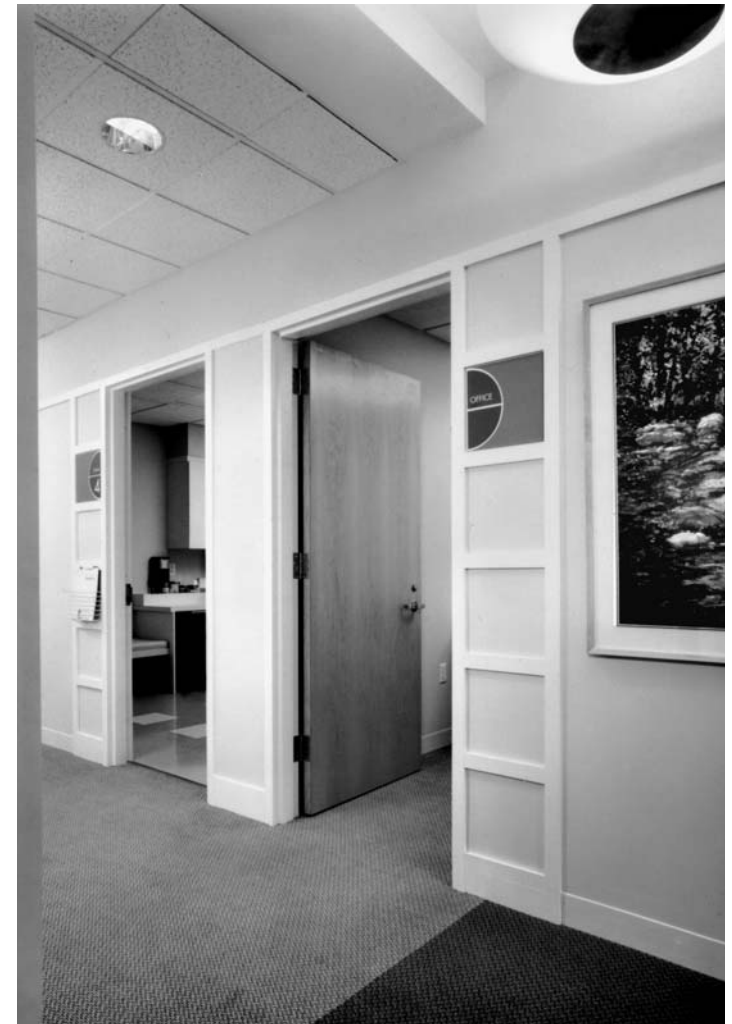
Figure 6-15. Modular signage panel alongside doors is both functional and attractive. Frisbie Memorial Hospital, Rochester, NH. (Photo courtesy: TRO/The Ritchie Organization, Newton, MA; Photographer: Edward Jacoby Photography.)
