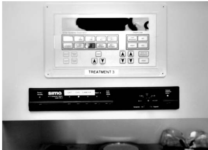
Figure 10-46. Communication system and AV control panel built into 12 o'clock wall. (AV consultant: Mr. Hookup, San Diego; Photographer: Jain Malkin.)
