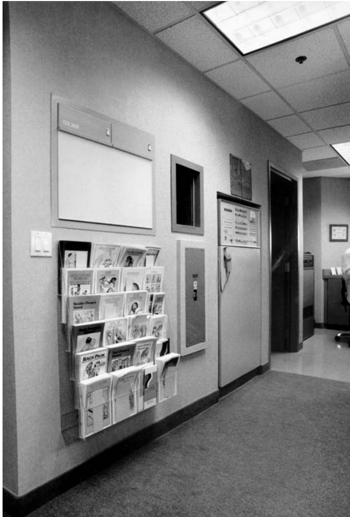
Figure 4-134. Tech work area. Control (generator) for X-ray unit is outside room. Lead glass window provides view into X-ray room. Emergency electrical shutoff panel located here. Automatic processor and tech viewing area can be seen in rear. Note: This photo shows an older-model film processor, but it is illustrative of a film-based tech work area. A brochure rack makes it easy for tech to distribute relevant literature to patients. (Design: Jain Malkin Inc.; Photographer: John Christian.)
