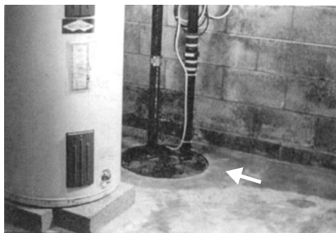
PHOTO 14.16 A sewage ejector. (Used with permission of ABC)
