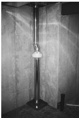
PHOTO 3.19 A subfloor depressurization system used to reduce radon levels by ventilating a crawl space below a structural basement floor. (Used with permission of ABC)
