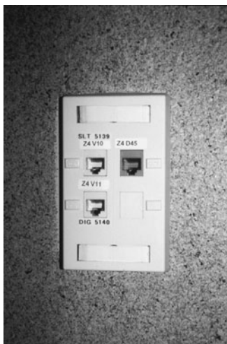
PHOTO 22.19 A telecommunications outlet with coded female connectors. (Used with permission of ABC)
