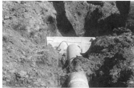
PHOTO 16.1 A community storm drainage line before placement of backfill. (Used with permission of ABC)
