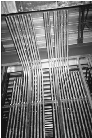
PHOTO 19.35 Conductors for each circuit extend through conduits from the main panelboard (under construction). (Used with permission of ABC)
