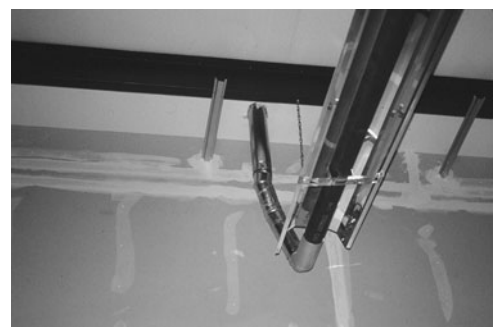
PHOTO 6.16 Combustion products from the infrared heater tube are exhausted through a roof vent. (Used with permission of ABC)
