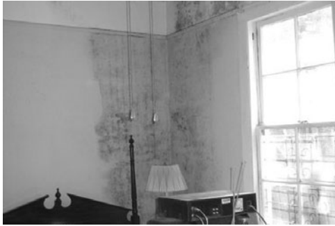
PHOTO 3.17 Evidence of mold growth caused by small leaks and inadequate airflow. (Courtesy of DOE/NREL)
