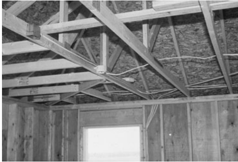
PHOTO 19.15 Rough wiring of branch circuits extends through framing to outlets. (Used with permission of ABC)
