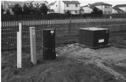
PHOTO 19.3 A power transformer (right) steps down distribution voltage to building system voltage (120/240 V). The power pedestal (at center right) is where the connection is made before being fed to the residence through the service entrance conductors. (Used with permission of ABC)
