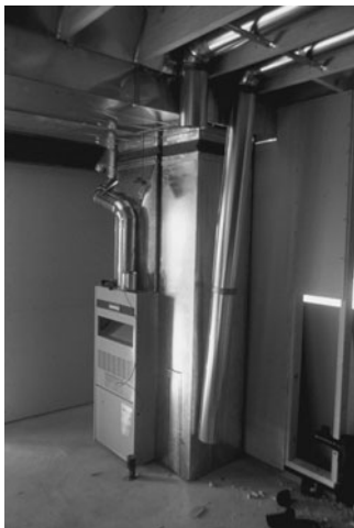
PHOTO 8.1 An upflow furnace installation. The supply air plenum (above furnace) carries heated air to the rectangular main duct or trunk suspended from the ceiling. Return air recirculates back to the furnace in the rectangular return air duct, also suspended from the ceiling (in foreground). Main ducts are isolated from the furnace with a flexible duct connection that allows movement and isolates furnace vibration. Round ducts on the side of furnace introduce air for combustion. (Used with permission of ABC)
