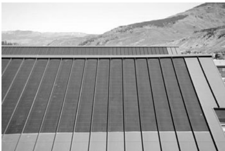
PHOTO 25.22 BIPV shingles at the BigHorn Home Improvement Center retail complex in Silverthorne, Colorado, with a design capacity of 8 kW. (Courtesy of DOE/NREL)
