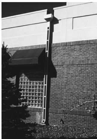
PHOTO 16.6 An exterior roof drainage system. Storm water from the low-sloped roof drains through openings in a parapet wall into funnel-like conductor heads at the top of the vertical conductor or downspout. The vertical conductor has an open face to prevent blockage from ice or debris. (Used with permission of ABC)
