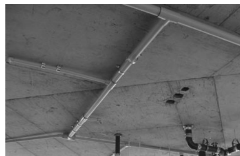
PHOTO 21.20 Chlorinated polyvinyl chloride (CPVC) pipe being installed as sprinkler pipe. It will be serving a dwelling unit in a high-rise condominium building. (Used with permission of ABC)
