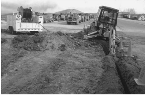
PHOTO 19.1 Underground electrical distribution lines serving a residential development being buried in a trench. (Used with permission of ABC)
