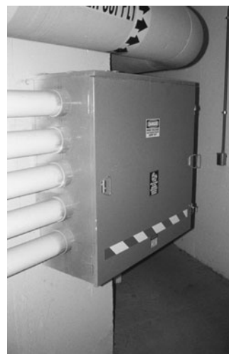
PHOTO 18.20 A large junction box. (Used with permission of ABC)
