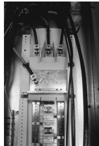
PHOTO 19.31 Three feeders from the main distribution panel (see Photo 19.26) connected to lugs in the panelboard (see Photo 19.30). The lugs connect to the three bus bars to which circuit breakers are connected. The fourth conductor (left side of photograph) is the grounding conductor, which connects the panelboard ground to the main distribution panel near the service entrance. (Used with permission of ABC)
