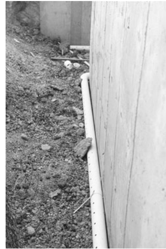
PHOTO 16.13 An exterior perimeter drain placed against a foundation wall during construction of a home. (Used with permission of ABC)
