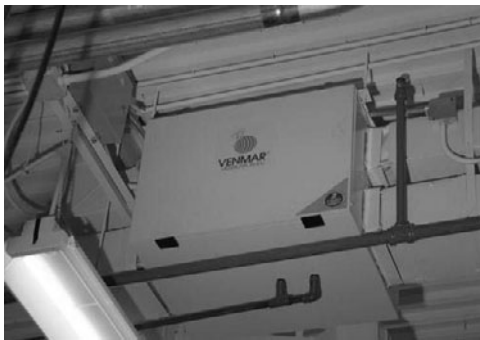
PHOTO 7.47 An air-to-air heat exchanger for ventilation air in a commercial application. (Courtesy of NREL/DOE)
