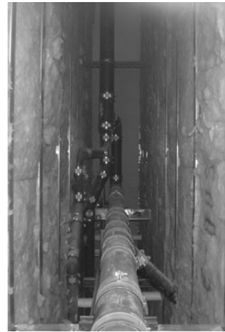
PHOTO 14.17 A view of the interior of a plumbing (wall) chase. DWV lines are cast iron (black). (Used with permission of ABC)
