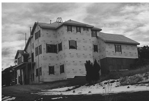
PHOTO 3.24 An installed air barrier wrapping the exterior sheathing before installation of the cladding (siding and masonry veneer). (Used with permission of ABC)
