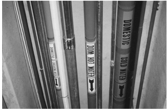
PHOTO 13.37 Properly marked domestic cold water, hot water, and hot water recirculating lines. (Used with permission of ABC)
