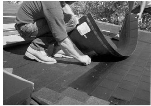
PHOTO 25.24 Installing flexible PV roofing shingles, rated at 17 W each. (Courtesy of DOE/NREL)
