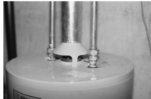
PHOTO 13.30 Plumbing connections to a residential storage tank water heater. Dielectric unions are used to minimize a galvanic reaction between the copper pipes and the water heater. (Used with permission of ABC)
