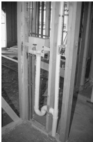
PHOTO 13.13 A rough-in of fixture branches and drain for a laundry connection. (Used with permission of ABC)
