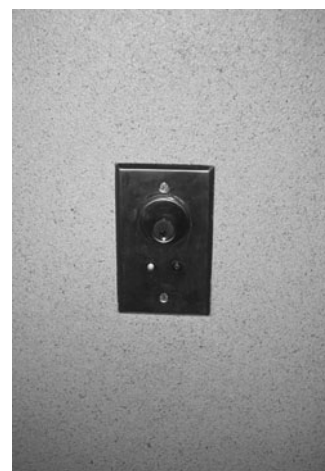
PHOTO 18.15 Keyed switch. (Used with permission of ABC)
