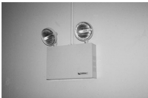
PHOTO 21.33 Emergency lighting with a remote battery backup for power outages. (Used with permission of ABC)
