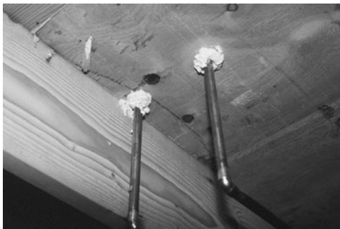
PHOTO 13.17 Sealed openings to prevent flanking of sound from a bathroom above. (Used with permission of ABC)
