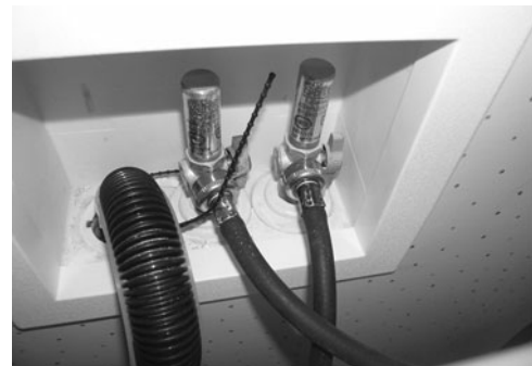
PHOTO 13.24 Water hammer arrestors (two) above shut-off valves at a clothes washing machine connection. (Used with permission of ABC)
