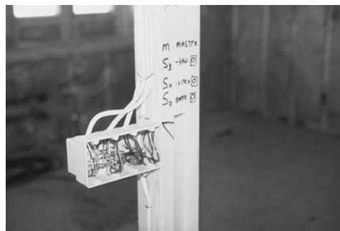
PHOTO 18.19 Switches in a four-gang nonmetallic electrical box. Nonmetallic (NM) sheathed cabling is entering the box. (Used with permission of ABC)
