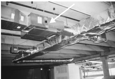
PHOTO 7.26 A terminal box branching off from an insulated main duct. (Used with permission of ABC)
