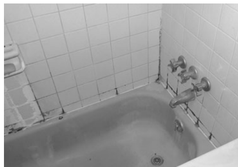
PHOTO 3.15 Evidence of mold growth in joints of bathtub surround tile. (Used with permission of ABC)
