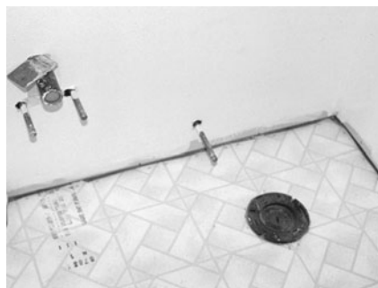
PHOTO 13.12 A rough-in of fixture branches for a lavatory and water closet. (Used with permission of ABC)
