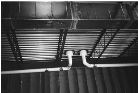
PHOTO 16.3 Conductors (pipes) on the underside of the roof surface carry storm water away from the roof drain. (Used with permission of ABC)
