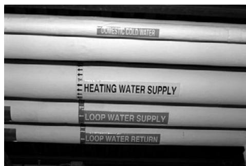
PHOTO 25.6 Loop water piping, part of the geothermal heat pump system at Cavett Elementary School in Lincoln, Nebraska. (Courtesy of DOE/NREL)
