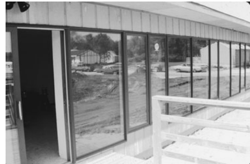
PHOTO 11.24 Double-glass windows covering thermal storage wall on the south side of the residence. (Used with permission from ABC)
