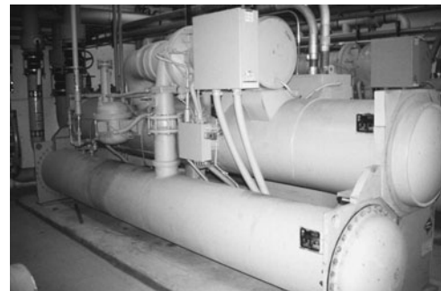
PHOTO 6.24 A commercial-size chiller is a water-cooled condensing unit. The slender tubes are fluid-to-fluid heat exchangers. (Used with permission of ABC)
