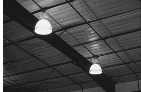
PHOTO 20.16 A low-bay HID luminaire. (Used with permission of ABC)
