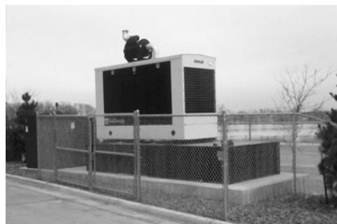
PHOTO 21.31 An emergency generator. (Used with permission of ABC)
