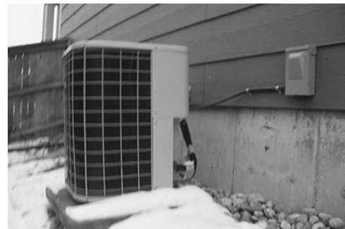
PHOTO 8.18 A pad-mounted condensing unit. Note the refrigeration lines connecting to the back side of the unit and the electrical box feeding power to the unit. (Used with permission of ABC)
