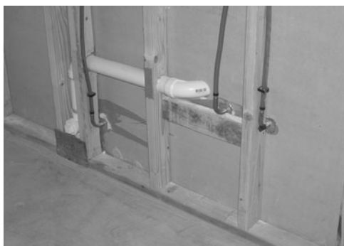
PHOTO 13.22 The backside of the terminating fitting at the end of runs of PEX pipe in the homerun water supply distribution configuration. (Used with permission of ABC)
