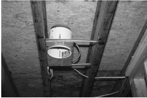
PHOTO 20.13 A recessed light fixture during construction. After it is secured to the joists, placement of the fixture can be adjusted (left to right). (Used with permission of ABC)
