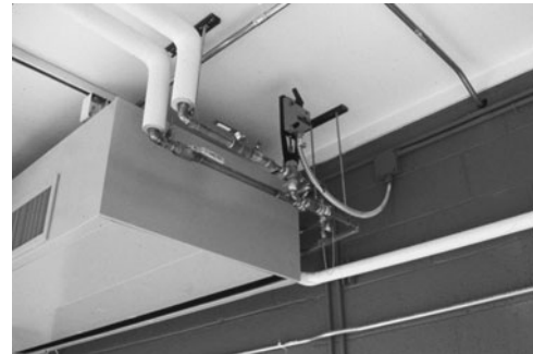
PHOTO 7.37 Pipes connected to the coil of a fan-coil unit. Note the automatic control valve. (Used with permission of ABC)
