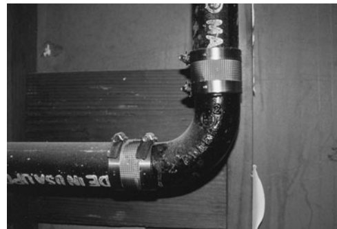
PHOTO 12.5 Cast iron pipes and elbow connected with compression fittings. (Used with permission of ABC)
