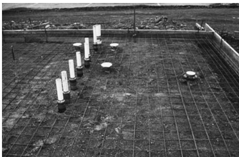
PHOTO 14.10 Placement of drain lines (tall pipes), water closet flanges, and floor drain (far right) before a concrete floor is cast. Note that the pipes are covered with an expansion material to isolate them from the concrete slab. This will prevent damage to the pipes that could be caused by movement of the concrete floor slab. (Used with permission of ABC)
