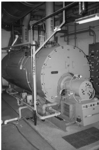
PHOTO 6.1 A commercial-size, hot water fire tube boiler. (Used with permission of ABC)
