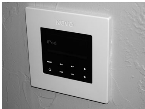
PHOTO 22.22 A residential computerized control panel with IPOD capabilities. (Used with permission of ABC)
