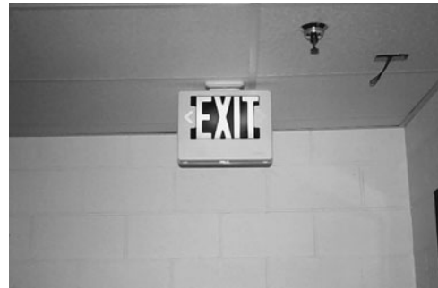
PHOTO 20.31 Exit lighting. (Used with permission of ABC)
