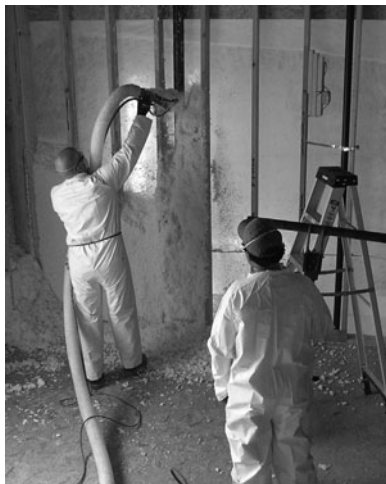
PHOTO 3.4 Loose-fill fiberglass insulation being sprayed into wall cavities. (Used with permission of ABC)
