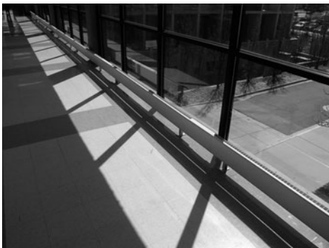
PHOTO 7.32 A convective radiator is placed along a curtain window wall to counter the downward convective drafts and radiant temperature effects. (Used with permission of ABC)
