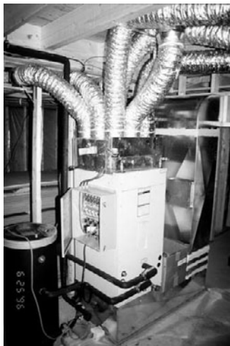
PHOTO 8.16 An individual supply duct system. (Courtesy of NREL/DOE)
