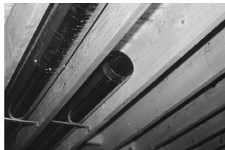
PHOTO 7.3 Unlined round ducts. (Used with permission of ABC)
