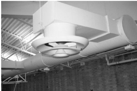
PHOTO 7.15 A large, round ceiling diffuser. (Used with permission of ABC)
