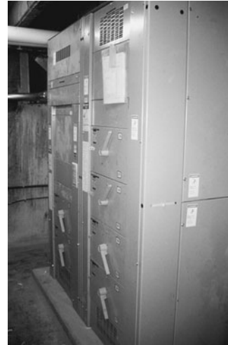
PHOTO 19.23 Switchboard for a manufacturing facility. (Used with permission of ABC)
