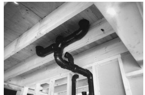
PHOTO 14.7 A drain stack passes through the wall above and picks up additional drain branches before transitioning to a short horizontal section and back to a vertical section to accommodate changes in wall alignment. The vent connecting to the horizontal section is under construction and not fully connected. (Used with permission of ABC)
