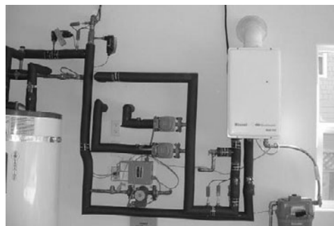
PHOTO 11.12 A solar domestic hot water system with a natural gas backup. This project is a demonstration project showing all components, except the flat-plate solar collectors mounted on the roof and associated piping. (Courtesy of DOE/NREL)
