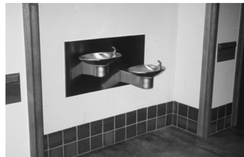
PHOTO 12.30 A wall-mounted drinking fountain unit. Chilled water is provided to the unit. (Used with permission of ABC)
