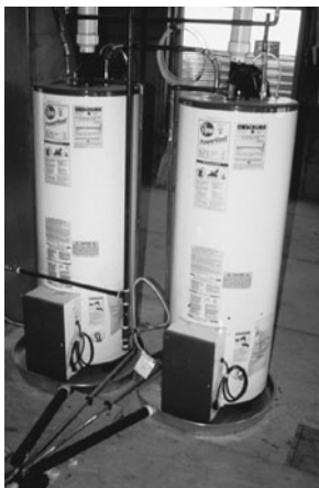
PHOTO 13.34 Two ultraefficient, gas-fired, power-vented, storage tank water heaters connected in series. Note the drain pans at the base of each unit that are designed to drain water into a floor drain. (Used with permission of ABC)
