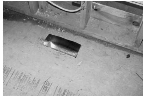
PHOTO 8.4 The register box fitting conveys heated air through the subfloor to the heated space. (Used with permission of ABC)
