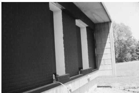
PHOTO 11.23 An unvented thermal storage wall under construction. The thermal storage wall is constructed of cast-in-place concrete and painted black to improve absorption of sunlight. Note the shadow line indicating shading of the wall. Photograph was taken at solar noon in early May. (Used with permission from ABC)
