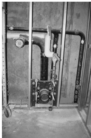
PHOTO 14.6 A flange and bracket connection to hold a wall-mounted water closet and connect it to a fixture branch. (Used with permission of ABC)
