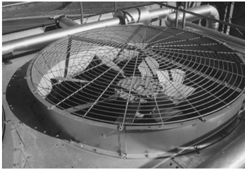
PHOTO 6.30 A fan draws outdoor air through the wet fill on the sides of the cooling tower to increase evaporation and cooling. Air is discharged above the tower. (Used with permission of ABC)
