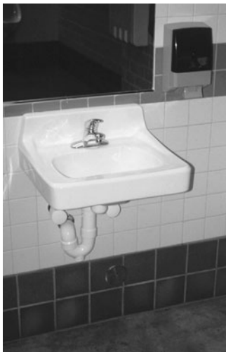
PHOTO 12.24 A cast, vitrified china wall-mounted lavatory in a public restroom. (Used with permission of ABC)
