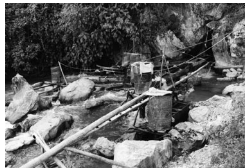
PHOTO 25.33 A crude pico hydropower system in Vietnam.
