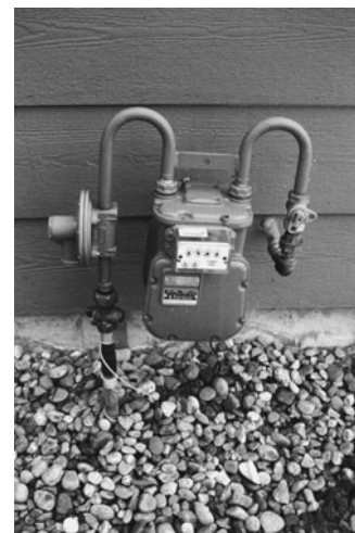
PHOTO 6.39 A natural gas meter. (Used with permission of ABC)
