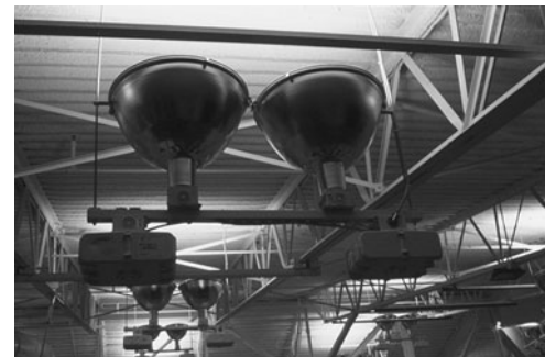
PHOTO 20.10 An HID uplight luminaire. (Used with permission of ABC)
