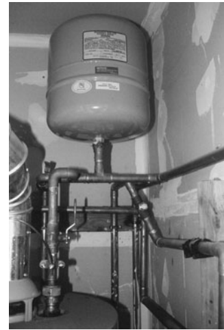
PHOTO 13.25 An expansion tank for potable water. (Used with permission of ABC)
