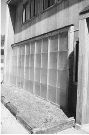
PHOTO 11.20 A close-up view of the thermal storage wall. (Used with permission from ABC)
