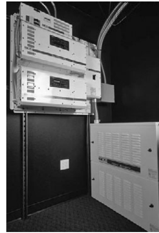
PHOTO 11.46 The PV solar system supplies power to inverters and battery storage that provide an uninterruptible power supply to the Zion Visitors Center. PV technology is covered in Chapter 25. (Courtesy of DOE/NREL)
