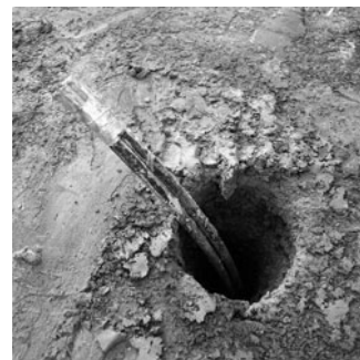
PHOTO 25.12 Vertical loops are installed and backfilled with coarse sand to a level of 30 ft (10 m), and then a 20% solid bentonite grout is pumped down to fill the remainder of the hole. (Courtesy of DOE/NREL)
