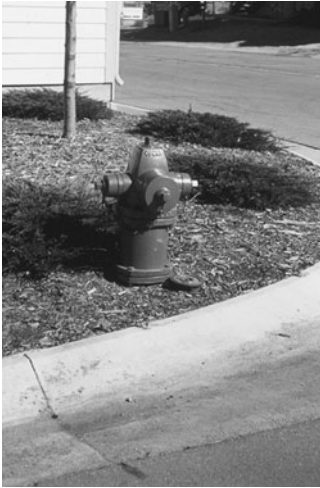
PHOTO 21.16 A fire hydrant for fire department hookup. (Used with permission of ABC)
