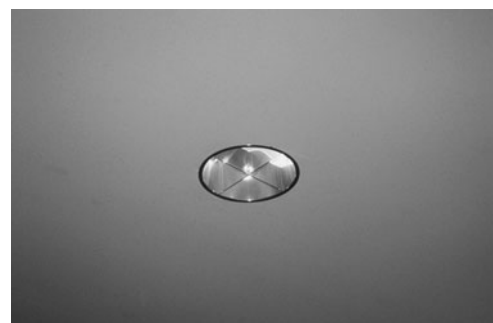
PHOTO 20.23 Louvers on this recessed compact fluorescent luminaire reduces glare. (Used with permission of ABC)
