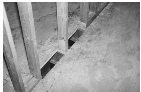
PHOTO 8.13 The opening in the subfloor through which return air flows. Note that the floor decking has been removed. (Used with permission of ABC)
