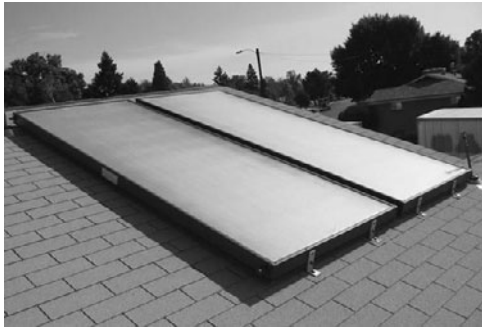
PHOTO 11.3 Two roof-mounted flat-plate collectors for domestic water heating at this Habitat for Humanity house in Denver, Colorado. (Courtesy of DOE/NREL)
