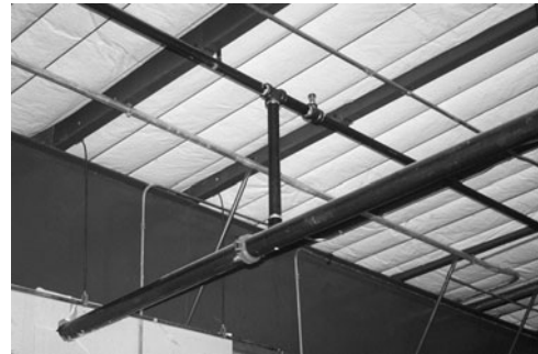
PHOTO 21.7 A cross main (large pipe) connected to a sprinkler branch. (Used with permission of ABC)
