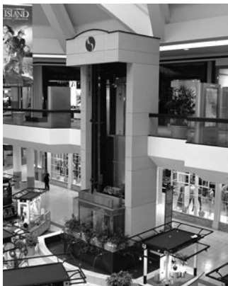
PHOTO 24.4 An open elevator hoistway serving two stories. (Used with permission of ABC)
