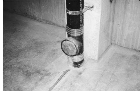
PHOTO 16.4 A cleanout is typically provided at the base of a vertical conductor. (Used with permission of ABC)
