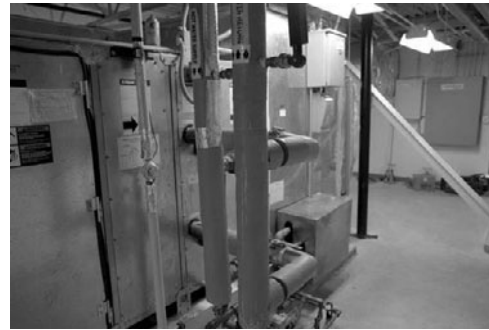
PHOTO 6.34 A commercial-scale direct evaporative cooler built into an air-handling unit and partially hidden from view by the hot water and hot water return lines (vertical pipes). The evaporative cooler is fed by a single pipe off of the hot water supply line (left pipe). (Used with permission of ABC)
