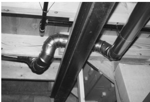
PHOTO 8.9 Ductwork must pass around obstacles. The design shown in this photograph is not effective because it has significant pressure loss. (Used with permission of ABC)
