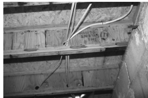
PHOTO 19.14 Circuit cables can pass through floor and ceiling joists. (Used with permission of ABC)
