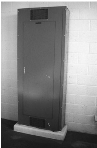
PHOTO 19.30 A 480 Y/277 V–400 A, three-phase panelboard providing three-phase power to equipment (e.g., milling machines, lathes, machining centers, and so on) or 277 V single-phase power for lighting. (Used with permission of ABC)
