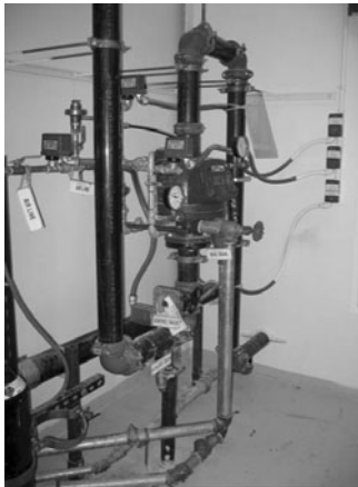
PHOTO 21.5 Wet-pipe sprinkler control with pressurized water in the pipe and mains. (Used with permission of ABC)
