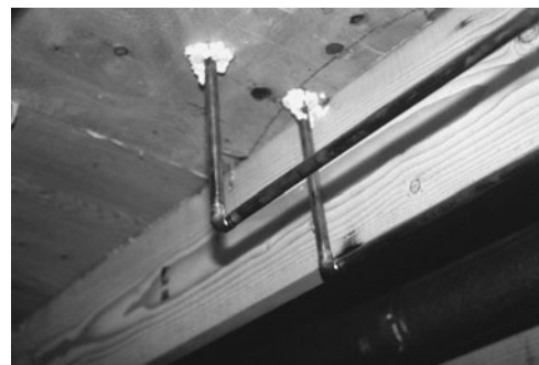
PHOTO 23.3 Sealed openings to prevent flanking of sound from a bathroom above. (Used with permission of ABC)
