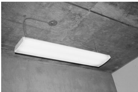
PHOTO 20.20 A linear fluorescent luminaire with prismatic wraparound lens that diffuses light. (Used with permission of ABC)
