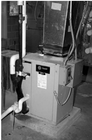
PHOTO 25.3 A 1.4 ton geothermal heat pump unit, part of the geothermal heat pump system. (Courtesy of DOE/NREL)
