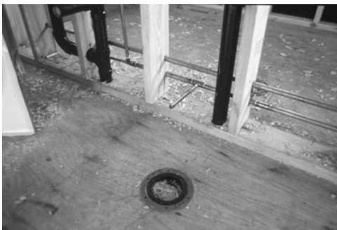
PHOTO 14.5 A floor-mounted water closet flange. (Used with permission of ABC)
