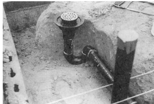
PHOTO 16.14 A below-slab floor drain. (Used with permission of ABC)
