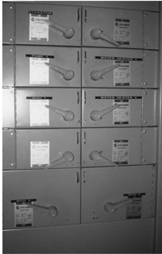
PHOTO 19.26 Distribution panels with fused disconnects. (Used with permission of ABC)
