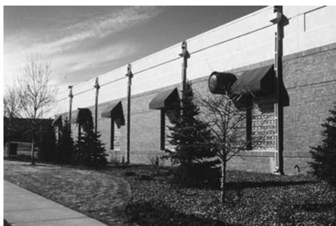
PHOTO 16.7 A series of exterior roof drains. (Used with permission of ABC)
