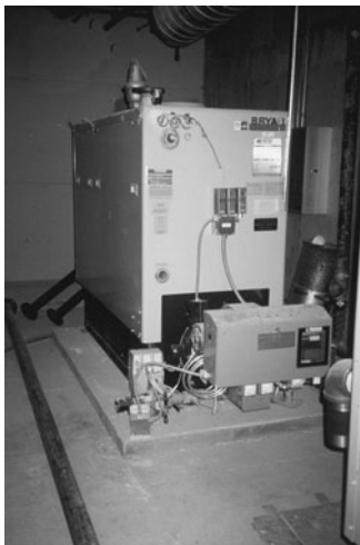
PHOTO 9.1 A commercial hot water boiler. (Used with permission of ABC)
