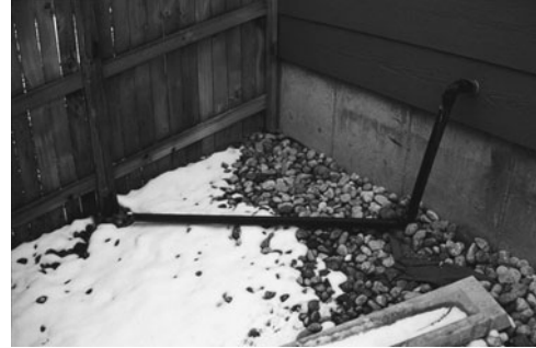
PHOTO 16.12 An exterior sump discharge line. (Used with permission of ABC)
