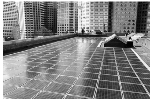
PHOTO 25.17 A PV system integrated into a horizontal roof consisting of 372 panels at the Williams Building in downtown Boston, Massachusetts. (Courtesy of DOE/NREL)
