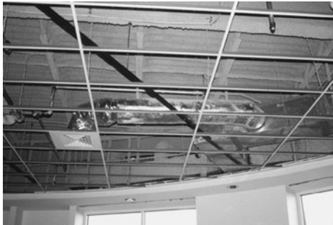
PHOTO 7.14 A ceiling diffuser connected to a flexible branch duct, which is tapped in to a main duct. Use of a flexible duct makes for easier placement of the diffuser once the suspended ceiling grid is installed. (Used with permission of ABC)
