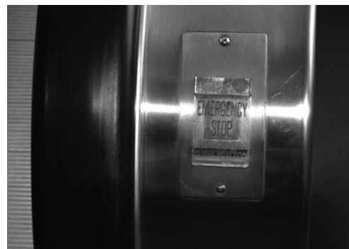
PHOTO 24.11 An emergency stop switch on an escalator. (Used with permission of ABC)
