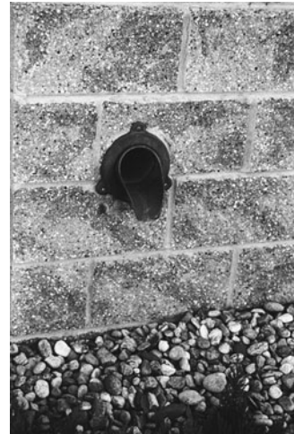
PHOTO 16.5 The discharge of storm water at the building exterior. (Used with permission of ABC)
