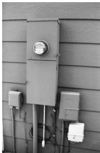
PHOTO 19.6 A 120/240 V-150 A, underground service entrance for a single-family residence. (Used with permission of ABC)
