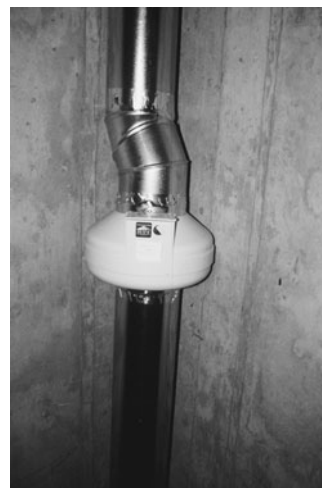
PHOTO 3.20 An inline blower draws soil gasses, including radon, and exhausts them to the outdoors before they enter the living space of the home. (Used with permission of ABC)
