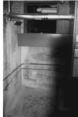
PHOTO 19.24 Service entrance conductors and feeder conductors encased in conduit and a wire gutter. Note the grounding wire (bottom wire). (Used with permission of ABC)
