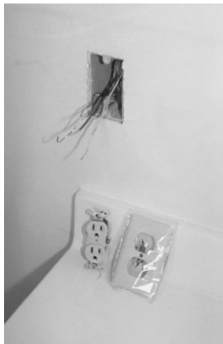
PHOTO 19.20 Exposed box in finished drywall with unattached receptacle and faceplate. (Used with permission of ABC)
