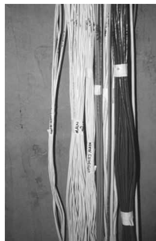
PHOTO 22.21 Home telecommunication wiring. (Used with permission of ABC)
