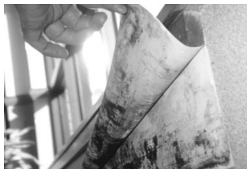
PHOTO 3.16 Evidence of mold growth under wallpaper; the cause was leakage in the return ducts. (Courtesy of DOE/NREL)
