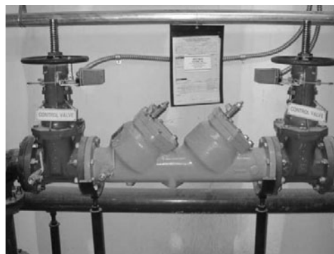
PHOTO 13.23 A double check assembly (DCA) is a backflow prevention device that consists of two check valves assembled in series usually with a ball valve or gate valve installed at each end for isolation and testing. The DCA shown is for the water supply to a fire sprinkler system. (Used with permission of ABC)
