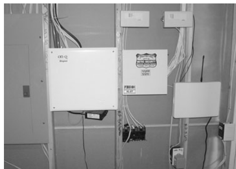
PHOTO 22.20 An advanced home wiring system service center with security and wireless capabilities. (Used with permission of ABC)
