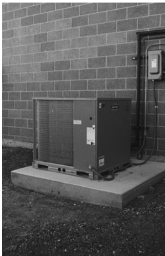
PHOTO 6.17 An air-cooled condensing unit on a split system. (Used with permission of ABC)
