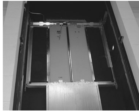
PHOTO 24.5 Hoistway doors as viewed from inside of hoistway. Guide rails are evident on the left and right side of the hoistway walls. (Used with permission of ABC)
