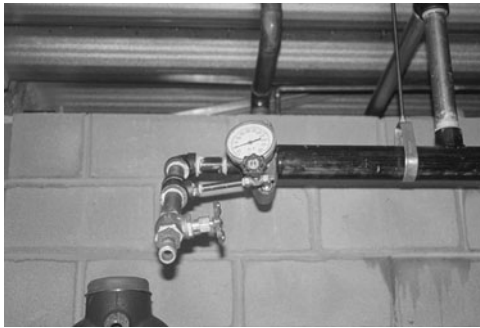
PHOTO 21.19 A pressure test of a sprinkler system. (Used with permission of ABC)
