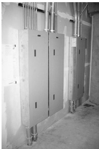
PHOTO 18.3 Power distribution and lighting panelboards serving one floor of a commercial office building. (Used with permission of ABC)
