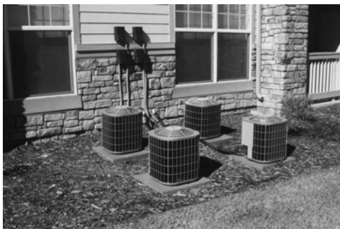
PHOTO 6.18 Four small air-cooled condensing units as part of an individual split system for four condominiums. (Used with permission of ABC)
