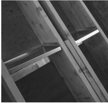
PHOTO 8.14 Sheet metal creates a return air duct between floor joist spacing. (Used with permission of ABC)
