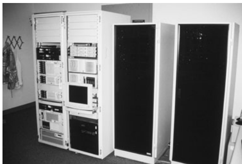
PHOTO 22.4 Telecommunications room and equipment, including server, router and switches. (Used with permission of ABC)
