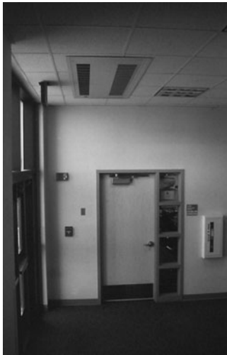
PHOTO 7.39 A flush-mounted ceiling fan-coil unit. (Used with permission of ABC)
