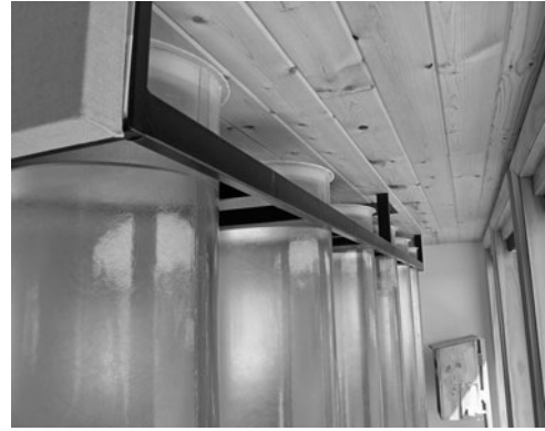
PHOTO 11.31 Fiberglass tubes are capped at top and secured at ceiling to prevent tipping. (Used with permission from ABC)
