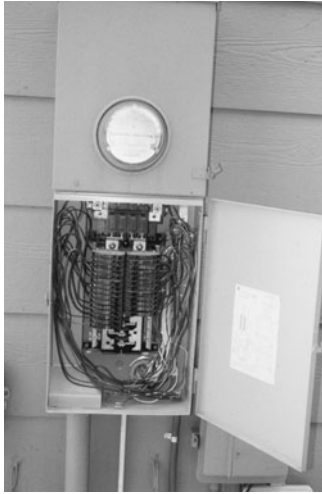
PHOTO 19.8 Panelboard with face removed. (Used with permission of ABC)
