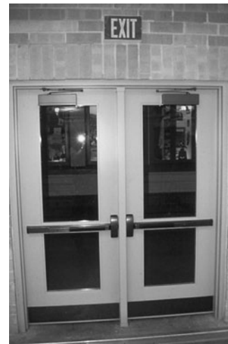
PHOTO 21.2 Exit signage for occupant egress. (Used with permission of ABC)
