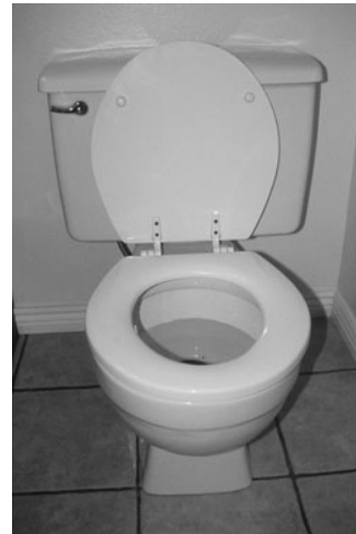
PHOTO 12.10 A flush tank water closet. (Used with permission of ABC)
