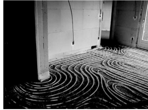
PHOTO 9.9 A radiant floor system. (Courtesy of DOE/NREL)
