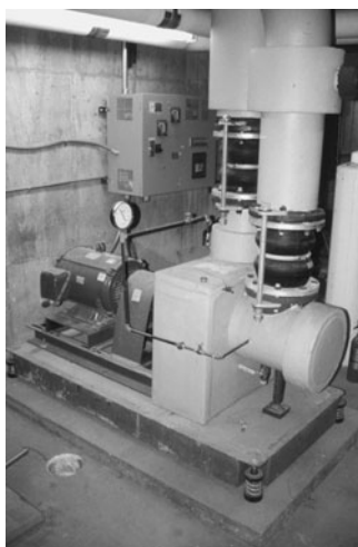
PHOTO 6.32 Pumps used to pump chilled water to several air-handling units located in different zones in the building. (Used with permission of ABC)
