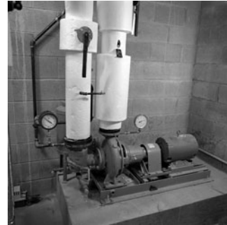
PHOTO 25.10 A commercial scale pump that circulates water from a geothermal heat pump to the ground source heat exchangers. (Courtesy of DOE/NREL)
