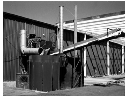
PHOTO 25.15 Biomass heat exchanger furnace can burn corn husks, wood residue, or other biomass fuels to produce warm air for space heating. (Courtesy of DOE/NREL)
