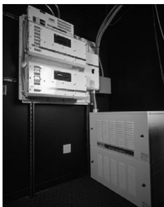
PHOTO 25.26 The PV solar system supplies power to inverters and battery storage that provide an uninterruptible power supply to the Zion Visitors Center. (Courtesy of DOE/NREL)
