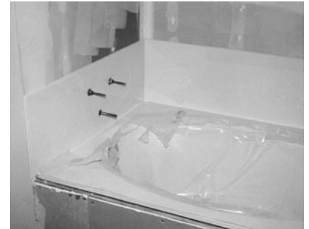
PHOTO 13.11 A rough-in of fixture branches for a bathtub (no showerhead). (Used with permission of ABC)
