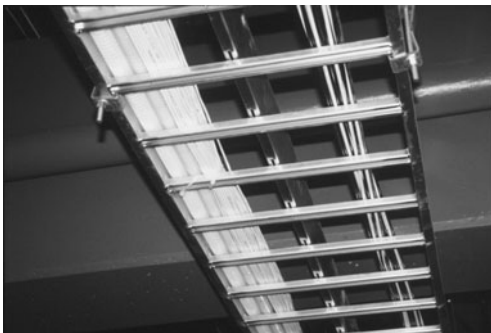
PHOTO 22.10 Horizontal backbone cabling in a wire tray. (Used with permission of ABC)
