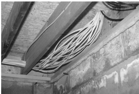
PHOTO 19.13 Branch circuit conductors are fed to outlets. (Used with permission of ABC)
