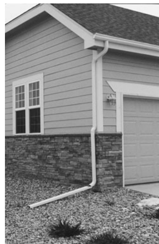
PHOTO 16.8 A residential roof drainage system consists of an ogee-shaped gutter to capture roof water (at roof overhand), a downspout (running vertically), and a downspout extension (at ground level), which is designed to discharge storm water well away from the building. (Used with permission of ABC)
