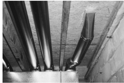
PHOTO 8.2 Branch ducts extend off the main duct to convey air to the heated spaces. (Used with permission of ABC)
