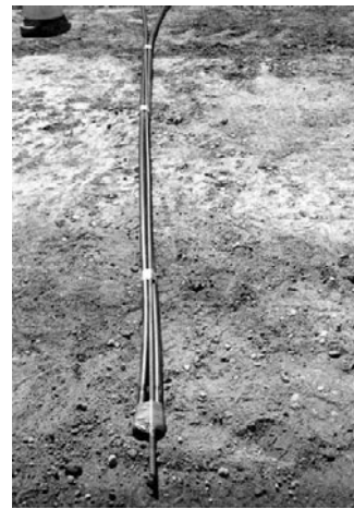
PHOTO 25.11 A 200 ft (61 m) loop being pressure tested. Note the 10-ft piece of rebar that is duct taped to the bottom of the loop. This rebar will help keep the loop straight as it is inserted into the hole. It also adds weight to help keep the loop in the hole. (Courtesy of DOE/NREL)
