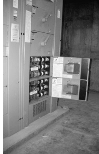
PHOTO 19.27 Open distribution panels exposing two sets of fuses. (Used with permission of ABC)
