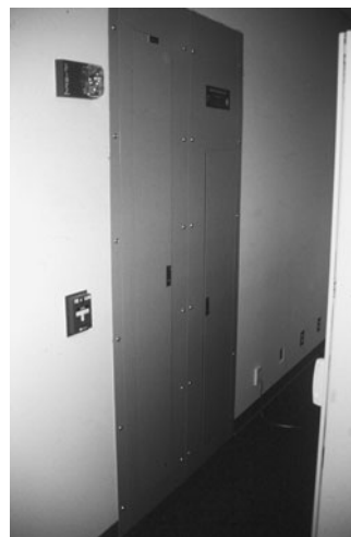
PHOTO 22.5 Electrical panelboard providing filtered “clean” power to telecommunications room equipment. Battery-backup provides an interruptible power supply. Note the fire alarm and manual pull station nearby. (Used with permission of ABC)
