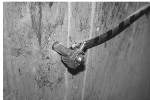
PHOTO 19.25 Ground wire connection to grounding rod that extends into earth on other side of foundation wall. (Used with permission of ABC)
