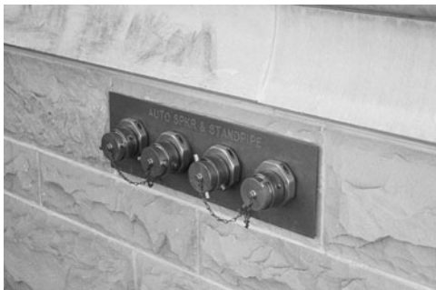
PHOTO 21.18 Automatic sprinkler system and standpipe connections for fire department hookup. (Used with permission of ABC)
