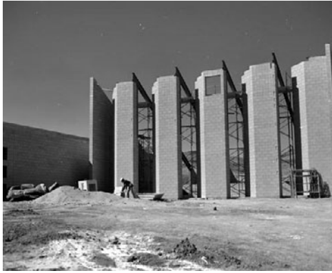
PHOTO 11.28 Construction of the fully grouted, reinforced concrete masonry articulated thermal storage wall at the NREL Visitor Center, Golden, Colorado. (Courtesy of DOE/NREL)
