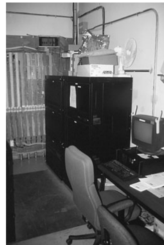
PHOTO 22.3 Local exchange carrier (LEC) and private branch exchange (PBX) building entrance. (Used with permission of ABC)
