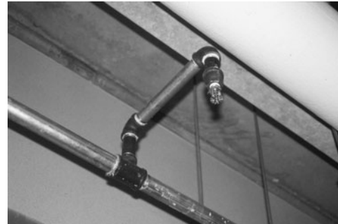
PHOTO 21.11 A sprinkler head connected to a branch before being covered with a suspended ceiling. (Used with permission of ABC)
