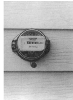
PHOTO 13.4 A wall-mounted exterior water meter. (Used with permission of ABC)
