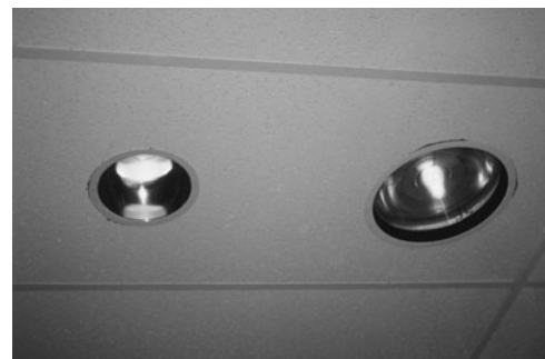
PHOTO 20.24 A blended lighting installation can be used to provide efficient ambient lighting with good color rendition. An incandescent luminaire (right) offers good color rendering characteristics and an HID luminaire (left) provides highly efficient lighting, which also serve to accent the space. (Used with permission of ABC)
