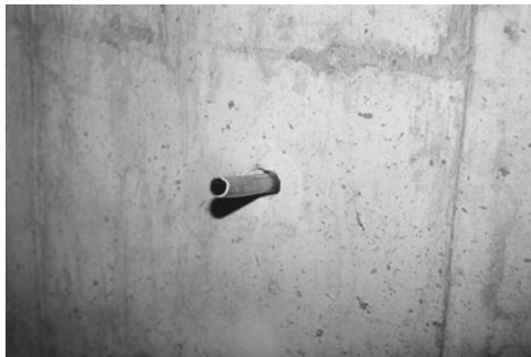
PHOTO 13.1 Rough-in of a residential service line passing through a foundation wall. (Used with permission of ABC)
