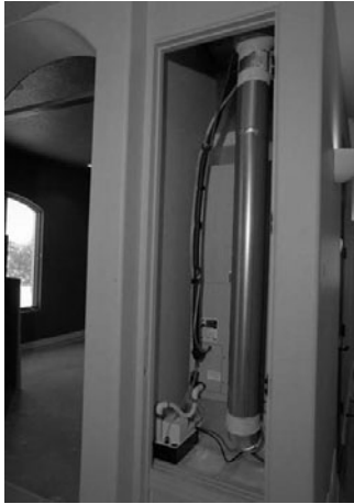
PHOTO 7.46 A small-scale (residential), supply-only air handler for outside air ventilation. (Courtesy of NREL/DOE)
