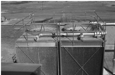
PHOTO 6.27 A side view of a cooling tower. (Used with permission of ABC)
