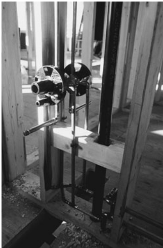
PHOTO 13.9 A front side view of branches connecting to a bathtub and showerhead control valve. (Used with permission of ABC)
