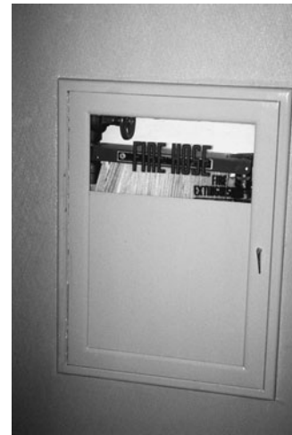
PHOTO 21.3 A properly marked fire hose cabinet (closed). (Used with permission of ABC)
