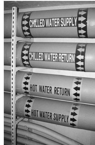
PHOTO 6.33 Labeled chilled water (from chiller) and hot water (from boiler) pipes on their way to and from several air-handling units located in different zones in the building. (Used with permission of ABC)
