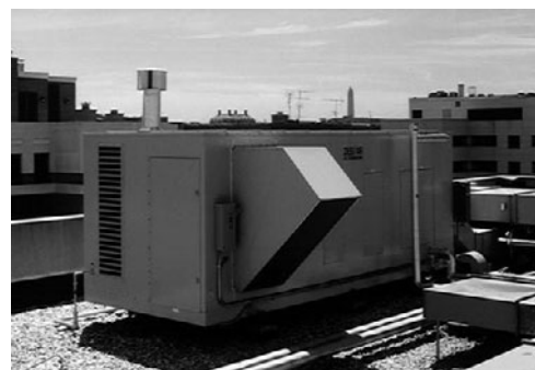
PHOTO 6.38 A rooftop desiccant unit designed to handle the make-up air requirements. (Courtesy of NREL/DOE)
