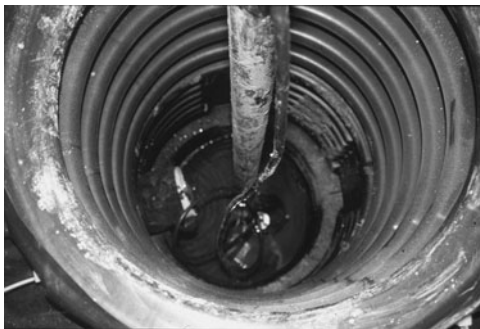
PHOTO 16.11 A view into the sump in the previous photograph. A sump pump is situated in the bottom of the sump. (Used with permission of ABC)
