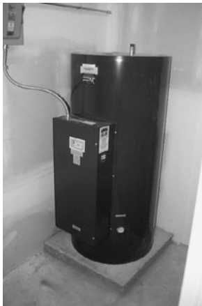
PHOTO 13.33 A commercial, electric storage tank water heater. Note the presence of an electrical connection and lack of presence of a vent. (Used with permission of ABC)
