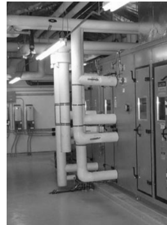
PHOTO 7.25 A close-up view of chilled water and hot water supply and return pipes connected to the air-handling unit (AHU) in the previous photograph. (Used with permission of ABC)
