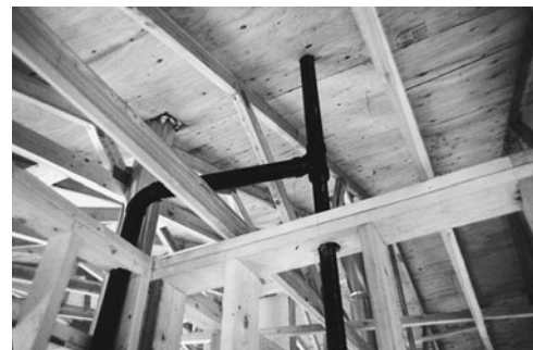
PHOTO 14.13 A vent connection and penetration through the roof decking. (Used with permission of ABC)
