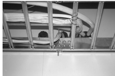
PHOTO 22.12 Horizontal backbone cabling entering a firewall. The openings are sealed with an approved firestopping material. (Used with permission of ABC)
