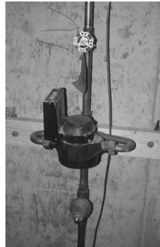
PHOTO 13.3 A residential service line with an interior water meter, shut-off valve (above meter), and pressure-reducing valve (below meter). (Used with permission of ABC)
