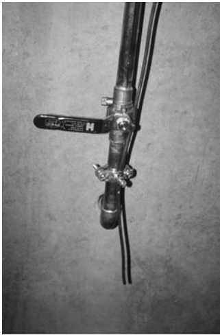
PHOTO 19.10 A main ground extends from the panelboard to the water service pipe and to a grounding rod (not shown). (Used with permission of ABC)
