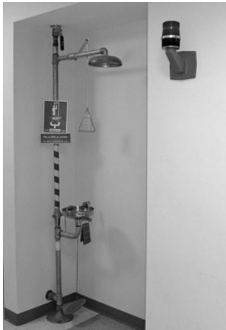
PHOTO 12.31 An emergency drench shower at a university laboratory. (Used with permission of ABC)
