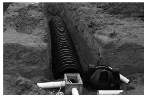
PHOTO 15.8 Gravel-less drain pipe during construction. Pipe will be covered with soil. (Used with permission of ABC)
