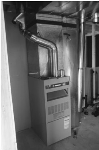
PHOTO 6.5 An upflow, warm-air furnace. The supply air plenum (above furnace) carries heated air to the rectangular main duct or trunk suspended from the ceiling. Return air recirculates back to the furnace in the rectangular return air duct also suspended from the ceiling (in foreground). Main ducts are isolated from the furnace with a flexible duct connection that allows movement and isolates furnace vibration. Round ducts on the side of furnace introduce air for combustion. (Used with permission of ABC)
