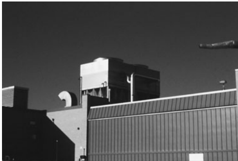
PHOTO 6.26 A roof-mounted cooling tower. (Used with permission of ABC)
