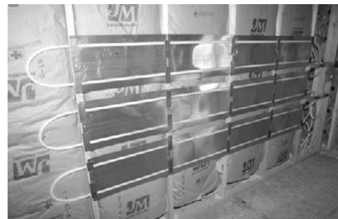
PHOTO 9.10 In-wall radiant panels. (Courtesy of DOE/NREL)
