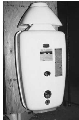
PHOTO 13.35 A gas-fired instantaneous water heater. (Used with permission of ABC)
