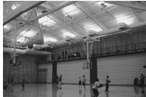
PHOTO 20.3 Ambient lighting is used to provide uniform illumination. In this case, HID upright luminaires are used to provide lighting in a gymnasium. (Used with permission of ABC)
