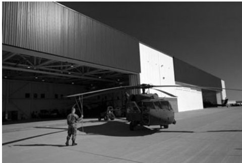
PHOTO 11.13 7800 ft 2 (725 m 2 ) of transpired solar collector area (the upper dark wall) used as a ventilation air preheating system on a helicopter maintenance hangar at Fort Carson U.S. Army Base, south of Colorado Springs, Colorado. (Courtesy of DOE/NREL)
