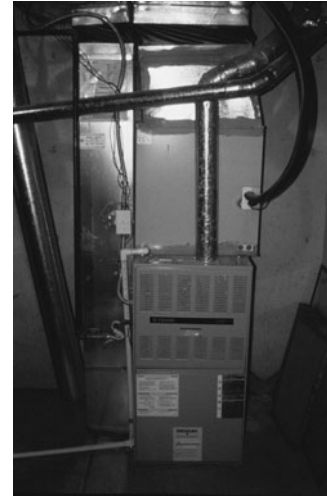
PHOTO 8.17 A furnace serves as an air-handling unit in many split-system air conditioning installations. In this installation, the absorption (cooling) coil is mounted in a plenum above the furnace. Refrigeration lines extend out of the furnace plenum (just above and to the right of the furnace) and are connected to the condensing unit located outdoors. (Used with permission of ABC)
