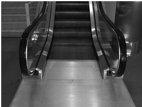
PHOTO 24.9 A lower landing of an escalator. Note how the stairs raise at the beginning of the escalator. An emergency stop switch extends from the right handrail. (Used with permission of ABC)
