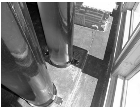
PHOTO 11.30 Fiberglass tubes are anchored to the concrete floor. (Used with permission from ABC)
