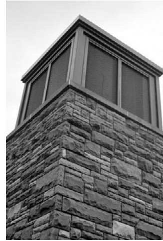
PHOTO 11.42 A close-up photograph of the PDEC tower of the Zion Visitor Center. (Courtesy of DOE/NREL)
