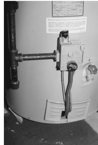
PHOTO 13.29 A gas connection to a residential storage tank water heater. Note the drain valve on the right side of the tank. (Used with permission of ABC)
