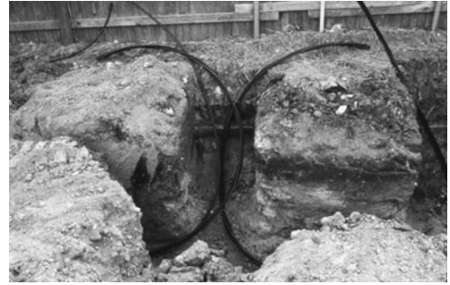
PHOTO 19.2 Underground distribution lines readied for connection to exterior transformer. (Used with permission of ABC)
