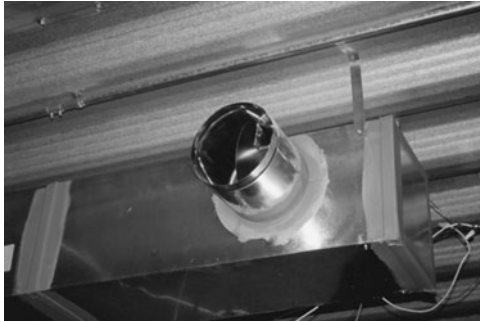
PHOTO 7.11 A butterfly damper in a round tap-in connection. Note use of duct mastic sealant. (Used with permission of ABC)
