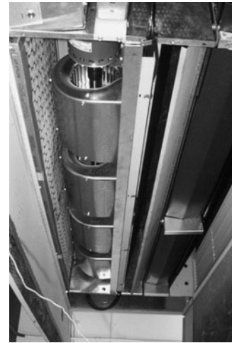
PHOTO 7.36 A close-up, inside view of a fan-coil unit. Evident are part of the filters (left side), four fans, and the drip pan below the cooling coil. (Used with permission of ABC)
