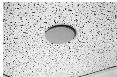
PHOTO 21.12 A covered sprinkler head in a finished suspended ceiling. The cover is used to conceal the sprinkler. It should not be painted. (Used with permission of ABC)
