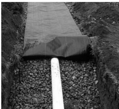
PHOTO 15.7 An absorption drainage trench. Trench will be covered with soil. (Used with permission of ABC)
