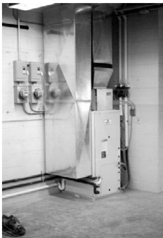
PHOTO 25.4 A residential-scale 3-ton geothermal heat pump unit, part of the geothermal system. (Courtesy of DOE/NREL)
