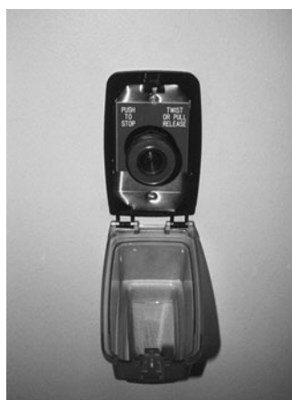
PHOTO 18.16 Emergency safety cut-off switch. Used to shut down equipment in an emergency (e.g., personal accident, fire, and so on). (Used with permission of ABC)
