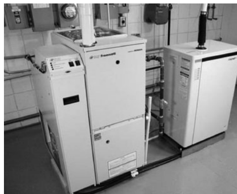
PHOTO 25.1 A residential-scale micro cogeneration (home heating and power) system that can produce about 1.2 kW of electric power and over 11 000 Btu/hr (3.26 kW) of heat. (Courtesy of DOE/NREL)
