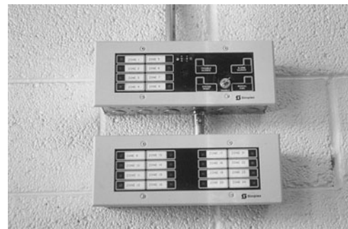
PHOTO 21.27 A fire status panel. (Used with permission of ABC)
