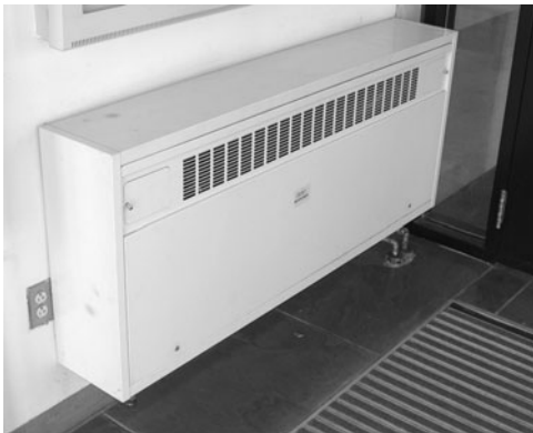
PHOTO 9.8 A cabinet heater. (Used with permission of ABC)
