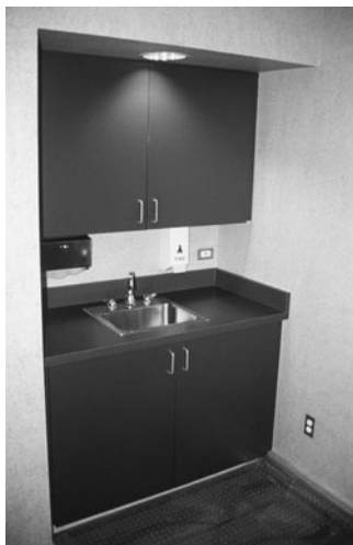
PHOTO 12.28 A stainless steel service sink. (Used with permission of ABC)
