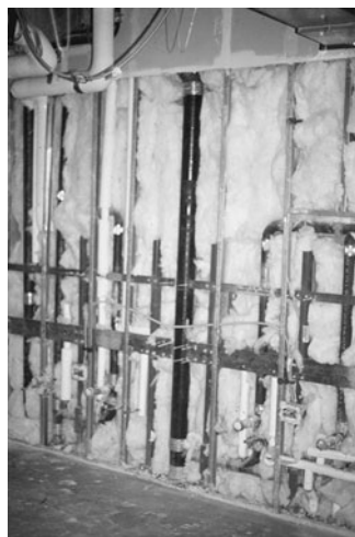
PHOTO 23.1 Acoustical insulation in a plumbing wall. (Used with permission of ABC)
