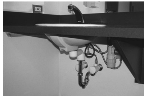
PHOTO 14.2 A P-trap under a bathroom lavatory. (Used with permission of ABC)
