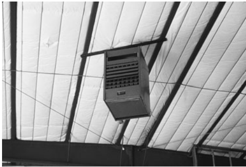
PHOTO 6.13 A gas-fired unit heater suspended from a warehouse ceiling before natural gas piping and venting are installed. (Used with permission of ABC)
