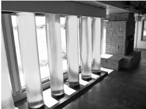
PHOTO 11.29 A water wall and stone fireplace used as a thermal storage wall in a classroom in a nature center facility. Fiberglass tubes contain about 75 gal/285 L (~625 lb/280 kg) of light blue-colored water. Floors are colored concrete, which also serve as thermal mass. (Used with permission from ABC)
