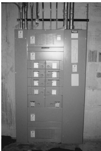
PHOTO 18.2 A switchboard divides large amounts of current into smaller amounts used by individual pieces of electrical equipment (e.g., air-handling units, pump motors, and so on) or panelboards. (Used with permission of ABC)
