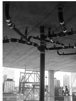
PHOTO 14.18 A drain stack interval in a high-rise condominium building. (Used with permission of ABC)
