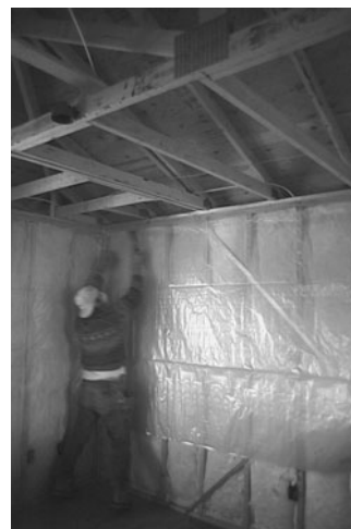
PHOTO 3.22 Installation of a polyethylene VDR on the “warm” side of a framed wall in a building in a heating climate. (Used with permission of ABC)
