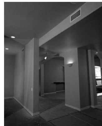
PHOTO 7.19 High wall registers used for cooling in a residential installation. (Courtesy of NREL/DOE)
