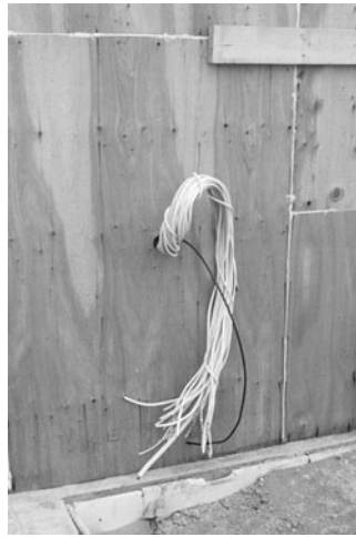
PHOTO 19.11 Branch circuit cables shown before installation of the panelboard. (Used with permission of ABC)
