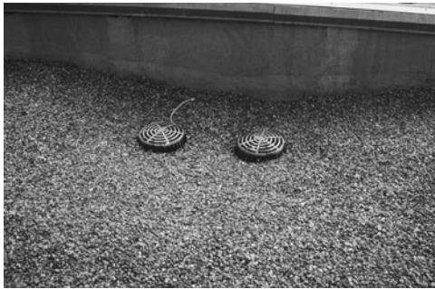
PHOTO 16.2 Interior roof drains on a low-sloped commercial roof system. (Used with permission of ABC)
