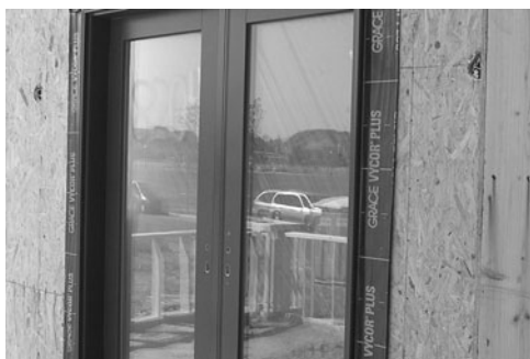
PHOTO 3.14 Self-adhered flashing installed to reduce air and moisture infiltration around window and door. (Used with permission of ABC)
