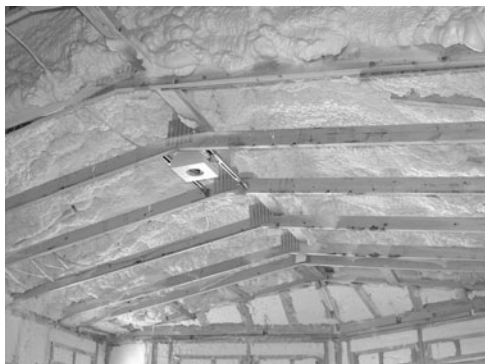
PHOTO 3.9 Icynene® spray foam insulation and air-sealing system installed in ceiling and wall cavities. (Used with permission of ABC)
