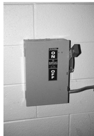
PHOTO 18.12 Heavy-duty switch. (Used with permission of ABC)
