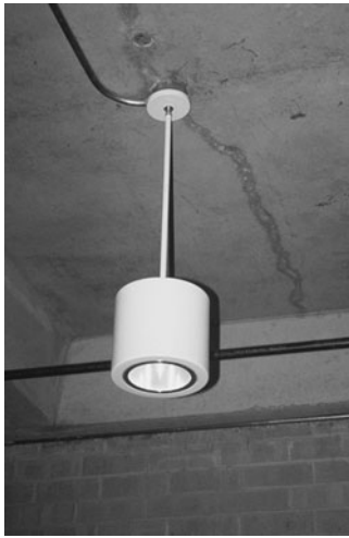
PHOTO 20.14 A pendent-type, recessed, compact fluorescent luminaire. (Used with permission of ABC)
