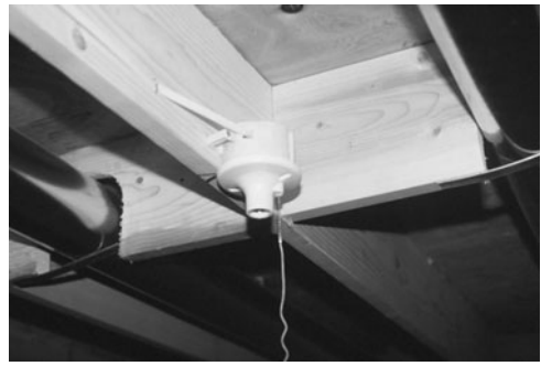
PHOTO 19.18 Exposed lighting fixture. (Used with permission of ABC)
