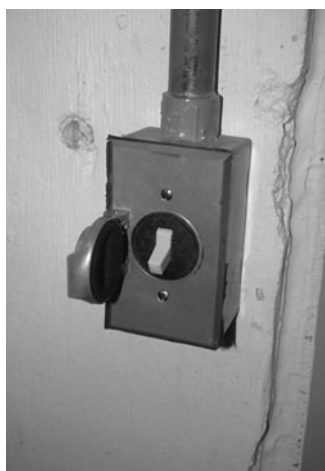
PHOTO 18.13 Weatherproof switch. (Used with permission of ABC)
