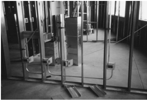
PHOTO 18.21 Four electrical boxes connected to metal conduit in a steel-framed partition. (Used with permission of ABC)
