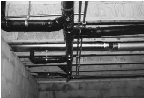
PHOTO 14.8 Horizontal branches connecting to a horizontal line. (Used with permission of ABC)
