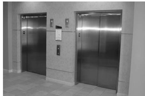
PHOTO 24.1 First-floor entrances to two elevator cars (doors closed). Note the hall lanterns between the doors (above sign). The hall station is below the sign.
