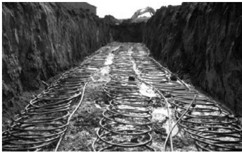
PHOTO 25.8 Placement of a Slinky® loop as part of a horizontal ground closed-loop system. (Courtesy of DOE/NREL)
