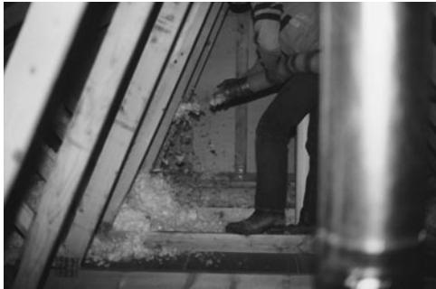
PHOTO 3.3 Loose-fill fiberglass being blown into an attic space. (Used with permission of ABC)
