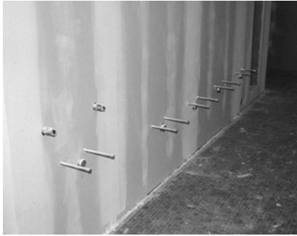
PHOTO 13.15 A rough-in of fixture branches for a group of lavatories in a public restroom. (Used with permission of ABC)
