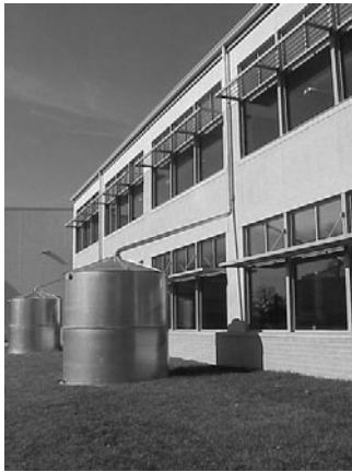
PHOTO 25.34 Rainwater harvesting cisterns. (Courtesy of DOE/NREL)
