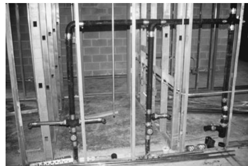
PHOTO 14.4 An unfinished plumbing wall with cast iron drain and vent lines. Copper fixture branches extend from the drain pipes and will be connected to trap arms that will extend from the wall. (Used with permission of ABC)
