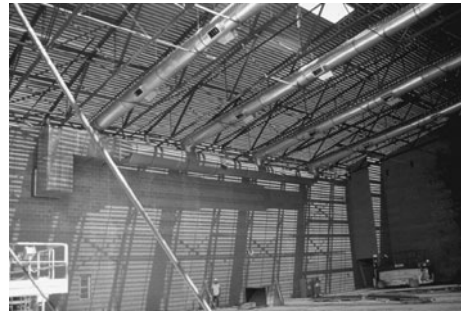
PHOTO 7.1 Ducts suspended from the ceiling of a gymnasium under construction. An air-handling unit (AHU) (not shown) behind the masonry wall blows conditioned air into the rectangular main duct (left side). Air then branches off into round branch ducts, where it is eventually introduced to the space through diffusers attached to the branch ducts. (Used with permission of ABC)
