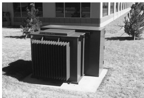
PHOTO 18.5 A pad-mounted building transformer serving a commercial office building. (Used with permission of ABC)
