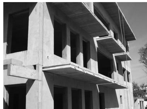
PHOTO 11.37 A view of a commercial building under construction with overhangs over windows that provide summer shading. (Courtesy of DOE/NREL)
