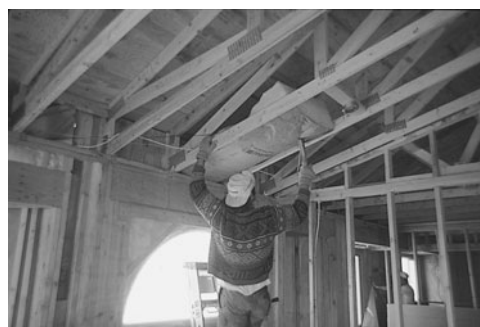
PHOTO 3.23 Installation of a blanket of insulation. Attached to the bottom face of the blanket is a bitumen-impregnated kraft paper facing (installed by manufacturer) that will serve as a VDR. (Used with permission of ABC)
