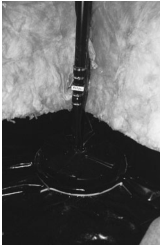
PHOTO 16.10 A sump in a crawl-space floor. (Used with permission of ABC)
