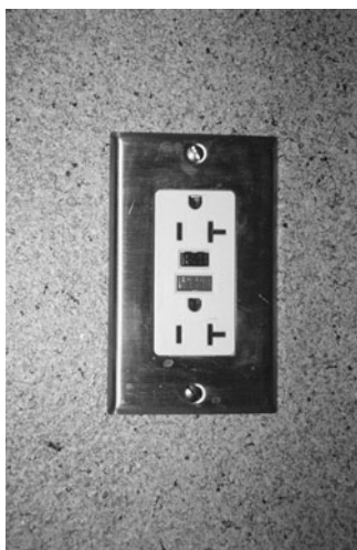
PHOTO 18.23 Receptacle outlet-type ground fault circuit interrupter. (Used with permission of ABC)
