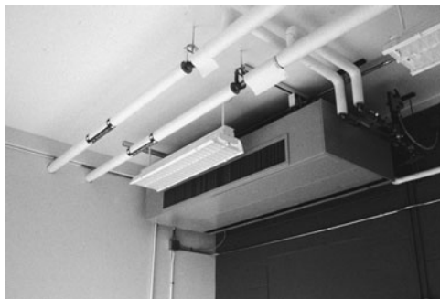
PHOTO 7.35 A ceiling-mounted fan-coil unit. (Used with permission of ABC)
