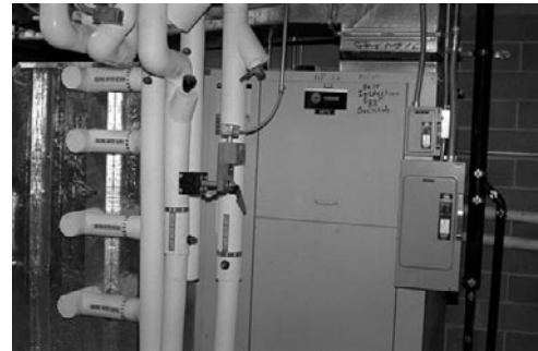
PHOTO 25.5 A medium-scale 16-ton geothermal heat pump unit serving Cavett Elementary School in Lincoln, Nebraska. (Courtesy of DOE/NREL)
