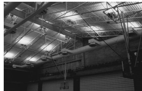
PHOTO 20.11 An HID uplight installation providing ambient lighting in a gymnasium. (Used with permission of ABC)
