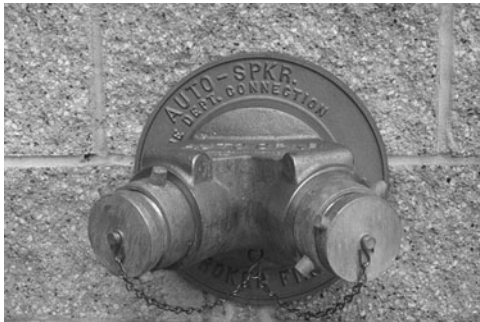
PHOTO 21.17 A Siamese connection for fire department hookup to automatic sprinkler system. These connections are a standard part of automatic sprinkler and standpipe systems. Firefighters connect a hose to the connection to introduce water to a standpipe or, in this case, a sprinkler system. (Used with permission of ABC)
