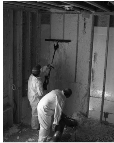
PHOTO 3.5 Loose-fill fiberglass insulation being scrapped to create a flat surface to accept gypsum wallboard finish. Excess insulation is vacuum collected for reuse. (Used with permission of ABC)
