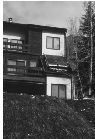
PHOTO 11.6 Two roof-mounted flat-plate collectors used in an active solar domestic water heating system. (Used with permission from ABC)
