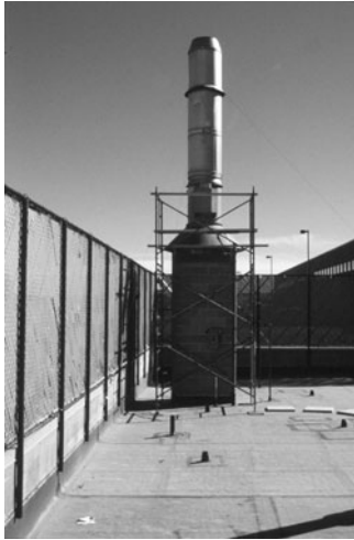
PHOTO 6.2 A close-up of the vent for the boilers in the next photograph. (Used with permission of ABC)
