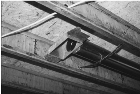
PHOTO 8.7 A branch duct can deliver heated air to a ceiling register. (Used with permission of ABC)
