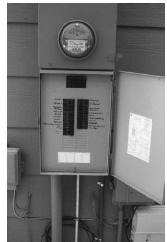
PHOTO 19.7 A service entrance with the electrical meter and main disconnect (below meter and above circuit breakers). Circuit breakers are properly marked on the panelboard face. (Used with permission of ABC)
