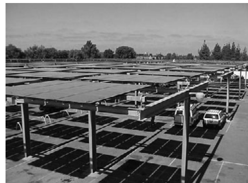
PHOTO 25.19 A 540-kW PV system provides shaded parking for about 1000 cars in a desert of scorching blacktop at the Cal Expo in Sacramento, California. (Courtesy of DOE/NREL)
