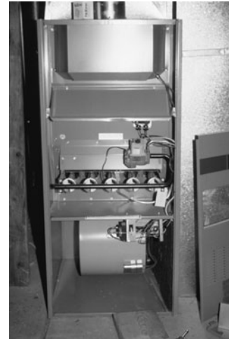
PHOTO 6.9 A standard, natural-draft, upflow warm-air furnace with access panels removed. The fan is evident in the lower blower compartment just below the inlets for five gas burners. The gas regulator is just above the burners. The regulator has not yet been connected to the natural gas line. (Used with permission of ABC)
