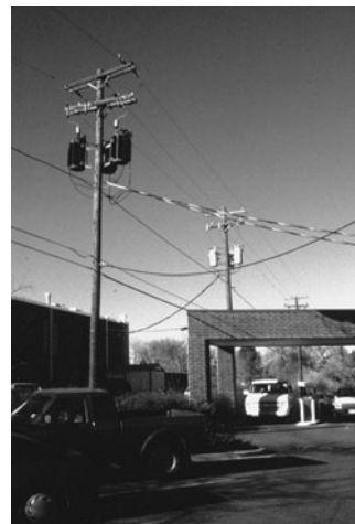
PHOTO 18.1 Overhead service entrance conductors extending from pole-mounted transformers. (Used with permission of ABC)
