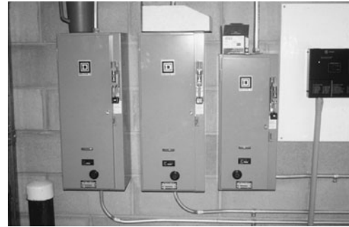
PHOTO 19.36 Circuits to equipment are controlled by heavy-duty switches. (Used with permission of ABC)
