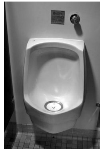
PHOTO 12.14 A waterless urinal, which represents the most water-efficient urinal option because they provide first-cost savings (e.g., eliminating the need to provide a water line and flush valve) and less maintenance (e.g., leaks, valve repairs, and water overflows) over the conventional urinals. (Courtesy of NREL/DOE)
