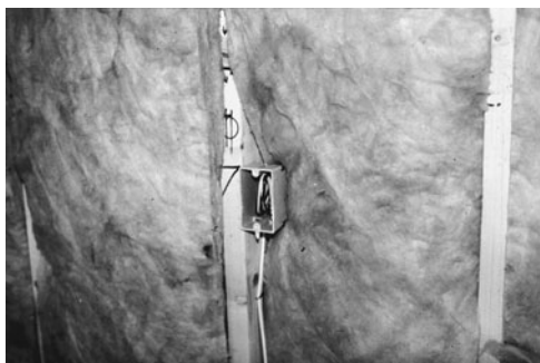
PHOTO 3.8 Care must be exercised in placement of blanket insulation. When it is compressed significantly, such as at electrical outlets, it loses its thermal effectiveness. (Used with permission of ABC)
