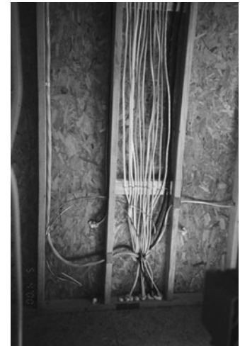
PHOTO 19.12 Branch circuit cables extend through the inside of the wall (behind the panelboard). (Used with permission of ABC)
