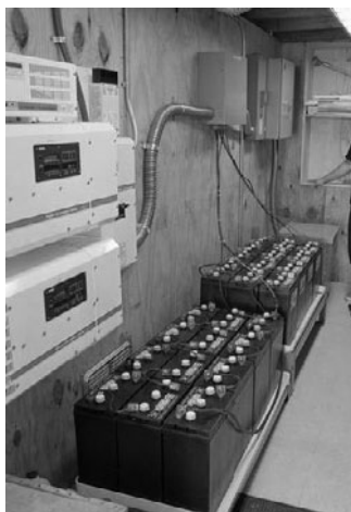
PHOTO 25.25 PV inverter (left) and battery storage at the Manzanita Indian Reservation near Boulevard, California. (Courtesy of DOE/NREL)
