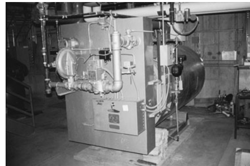
PHOTO 13.36 A water heating boiler that provides hot water to a commercial building. (Used with permission of ABC)
