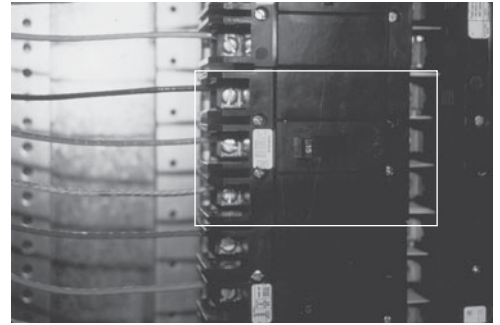
PHOTO 19.34 An individual three-phase breaker protects three conductors on a three-phase circuit. (Used with permission of ABC)
