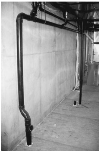
PHOTO 14.9 Horizontal branches connecting to a horizontal line, which then connects to a stack. A floor cleanout is located at the base of the stack. (Used with permission of ABC)
