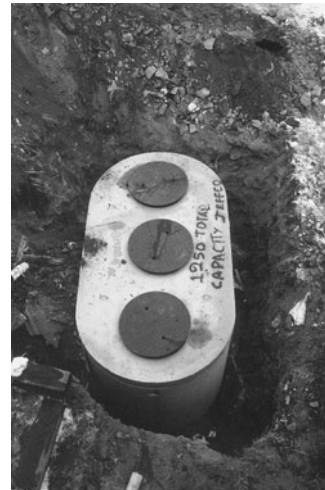
PHOTO 15.5 A 1250 gallon (4725 L) septic tank in hole before hole is backfilled. The three covers allow access to each compartment. Tank will be covered with soil. (Used with permission of ABC)
