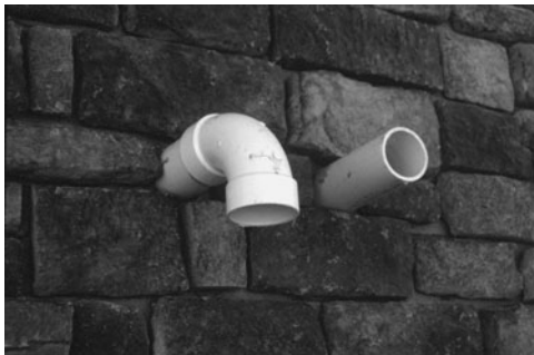
PHOTO 6.8 Sidewall, thermoplastic vents (under construction) to the two high-efficiency furnaces. (Used with permission of ABC)
