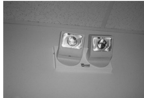
PHOTO 20.7 Emergency lighting installation. (Used with permission of ABC)
