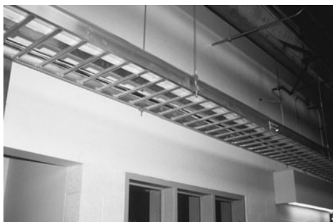
PHOTO 18.22 Conductors in an overhead wire tray. (Used with permission of ABC)
