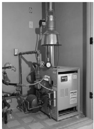
PHOTO 9.2 A residential hot water boiler. (Courtesy of DOE/NREL)
