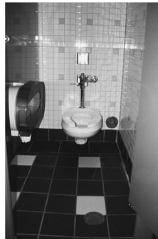
PHOTO 12.11 A wall-mounted, flush valve water closet. Note the wall cleanout cover at the floor line to the right of the water closet. (Used with permission of ABC)
