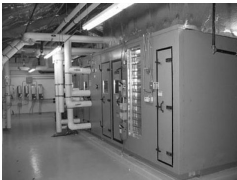
PHOTO 7.24 A medium-sized air-handling unit (AHU) in a mechanical room. This unit contains fans (blowers), a bank of filters, and heating and cooling coils. (Used with permission of ABC)
