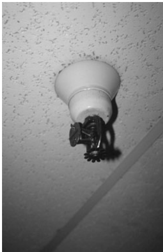
PHOTO 21.15 A fusible link pendent sprinkler head exposed in a finished ceiling. In this design, the water is prevented from leaving the sprinkler head by an arrangement of levers and links. The levers and links are soldered together on the sprinkler head. The solder is a metal alloy with a fixed melting point. (Used with permission of ABC)
