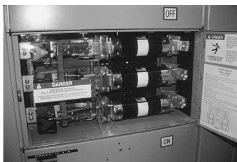
PHOTO 18.9 Three cartridge fuses installed to protect a three-phase circuit. (Used with permission of ABC)
