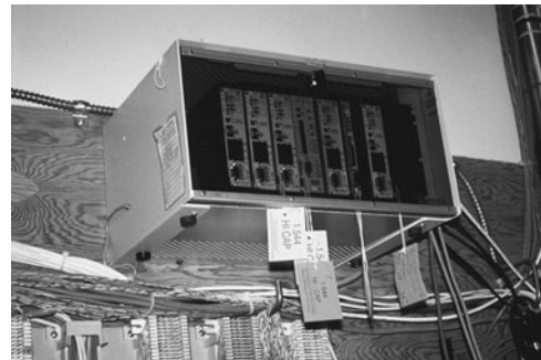
PHOTO 22.2 Internet service building entrance. (Used with permission of ABC)
