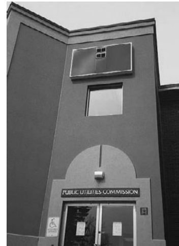
PHOTO 11.15 A thermosiphon air panel discharges air directly into the living space. (Courtesy of DOE/NREL)
