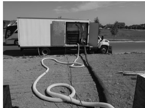
PHOTO 3.6 Loose-fill insulation is blown through a hose connected to a blower in a truck. Insulation is manually loaded into a hopper connected to the blower. This is one method of installing loose fill insulation. (Used with permission of ABC)
