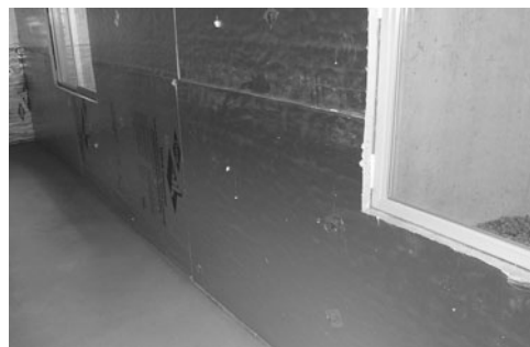
PHOTO 3.11 Foil-faced rigid foam insulation installed on basement foundation wall. (Used with permission of ABC)
