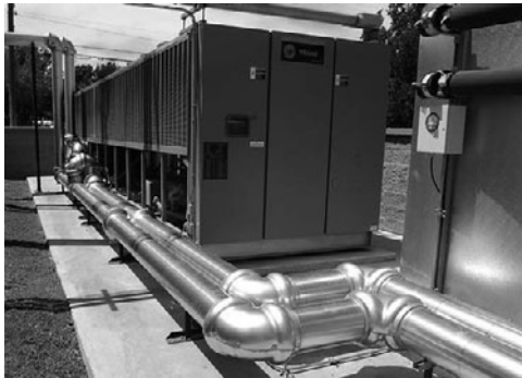
PHOTO 6.23 A rooftop central hot/chilled water plant that produces both hot water and chilled water (in lieu of a boiler and chiller). (Courtesy of NREL/DOE)
