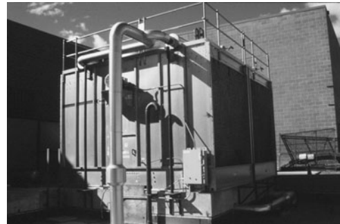
PHOTO 6.28 Condenser water is piped to the top of the cooling tower, where it is sprayed over the cooling tower fill. (Used with permission of ABC)
