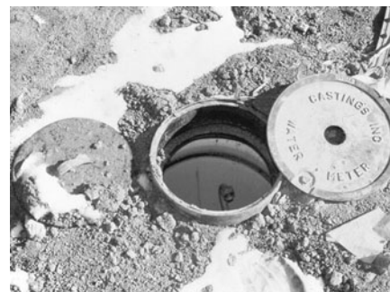
PHOTO 13.5 An underground curb box ready for water meter installation. (Used with permission of ABC)
