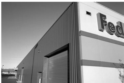
PHOTO 11.10 A transpired collector on the entire south (left) side of the Federal Express building in Englewood, Colorado. Solar energy absorbed by the wall provides heated ventilation air to the warehouse. (Courtesy of DOE/NREL)
