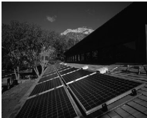
PHOTO 25.16 A 7.2 kW PV rooftop array at the Visitor Center at Zion National Park, Springdale, Utah, provides electricity. It provides about 12% of the Center's power needs. This Center was introduced at the end of Chapter 11. (Courtesy of DOE/NREL)
