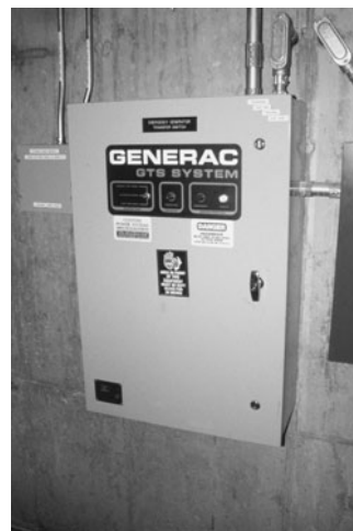
PHOTO 21.32 An automatic transfer switch for an emergency generator system. (Used with permission of ABC)
