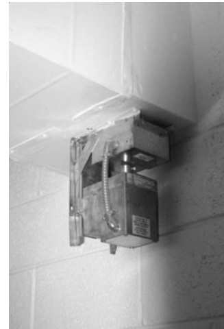
PHOTO 7.27 A damper motor used to control the position of a set of dampers (not visible) inside the duct. (Used with permission of ABC)
