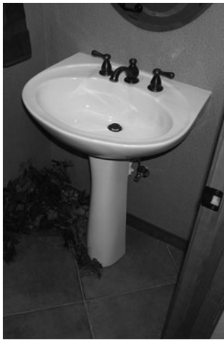
PHOTO 12.23 A pedestal lavatory. (Used with permission of ABC)
