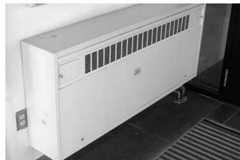
PHOTO 7.38 A cabinet heater. (Used with permission of ABC)
