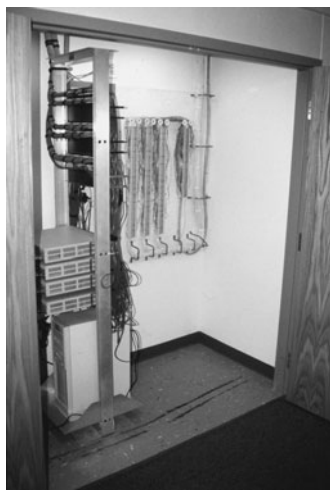
PHOTO 22.6 Telecommunications closet. (Used with permission of ABC)
