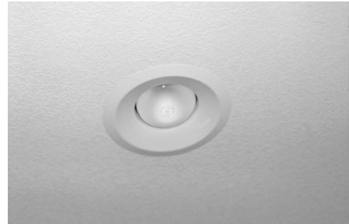
PHOTO 20.17 A surface-mounted floodlight luminaire. (Used with permission of ABC)
