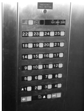
PHOTO 24.6 An elevator controller. Note that Floor 13 is “missing.”
