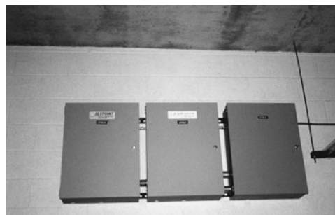
PHOTO 22.9 Wall-mounted telecommunications panels. (Used with permission of ABC)
