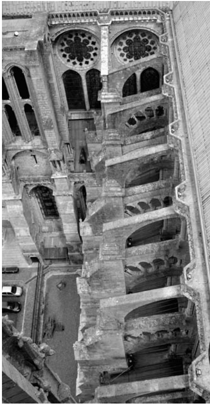
Figure 3.23. A sequence of flying buttresses bracing corresponding sets of ribs and columns. Photo by Harmonia Amanda
