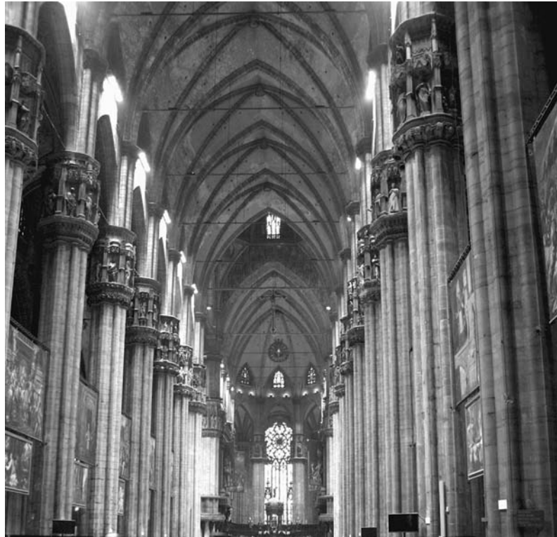
Figure 3.29. Some of the main piers of the nave with capitals and iron binding rods, and Gothic vaulting of the Milan Cathedral. Photo by Giovanni Dall'Orto
