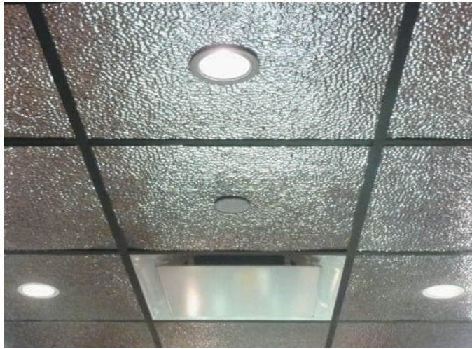
FIGURE 6.1 A change from the patterned ceilings of the past, this contemporary ceiling in the Houston Toyota Center has a shiny finish. Photo courtesy of Chelsea Decorative Products.
