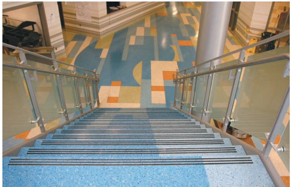
FIGURE 4.9 Solid colored Key Resin terrazzo was used on the stairs and multi colors were used in the lobby of a High School. Photograph courtesy of Michael McBride of Abingdon Industries.
