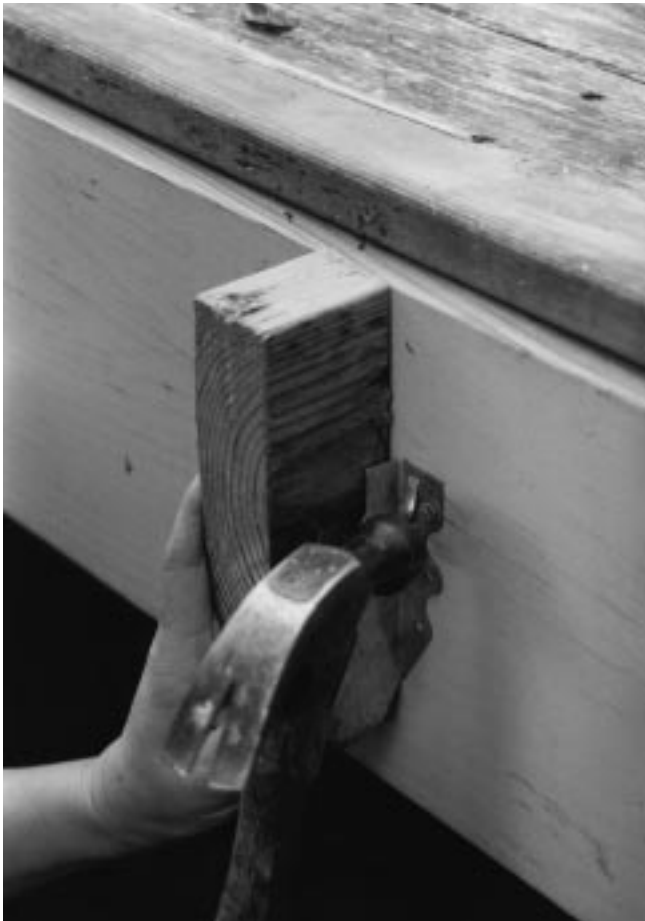
Figure 29–12 Installing joist hangers. The block positions the hanger at the correct height. The prepunched tabs are driven in to hold the hanger until nails can be installed.
