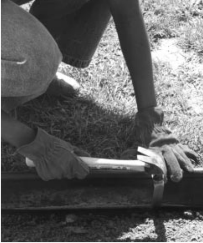
Figure 36-6 Staking plastic edging by driving metal stakes through channel at bottom. Edging must be held flat against edge of trench with top flush with finish grade.
