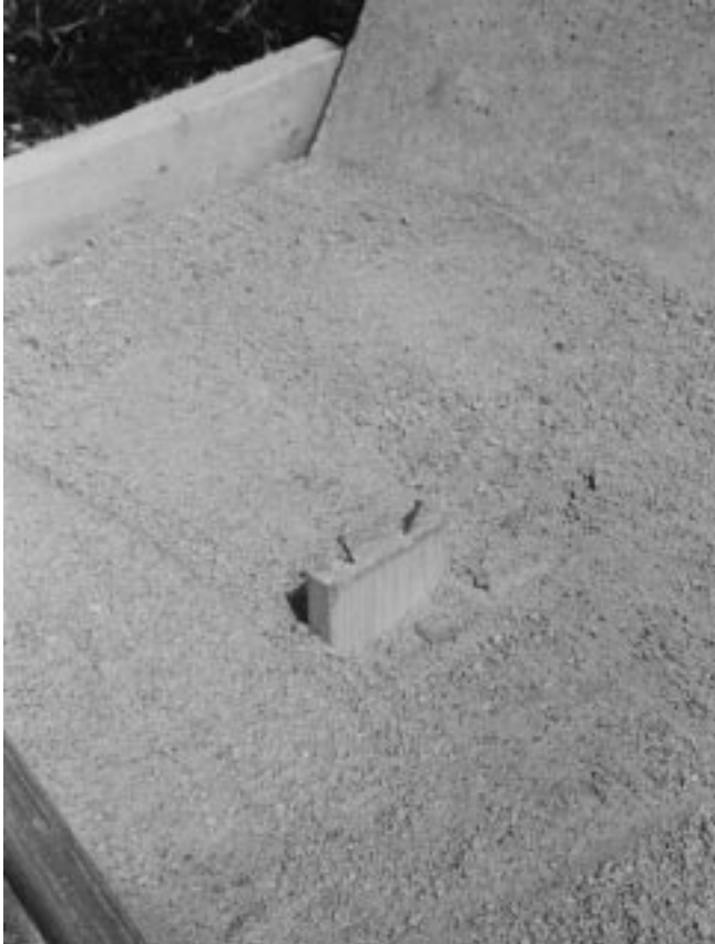
Figure 23-16 Support stakes for temporary screeding bars. These stakes will be buried in the slab; verify that nails do not project above screed bars.
