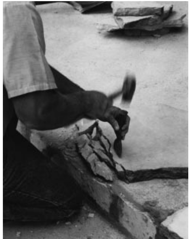
Figure 7-15 Cutting paving materials with a brick set. Set the paving material on a flat surface. Place the blade of the set along the line where you want the stone to cleave, then strike firmly with a hammer.
