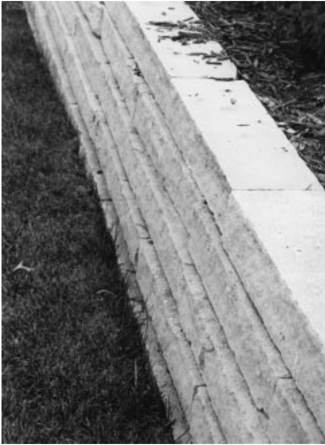
Figure 19-3 Dry-laid stone wall showing set-back batter of 1 inch with each higher course.
