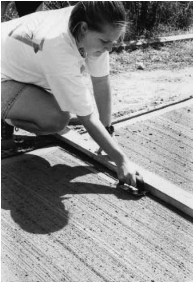
Figure 23–23 Jointing a concrete slab using a jointing tool run alongside a 2 × 4 guide.
