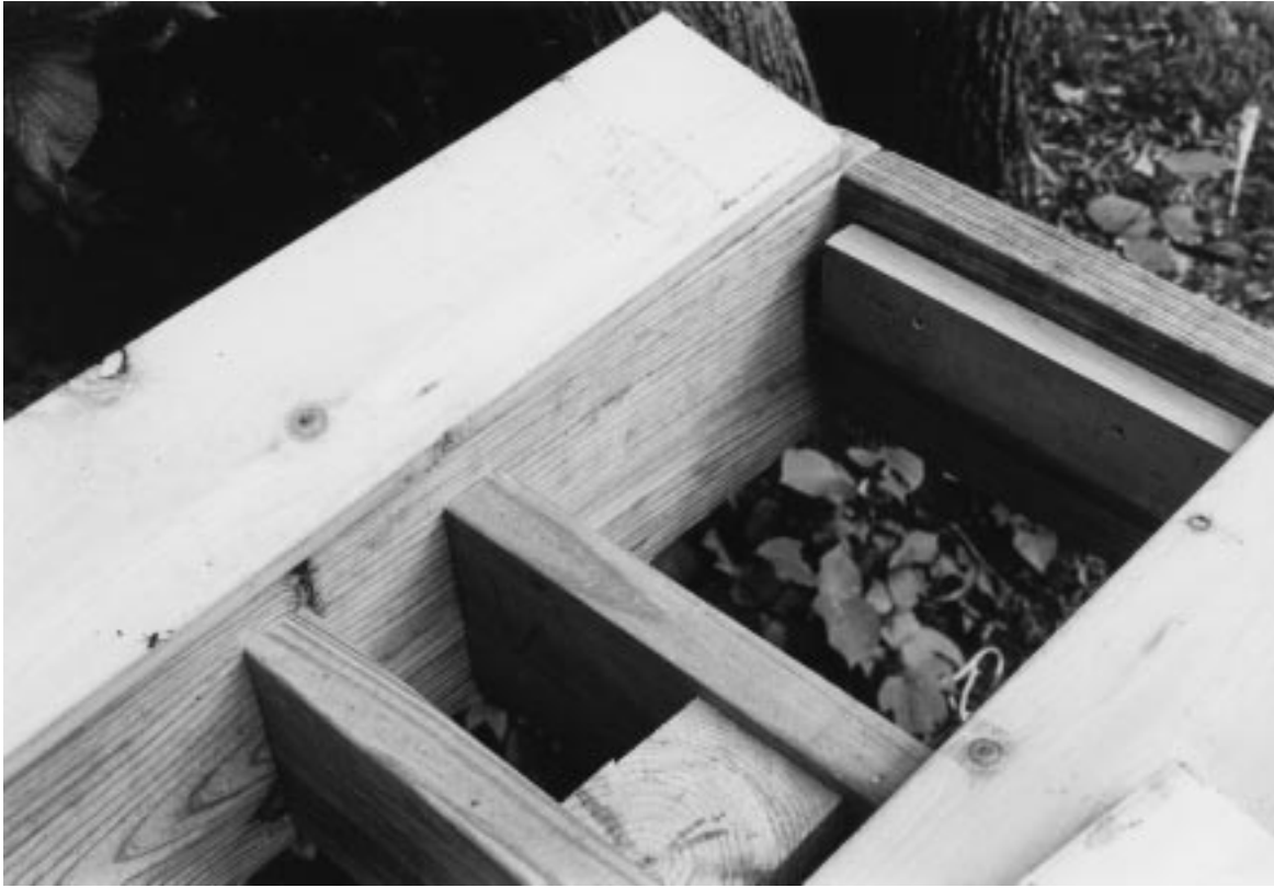
Figure 30-18 Seat surfacing inset at edges. Framing is set higher than beams to accommodate thickness of surfacing material. A cleat supports the framing at the end.
