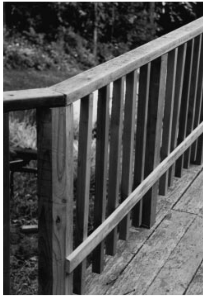
Figure 30–11 A 2 \times 4 stringer has been placed across the top of the posts. Balusters are then hung from the stringer. Surfacing of 1 \times 2 s is being installed beginning at the bottom of the balusters.
