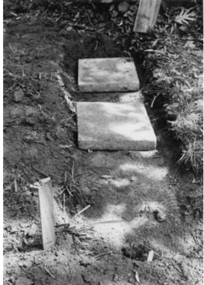
Figure 30-2 Stair landing is excavated and precast blocks are placed to support the bottom of the carriage. The stake in the front left is marked with the level required for the top of the precast blocks.
