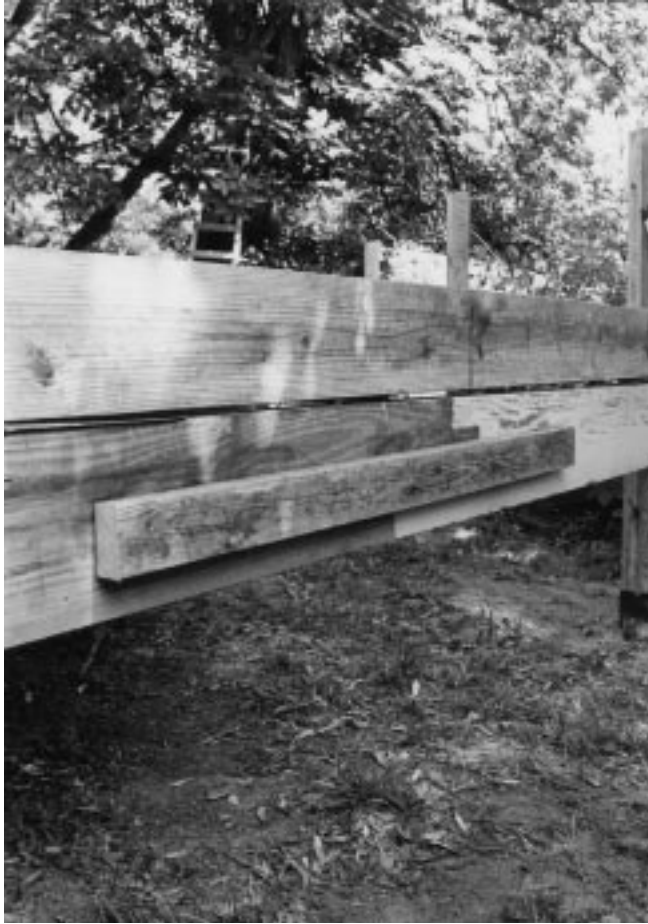
Figure 30-1 Extra stair supports. The bottom 2 × 10 provides a solid surface to nail to and the 2 × 4 assists in supporting the bottoms of the stair carriages.
