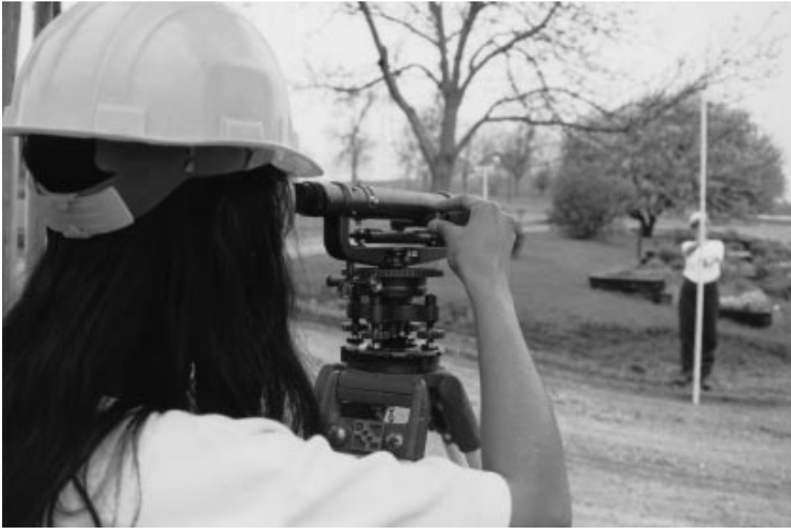
Figure 8-10 Focusing a survey instrument. Use caution not to bump the instrument out of level.
