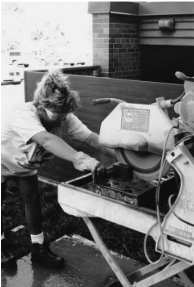
Figure 7-17 Cutting paving materials with a wet masonry saw. Cutting with a masonry saw is slow but accurate.
