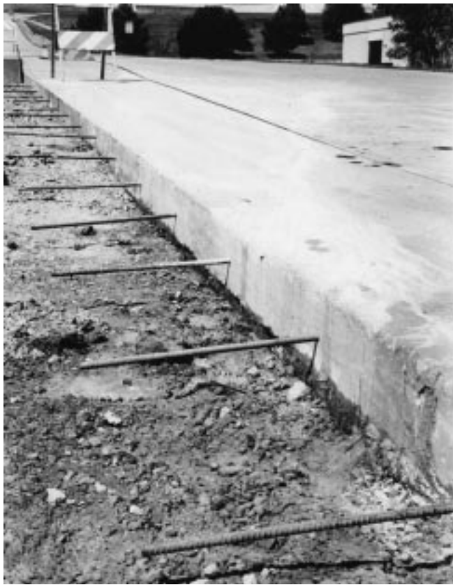
Figure 23-6 Rerod placement along edge of pour to anchor new slab to existing slab.
