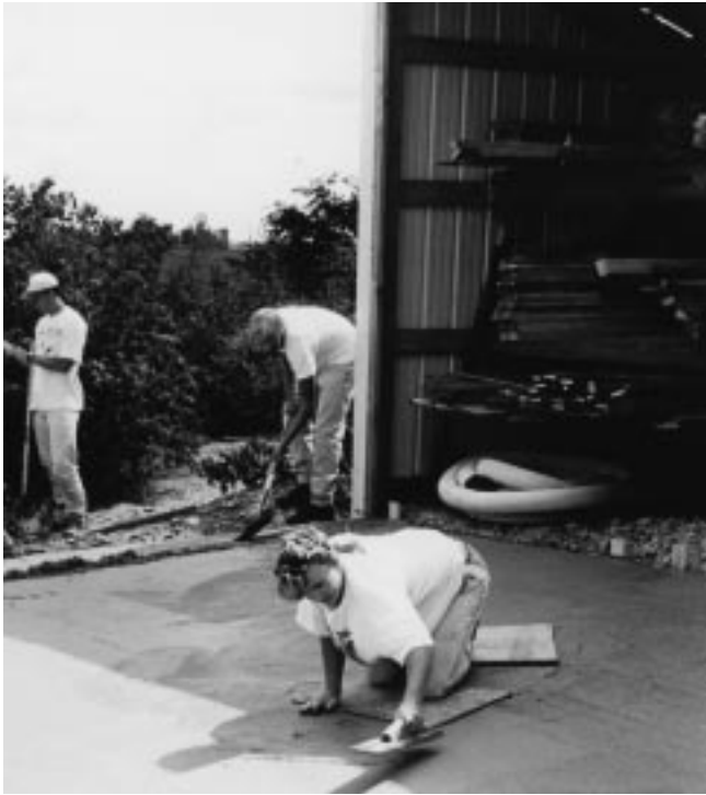
Figure 23–21 Using kneeboards to reach center of a concrete slab for floating. Concrete must begin to set before boards can be placed on slab.
