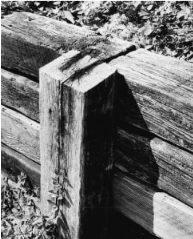
Figure 16–12 Vertical tie anchor for a stacked tie retaining wall. Note that the vertical is placed at the joint between wall sections.
