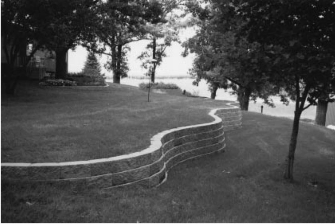
Figure 16-2 Segmental precast concrete unit retaining wall. (Courtesy of Gary Pribyl, Kings Materials)
