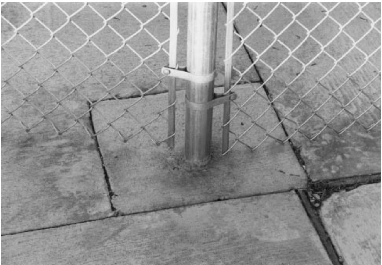
Figure 32-21 Chain link fence post set in concrete. Concrete slab was poured earlier. A box was left out in which the fence post and footing could be placed.
