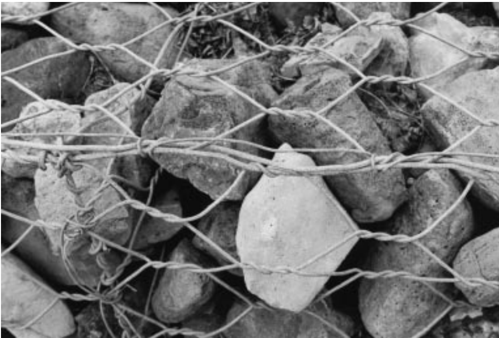
Figure 20-2 Gabion cages are filled with stone larger than the diameter of the cage openings. Cages are wired shut using 12 gage galvanized wire.
