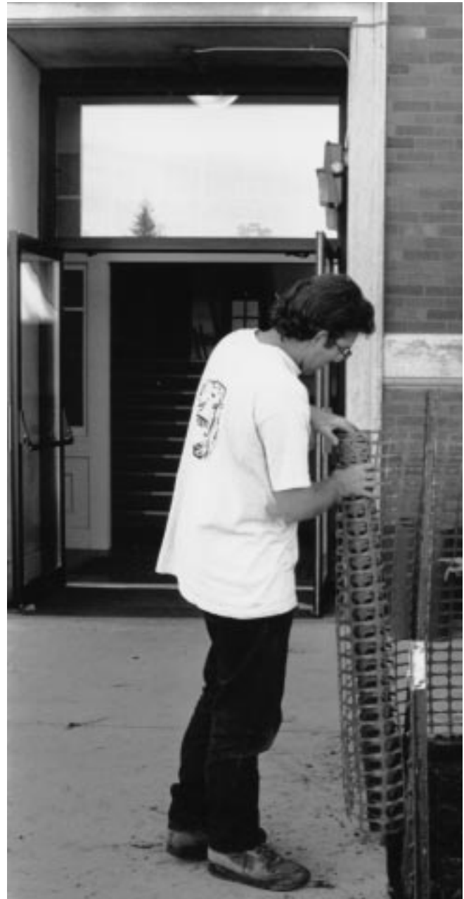
Figure 9-5 Installing temporary fencing at a construction site to protect public from hazards.
