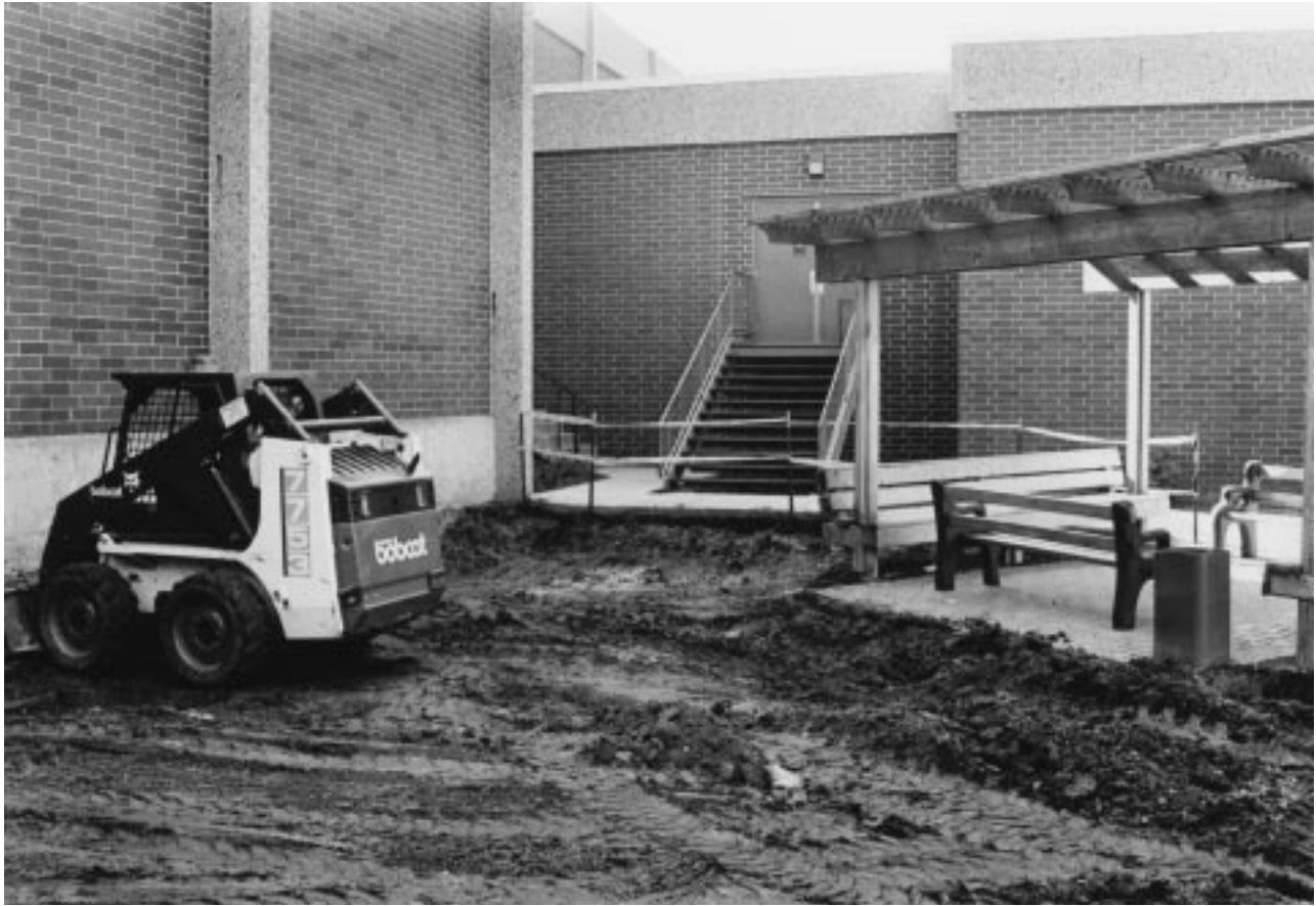
Figure 22–7 Using a skid-steer to excavate the base for an expanding paved area.
