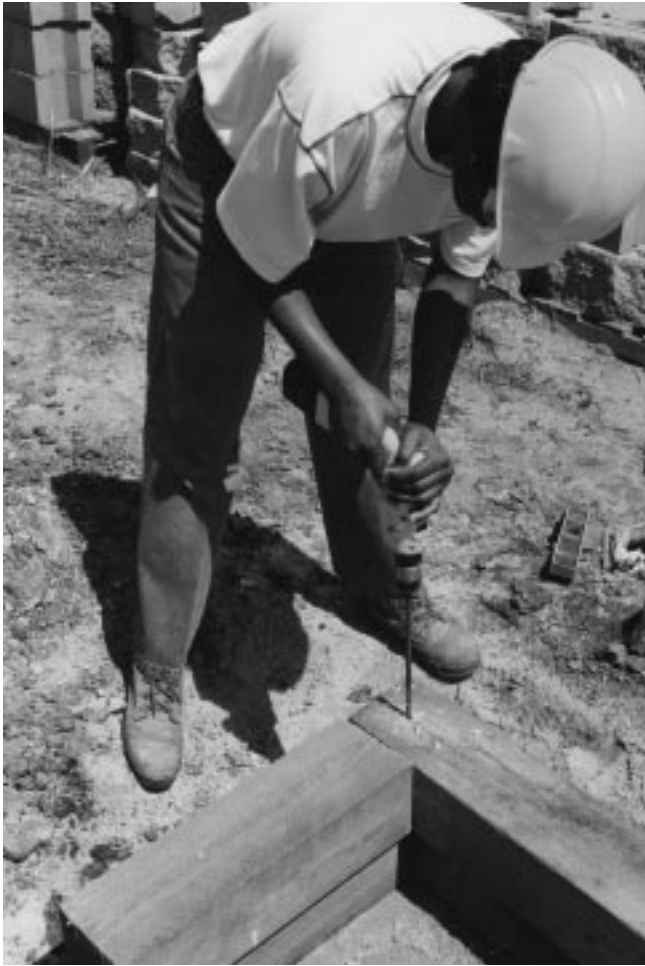
Figure 17-8 Drilling holes in timber with a cordless drill for 3/8 inch \times 10 inch spikes.
