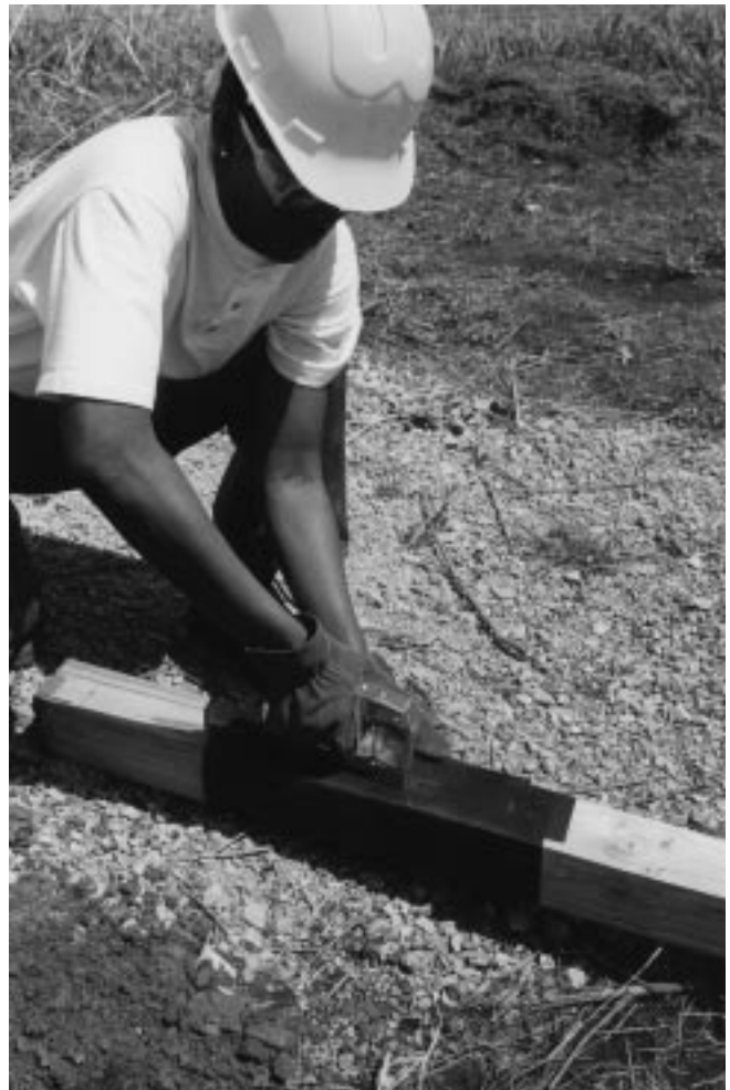
Figure 29–4 Stapling roofing felt around a direct burial post. Felt extends 6 inches above and 9 inches below the ground line.
