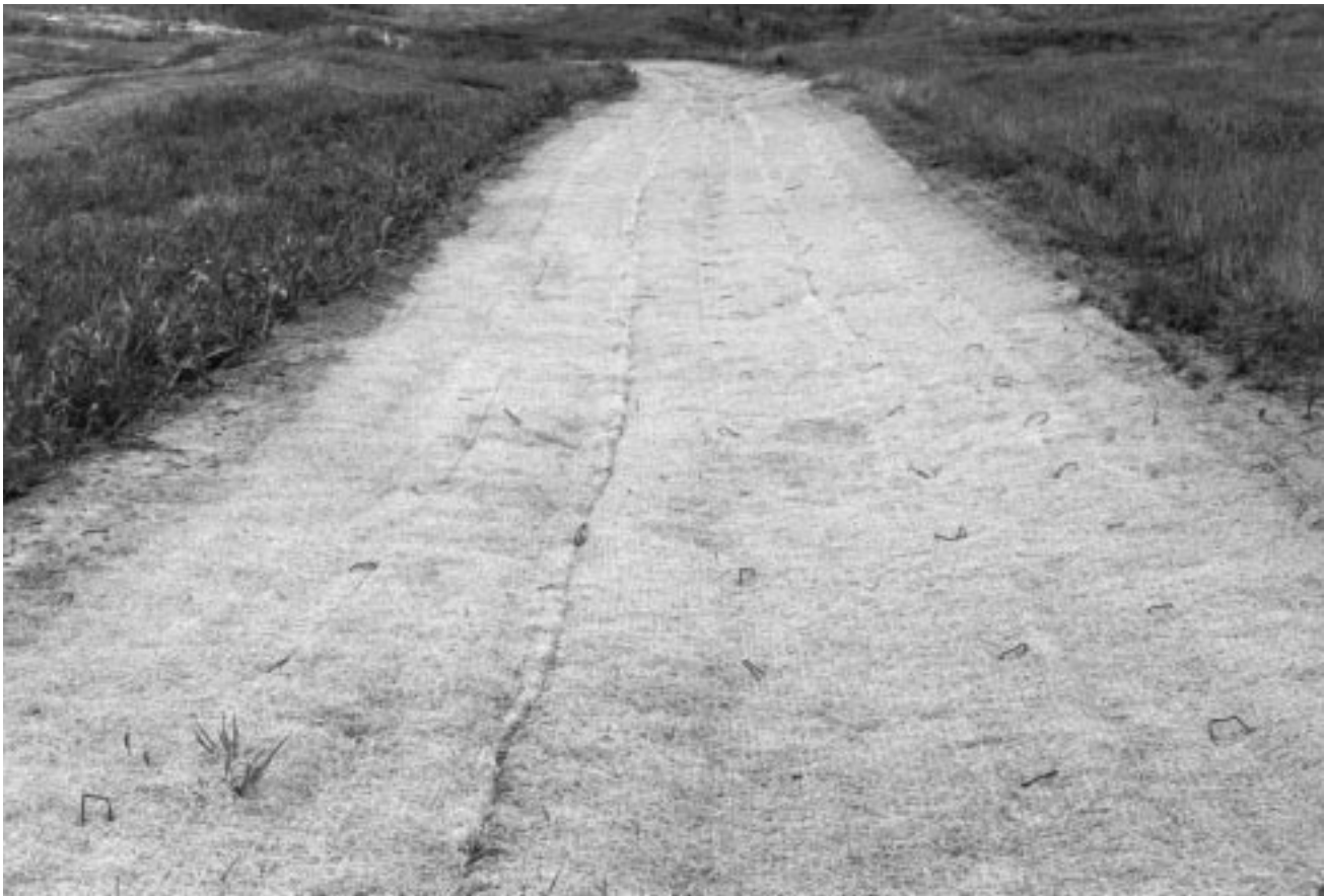
Figure 13–2 Placement of erosion mat along length of a channel. Note that the mat is placed with the long dimension running the same direction as water flow.
