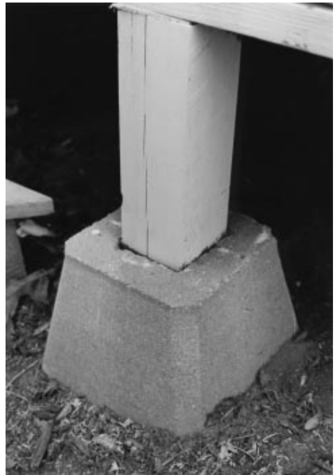
Figure 29–6 Precast concrete pier holding a support post.
