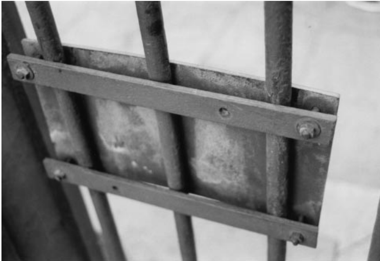
Figure 35–5 Attachment of signage to decorative metal fencing. (Courtesy of Margaret Sauter)
