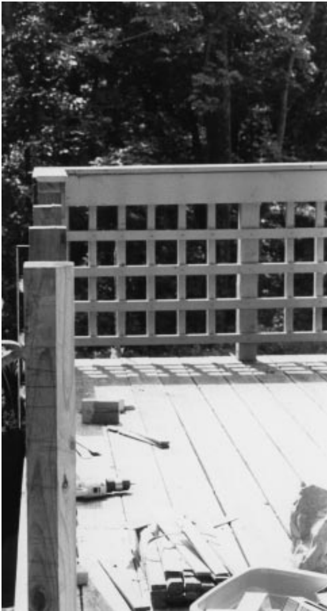
Figure 30–10 Railing post installation. Decking material has been marked and cut to place pots through deck surface to structure below.
