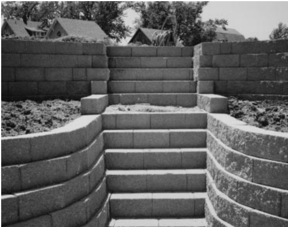
Figure 21-9 Completed interlocking stairs with precast segmental units. (Courtesy of Gary Pribyl, Kings Materials)
