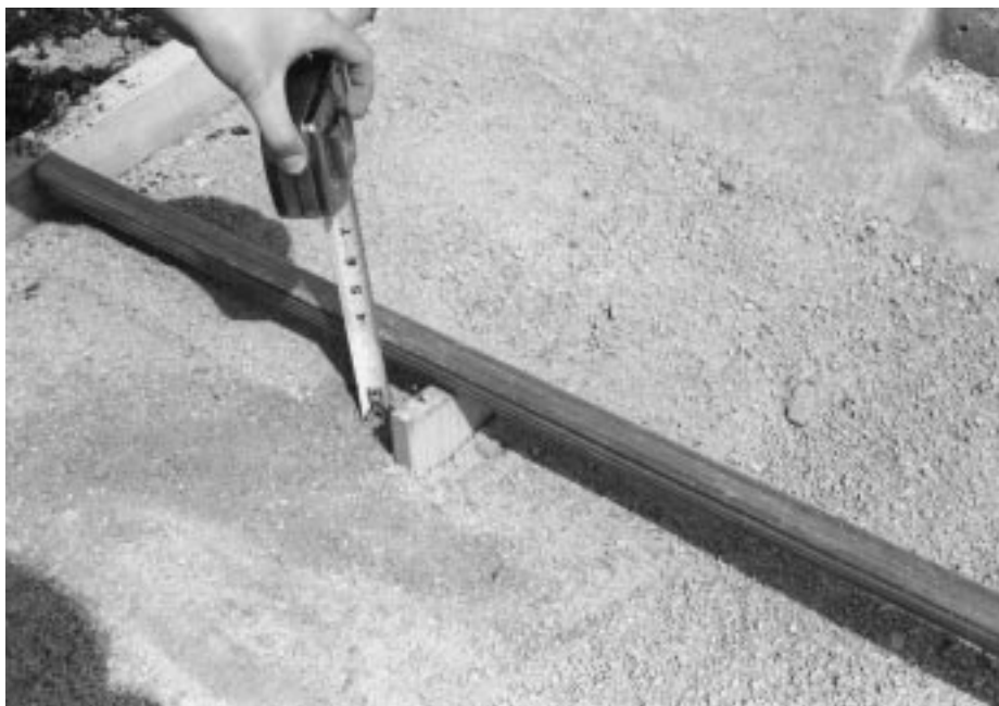
Figure 23-17 Temporary screeding rails used for screeding wide pours. The top of the rail should be set at the desired thickness of the slab.
