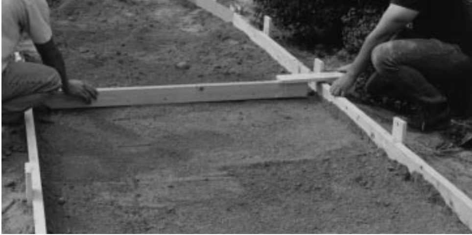
Figure 23–11 Screeding 3/8s minus granular base to a consistent depth. Base will be compacted after screeding.
