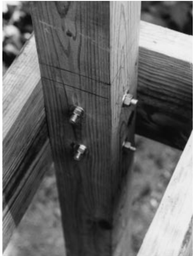
Figure 29-11 Post to joist connection using carriage bolts. At this corner, bolts are installed from both sides. Markings indicate top and bottom of deck surfacing.
