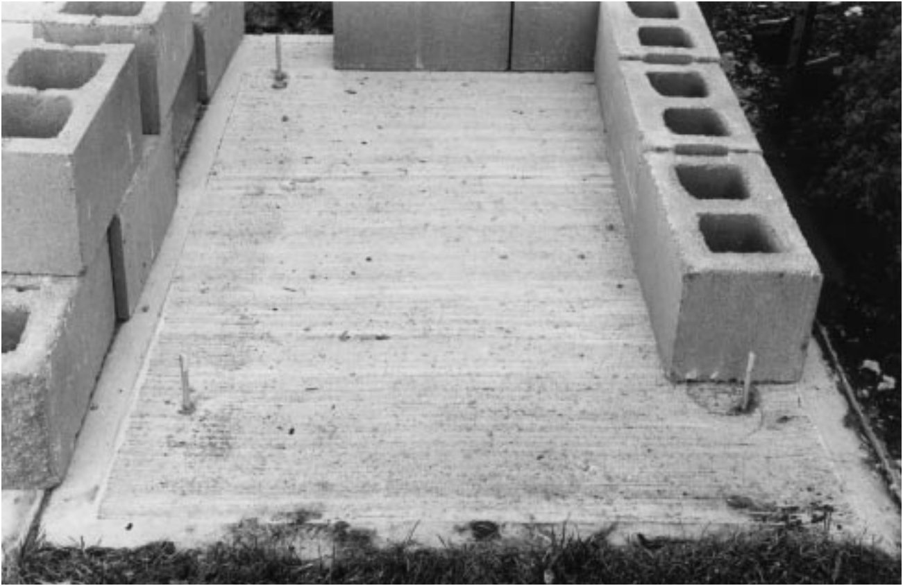
Figure 33–5 Masonry pier footing installation, showing bond chasing and anchor bolts placed when foundation was poured.
