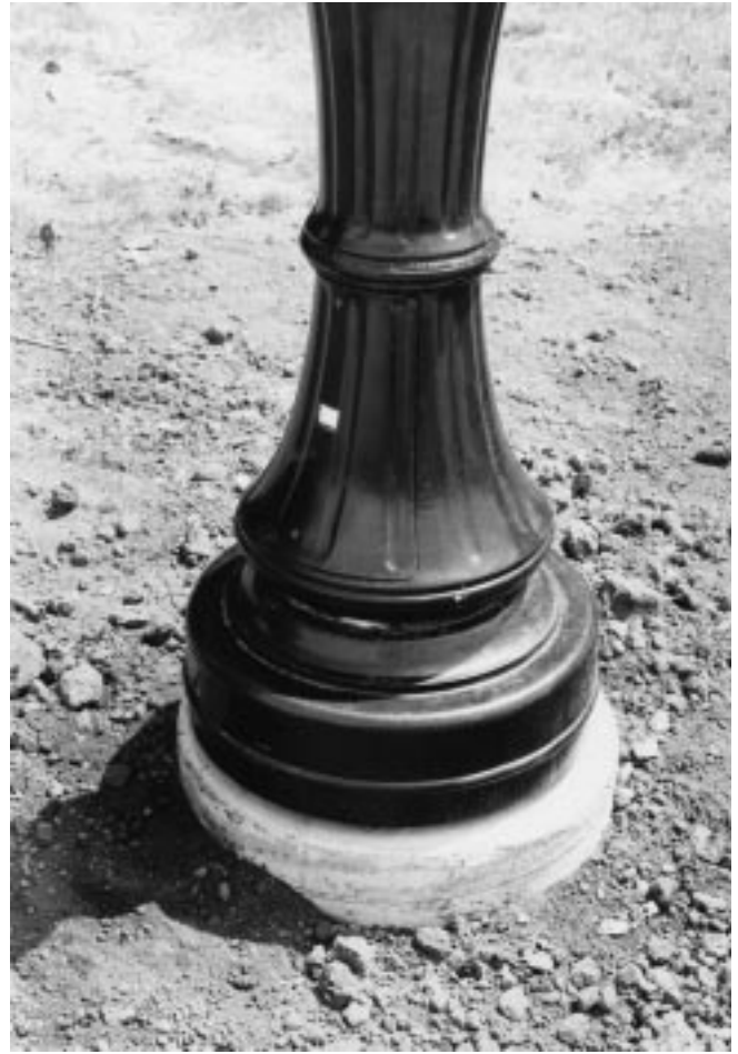
Figure 14–10 Handhole at the base of a lighting standard. Electrical connections are made inside this handhole after the fixture has been installed.
