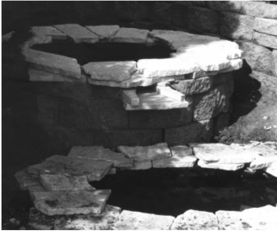
Figure 34–12 Construction of a wall between flexible liner pools set at different levels. The upper pool is adjacent to the lower pool with a waterfall planned between the two.
