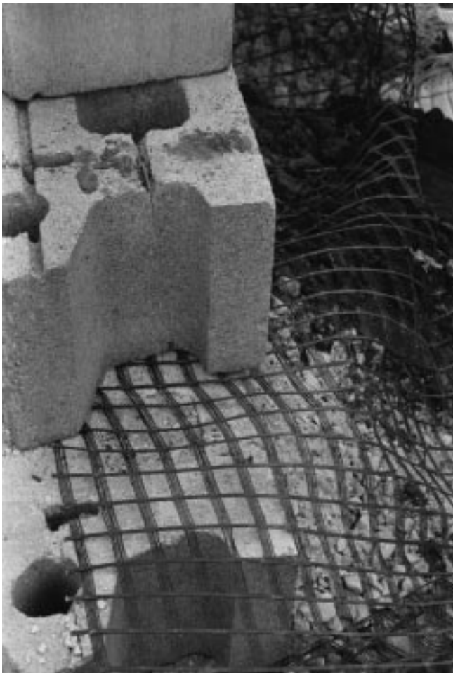
Figure 18–6 Geogrid placement between courses of precast segmental units. Geogrid should be hooked over the fiberglass pins before placement of following course.
