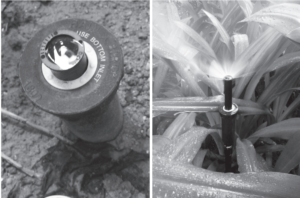
Figure 10.1 Popup spray sprinkler heads that will emerge when it is time to water the plants and submerge when the watering is done.
