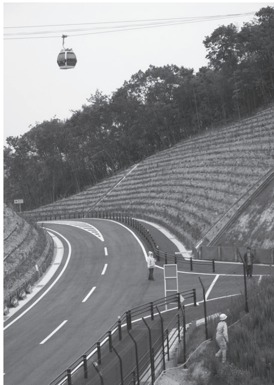
Figure 6.10 Structure built to prevent soil erosion on the slope and which is supported by vegetation
