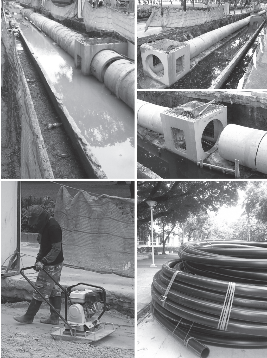
Figure 4.15 The construction of the new closed drainage system in chulalongkorn University. The old road surface was stripped to make way for the drainage system and other public utilities. Then they were covered, graded and paved with concrete.
