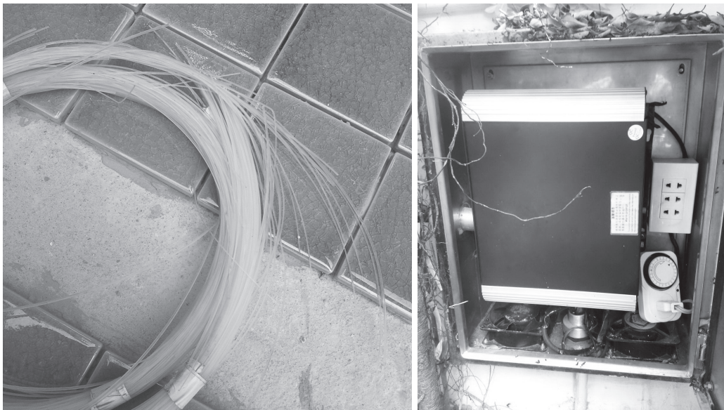
Figure 8.7 Fiber optics for lighting in the swimming pool, flickering (left) and the control box and timer (right)
