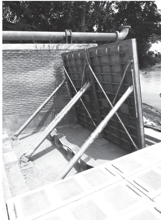
Figure 5.7 Semi-temporary flood prevention using a levee in front of Chaiwattananram Temple, Ayuttaya Province. The levee can be raised during the rainy season (above) and folded down so that the temple can be seen from afar in the dry season (below).
