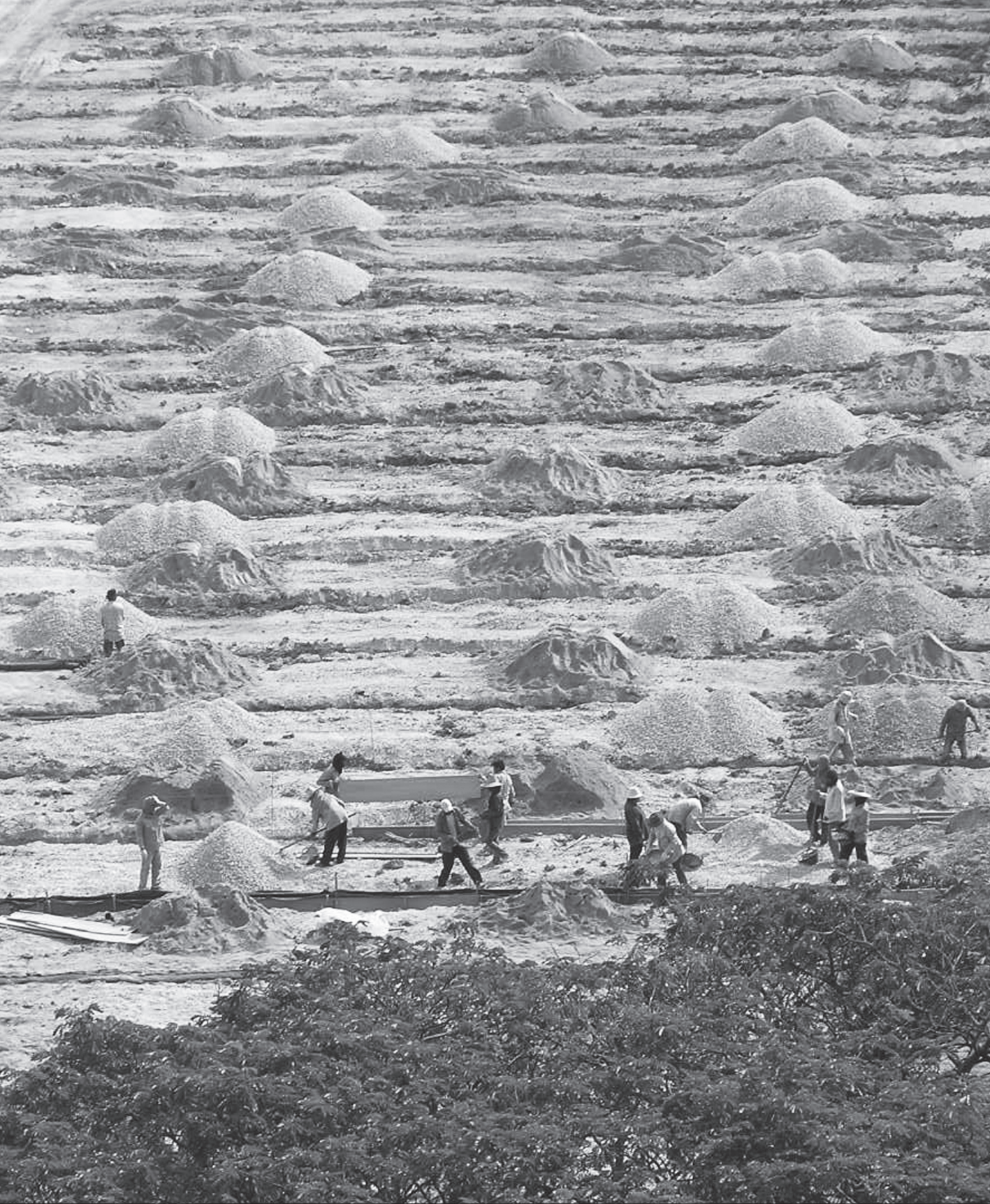
The laying of a parallel subdrain to solve the problems of high underground water level and slow drainage of multi-functional lawn in front of the Memorial of the Two Kings at Chulalongkorn University. The Figure shows the stripping of topsoil to put porous pipes in the ground and cover them with gravel and sand before growing grass on top.
