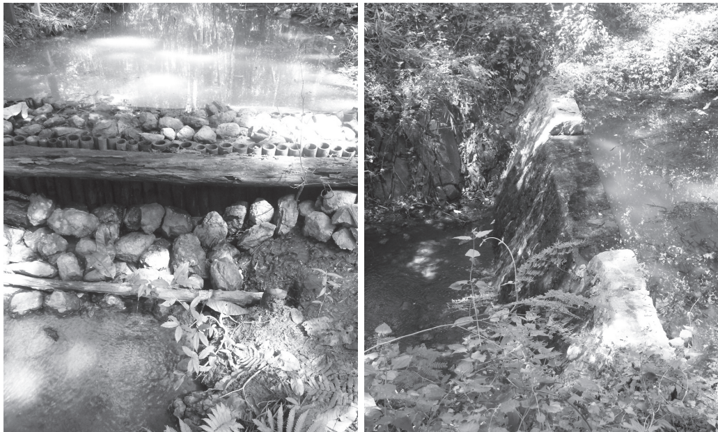
Figure 5.17 A temporary weir (left) and a permanent check dam (right) to restore dilapidated forest areas in the Huay Kong Krai Royal Development Study Center. This is a center for studying the restoration of forest areas at the source of water.
