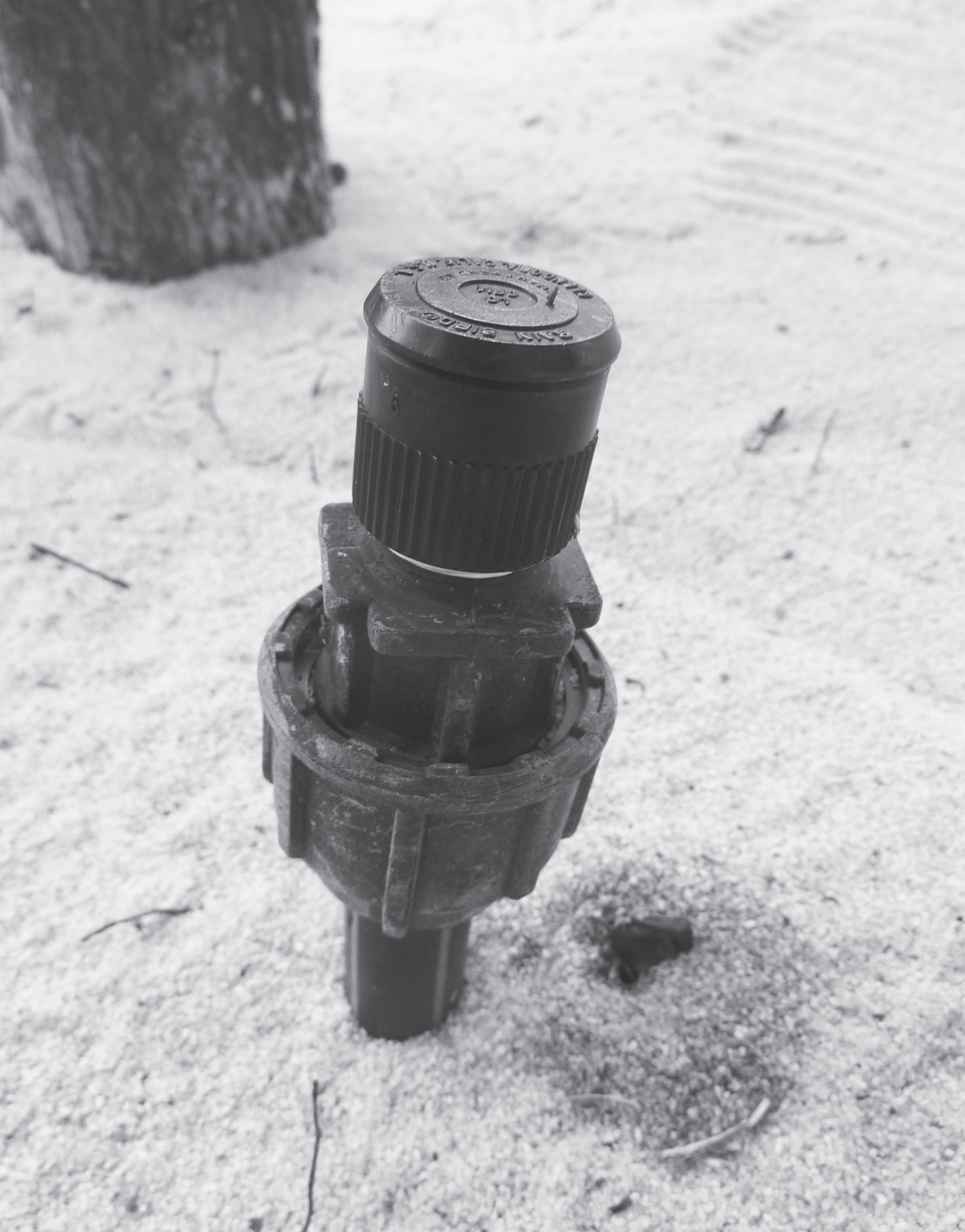
Popup spray sprinkler head
