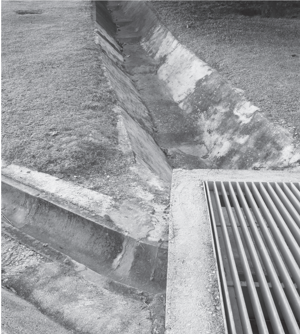
Figure 4.8 The open drainage system in the slope landform. The slope surface should be paved to prevent erosion.
