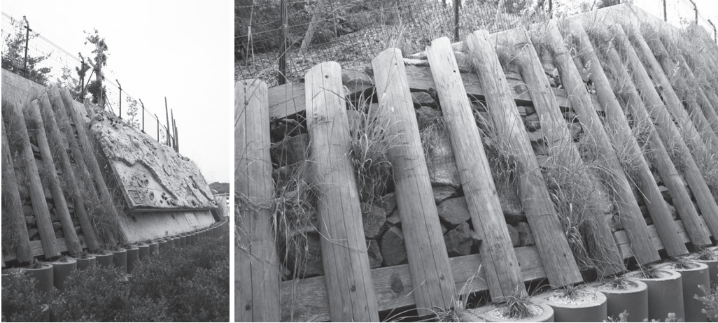
Figure 6.9 Retaining wall made of natural materials such as wooden posts made into a box for holding rocks; as a result, vegetation or weeds can grow on it
