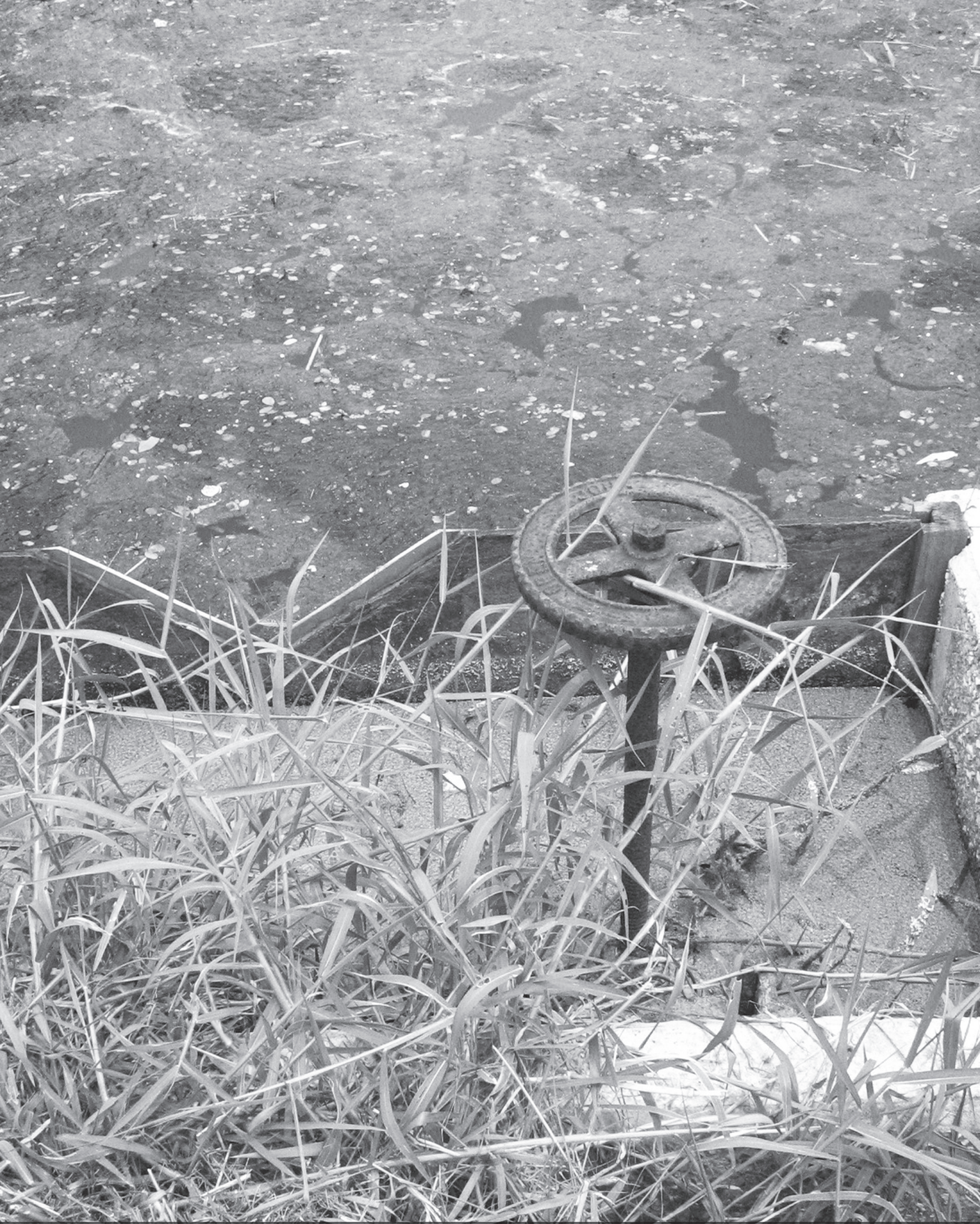
A pond for collecting wastewater from the project before going to a facultative pond. The water is black or dark grey and smelly. Its BOD is likely to be over 20 milligrams/liter.
