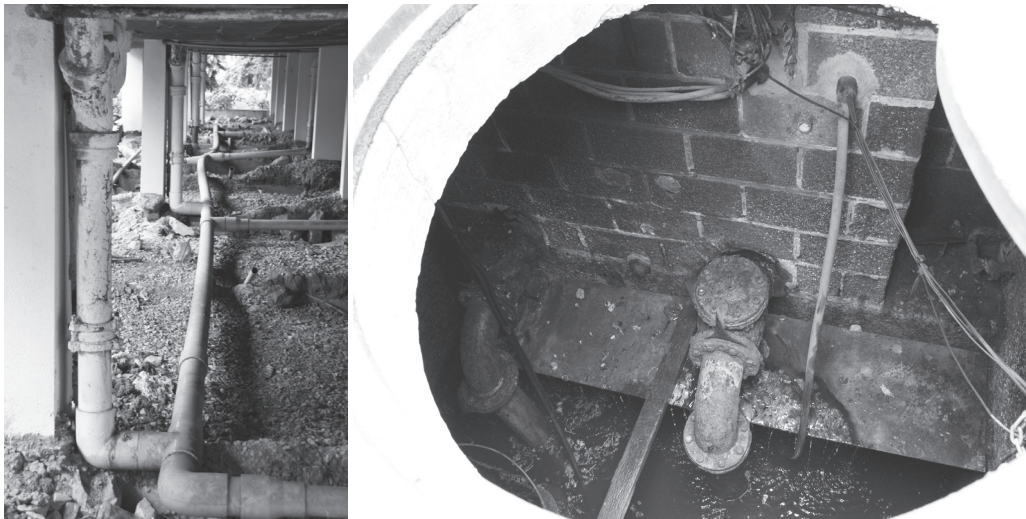
Figure 9.1 The area to collect and treat wastewater from the sources – toilets and washing area. The wastewater is carried through the pipe (left) to the area (right) to be treated.
