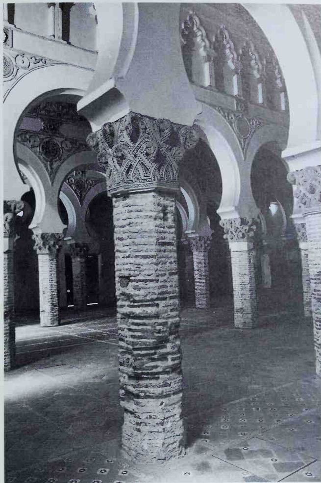
Santa María la Blanca: the piers temporarily stripped of plaster to reveal the brickwork.
