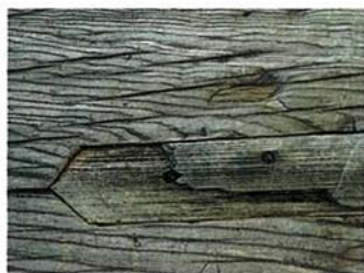
This close-up of a post at Hōryūji Temple, near Nara, demonstrates one method of preservation: cutting out a rotted piece of wood and replacing it with a plug made from the same kind of material.
