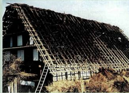
A roof after the old thatch has been removed in preparation for rethatching.
