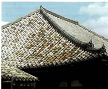
The Main Hall and Meditation Hall at Gangōji Temple. These beautiful multicolored tiles, made by Korean craftsmen in the Asuka Period, are the oldest tiles in Japan. The more recent tiles used on the adjacent roof slope to the right are more uniform in color.
