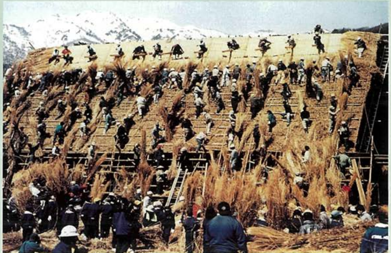
A roof being rethatched. About 100 people are on the roof of the house, with 300–400 more working inside or on the ground.
