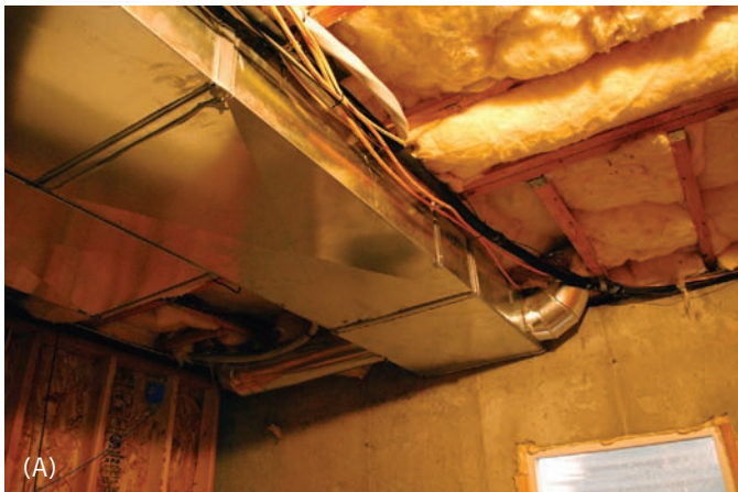
Figure 7.23 (A) Ducts or ductwork is the system that brings heated air from a furnace to all areas of the home. This shows ductwork in an unfinished basement and insulation in the floorboards, to be covered later with Sheetrock when the basement is finished. The smaller duct leads to a register in the floor. Rough electrical wiring is also seen here. (B) This central air-conditioning unit provides refrigerated air to the home. These units are efficient, but generally costly to run in terms of electricity used. Photo © Kathryn Taylor
