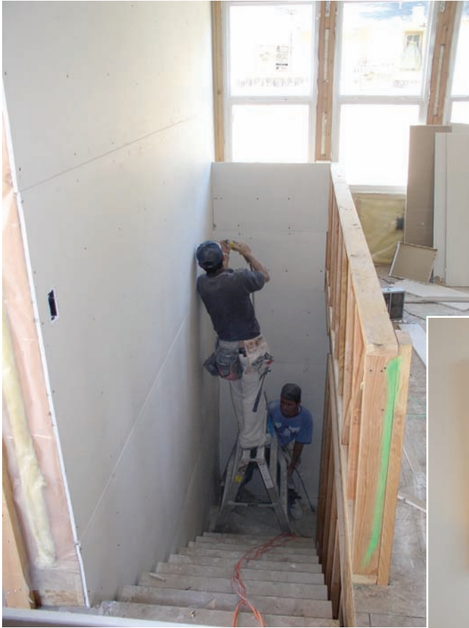
Figure 7.17 Sheetrock may be finished as rough plaster, as lightly textured, or with a smooth finish. Here installers attach drywall panels with screws. The seams will be covered with plaster (mud) and tape, and the screw holes will also be filled with plaster. Photo © David A. Taylor
