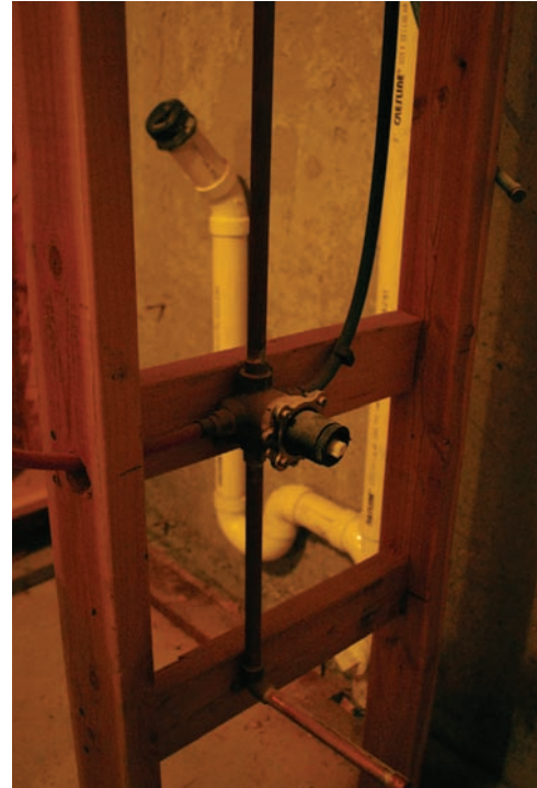
Figure 7.19 Rough plumbing is installed after the wall is framed. The black and copper pipes will carry fresh, culinary water to sinks, dishwashers, bathtubs, showers, and washing machines. The larger white pipe will carry away the waste water. Photo © Kathryn Taylor
