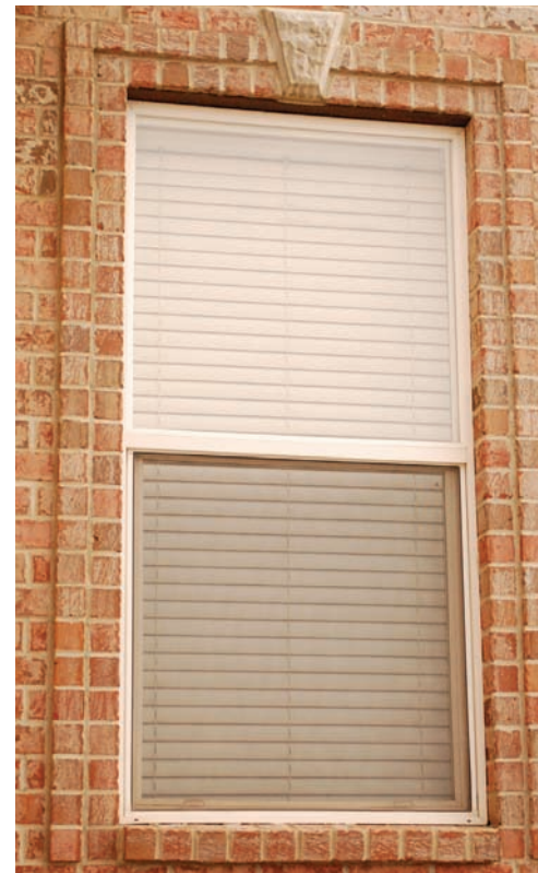
Figure 7.16 Windows are installed and framed here with brick masonry. Photo © Kathryn Taylor
