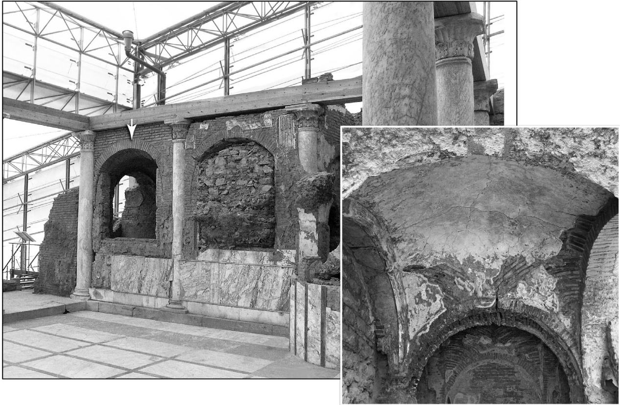
51. Peristyle of Residential Unit 6 in Terrace House 2 at Ephesus showing original portico infilled for the addition of a bath suite. Arrow indicates location of inset photo of the fan sail vault. Note the crack in the middle of the vault.
