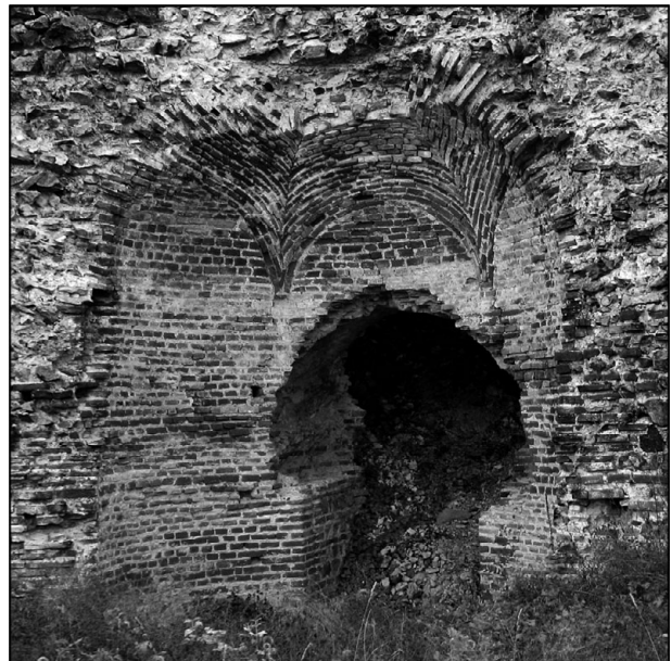
59. Palace of Galerius at Gamzigrad, Serbia (ancient Felix Romuliana) (early fourth century CE). Photo of sail vault from one of the towers of the fortification walls (photo: Ulrike Wulf-Rheidt).
