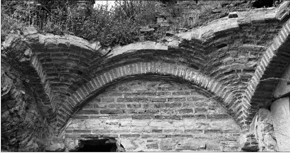
48. Terrace House 1 at Ephesus (mid-second century CE). Upper stair vestibule of Domus with sail vault built using the fan method of laying the bricks.
