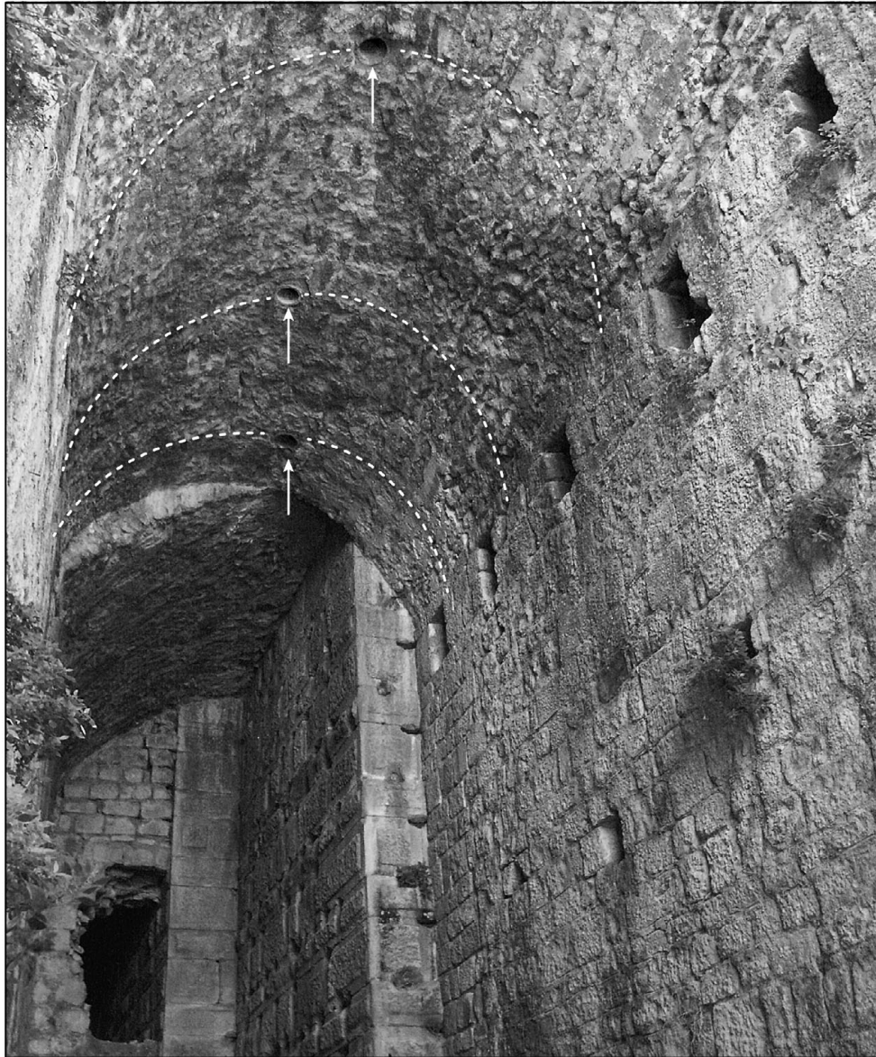
6. Temple of Trajan, Pergamum (117–136 CE). View of substructure chamber. Arrows indicate vertical tubes in the crown of the vault, which are positioned between the rectangular centering holes visible on the right.
