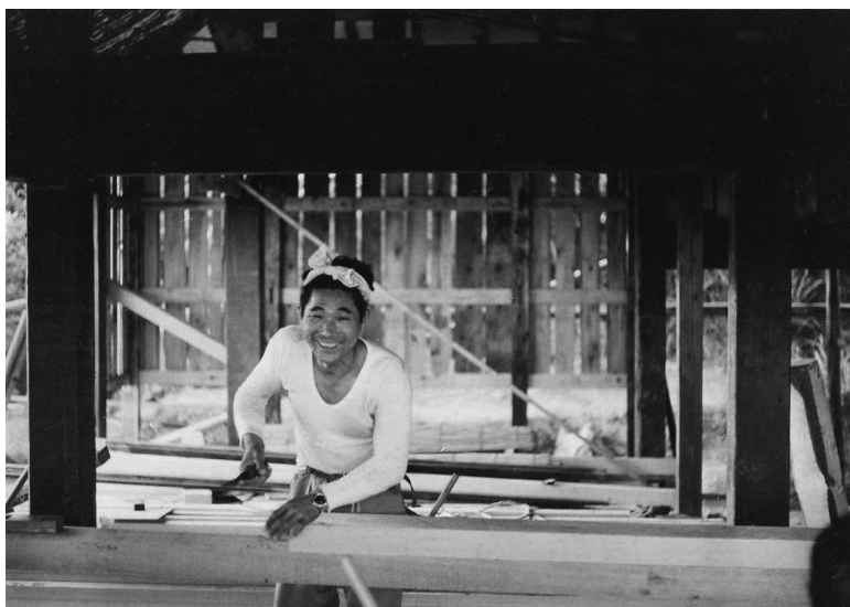
Daiku-san Taizou Miwa works in what is to become the living room.
