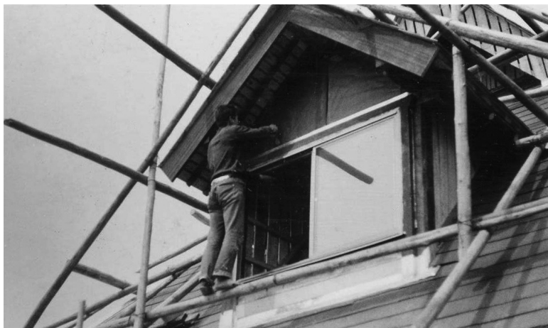
Tadashi Mizoguchi applies plaster to the area above the west dormer window.
