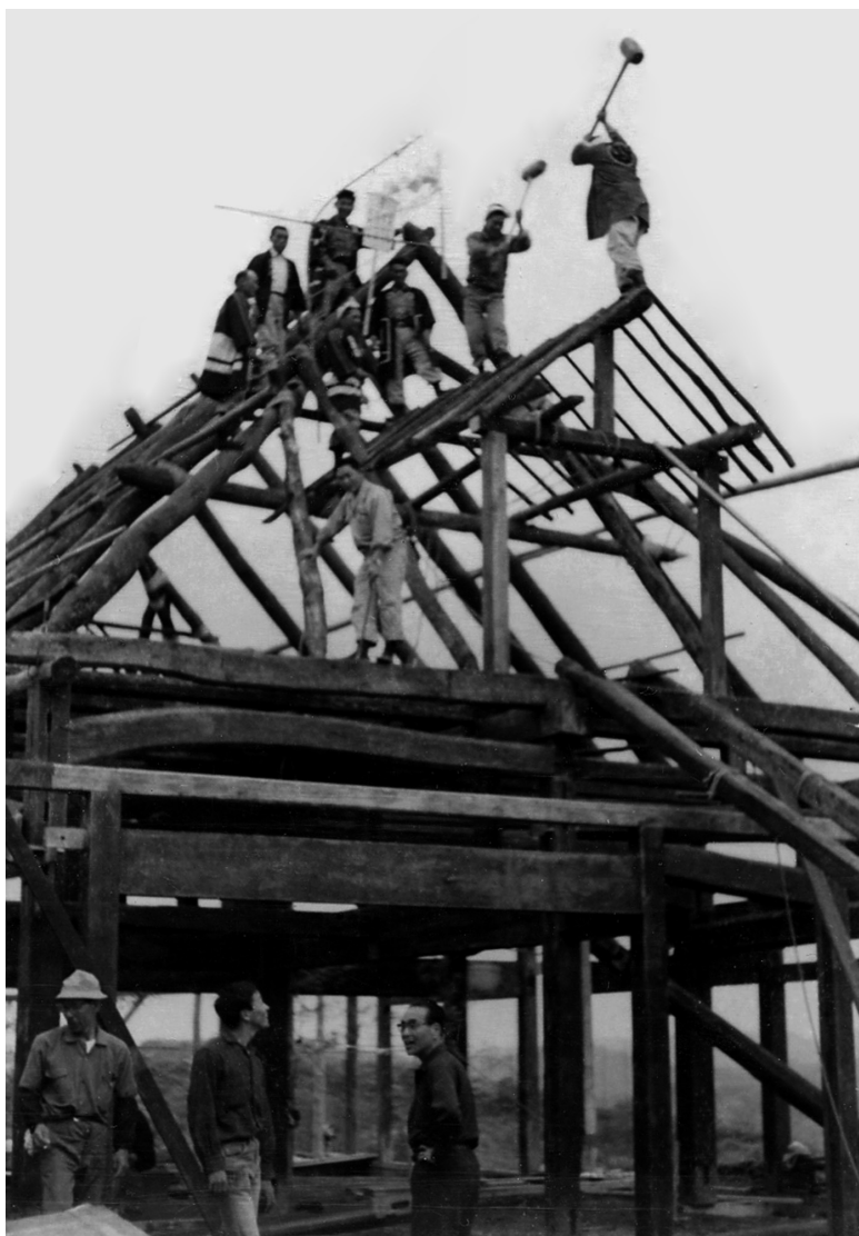
Using mallets, just as the carpenters of Ise did in 1734, the daiku-san ceremoniously install the roof ridge pole; uncle Kakehi, Yochan, and Katoji watch below.
