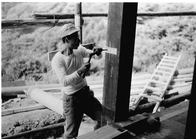
Etori Kaneshige preparing to create a window sill on one of the pillars.
