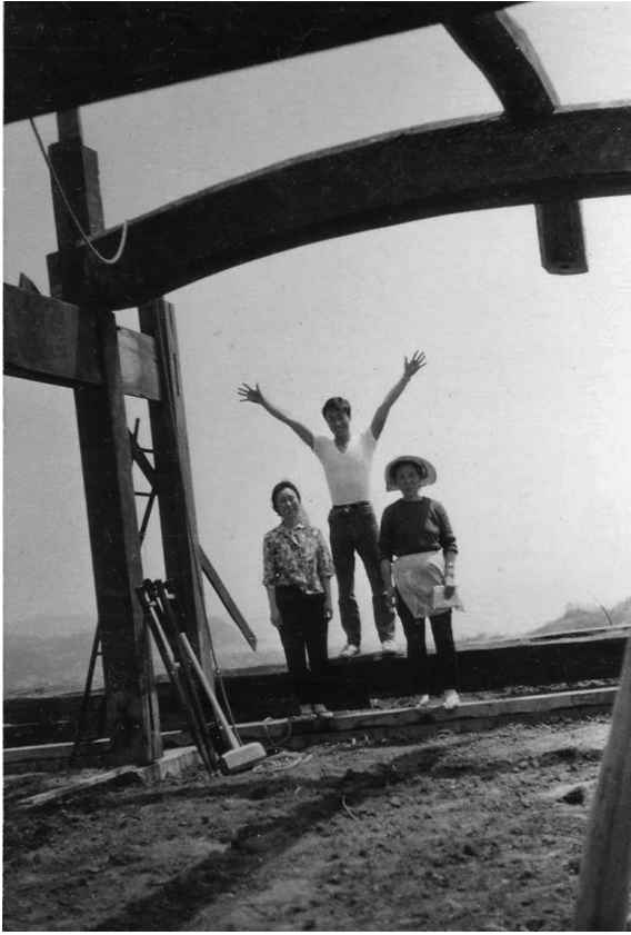
Yochan, his aunt Kakehi, and Kazu below the most massive transverse curved beam
