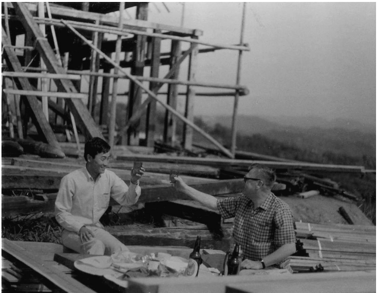
(top) Carpenters begin laying the wooden sheath that will support the roof. (bottom) Yochan and I raise a glass to toast progress so far.
