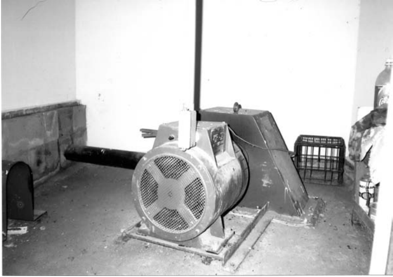
Fig. 2.2. Pelton wheel turbine and generator set for the microhydro-power system at Long Branch
