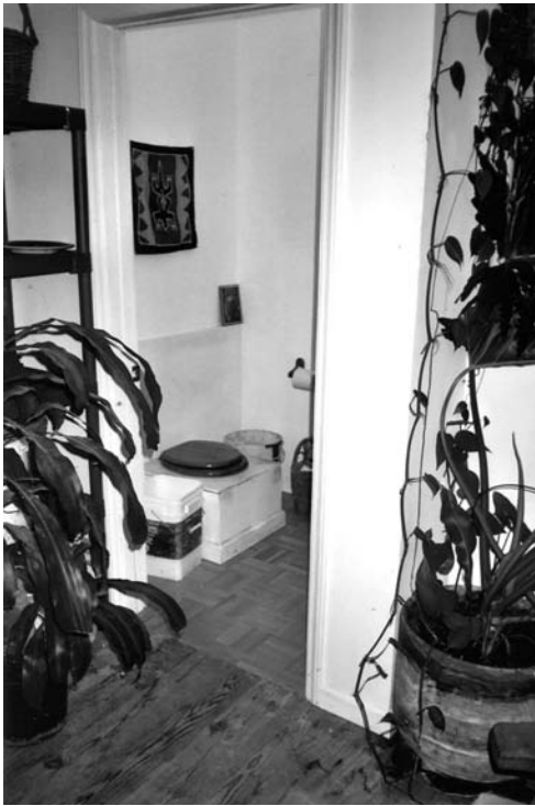
Fig. 26.4. Composting toilet inside attached solar greenhouse at Long Branch office complex
