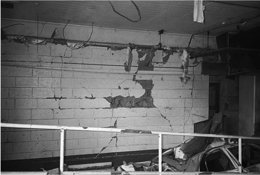
Figure 16.3 Crack Pattern on Masonry Infill Wall
