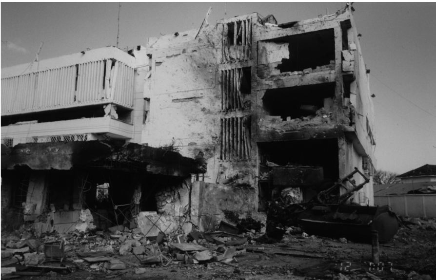
Figure 16.2 Failure of Masonry Infill Wall
