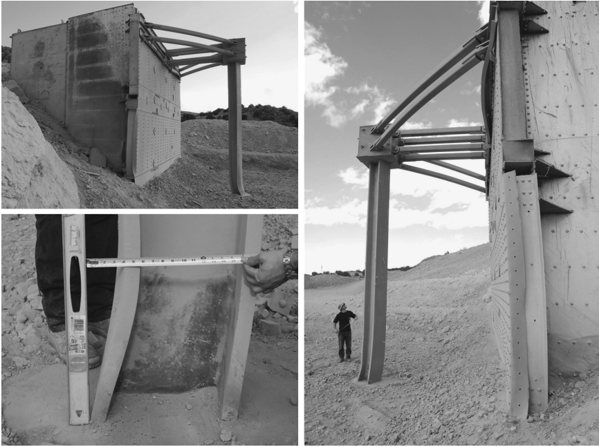
Figure 4.5 Steel Cross Section Distorted Due to Air-Blast Loading (Courtesy of American Institute of Steel Construction)
