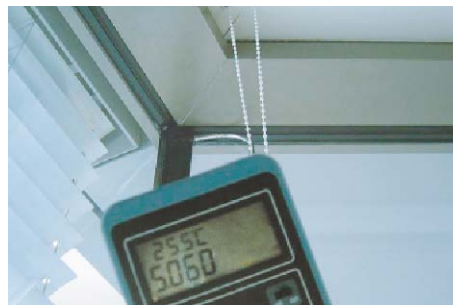
Fig. C3.2 Infiltration reading shows an untight crack at the upper edge of the glass joint.
