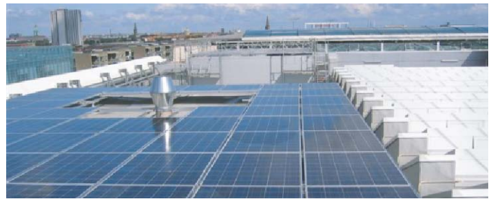
Fig. C2.28 Photovoltaic-collectors for electricity generation
