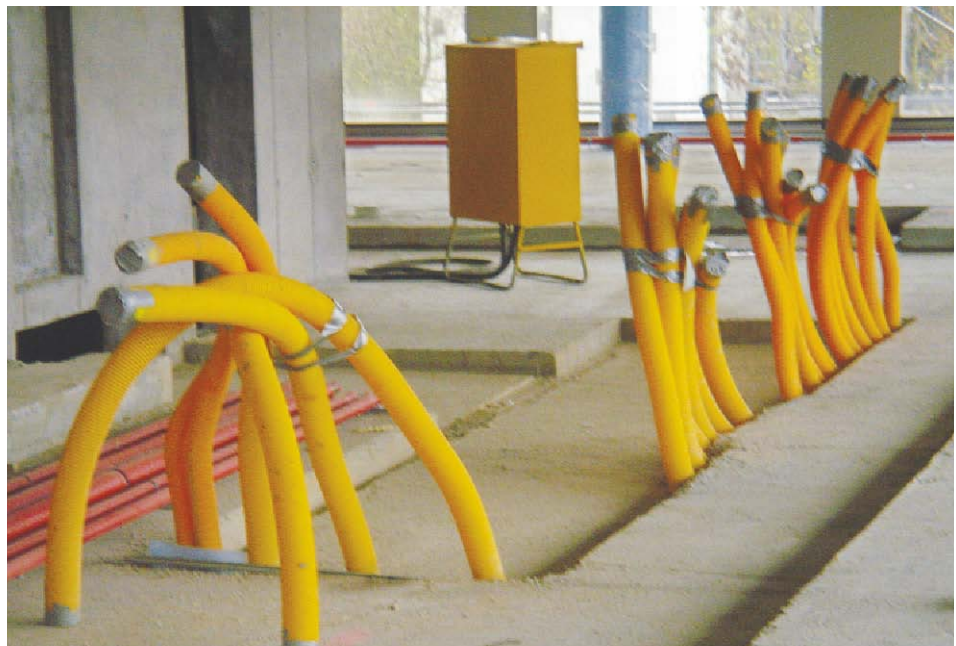
Fig. D3.11 Ventilation ducts for the offices. Distribution occurs inside the concrete ceiling.
