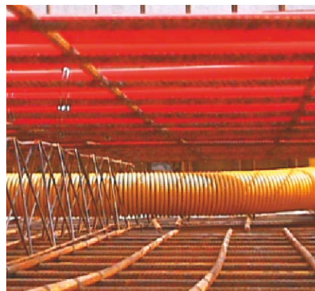
Fig. D9.2 Thermally active components and ventilation pipes, integrated into the concrete ceilings
