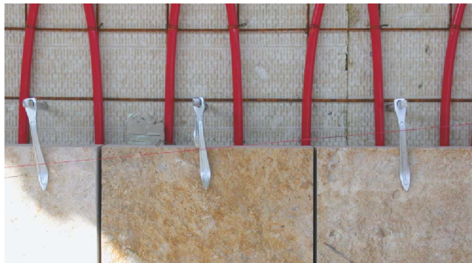
Fig. D5.3 Water-filled pipe coils serve for thermal activation of the natural stone wall
