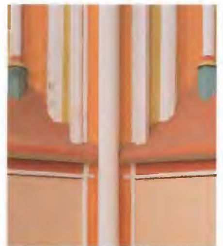
Marburg, castle chapel, consecrated 1288 View from east (top) Pier profile in choir (above)
