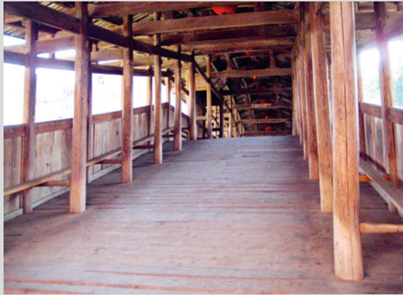
Fig. 8.12 The interior structure of the Xuezhai Bridge. Source Photograph by Xinmin Huang
