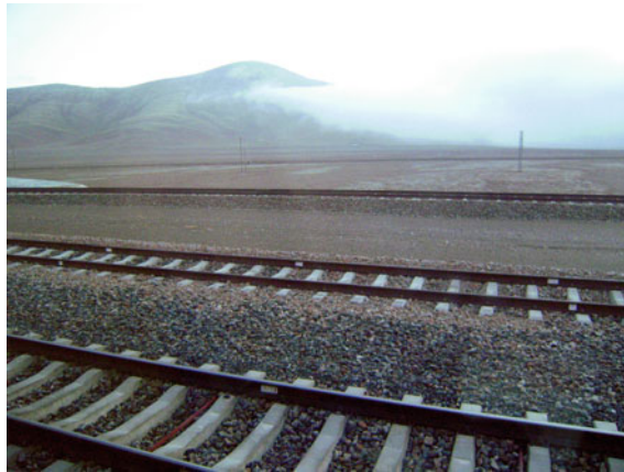
Fig. 6.50 The elevated gravel track bed is intended to preserve the stability of the ground temperature. Source Photograph by Yabin Song, provided by Xiufeng Yu
