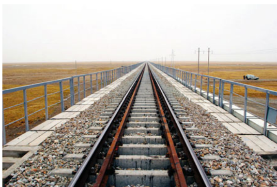
Fig. 6.43 The railroad extends to the horizon, which serves as a transportation artery for the area and increases the speed of freight transportation between Qinghai and Tibet. Source Photograph by Zhiguo Zheng, provided by Jiali Zhou
