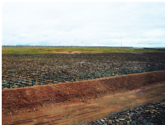
Fig. 6.51 The structural use of riprap for revetment and track beds can be seen over 80 % of the railway, which protects the railway from the potential damage due to the sinking and swelling of the permafrost below. Source Photograph by Ye Shen
