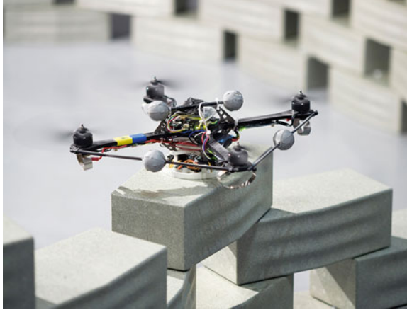
Fig. 1 The complex structure of the 1:100 installation has been assembled by autonomously flying “quadcopters” which land on a platform to pick up building elements and then set them down precisely on top of one another (Image by François Lauginie)
