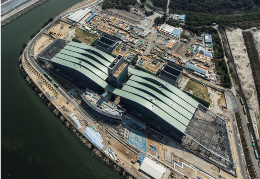
Fig. 5 The Hong Kong Sludge Treatment Facility adopts fluidised bed incineration technology to decompose sewage sludge at 850 °C in order to meet with the highest environmental requirements on air emission control. The plant is currently under construction (©Marcel Lam Photography)
