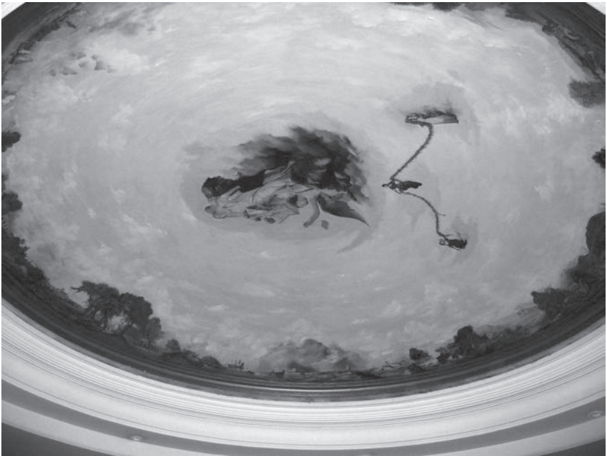
Figure 6.7 Ceiling detail, the lobby of Kūh-a Nūr Residence, Kāmrāniyyah District, 2000. Designed by Farzad Dalīrī. Photograph by author, 2007
