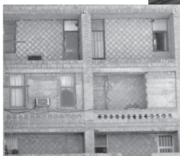
Figure 4.17 Altered façade with blocked veranda in Shūshtar New Town. Courtesy of S. Urdübādī, 2010
