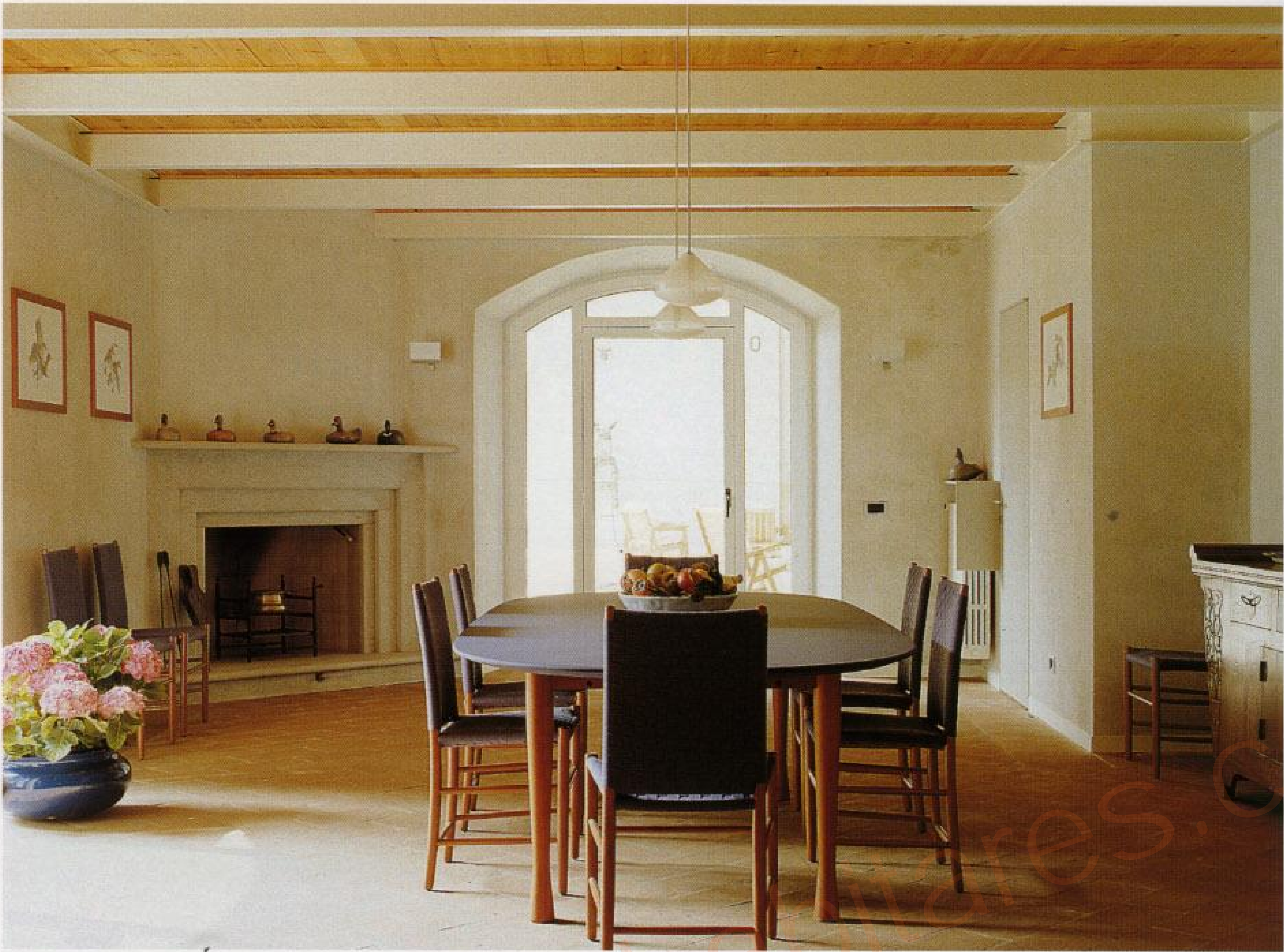
The original loadbearing structure made of wooden trusses has been treated with resins for conservation and reinforced with metal elements.
