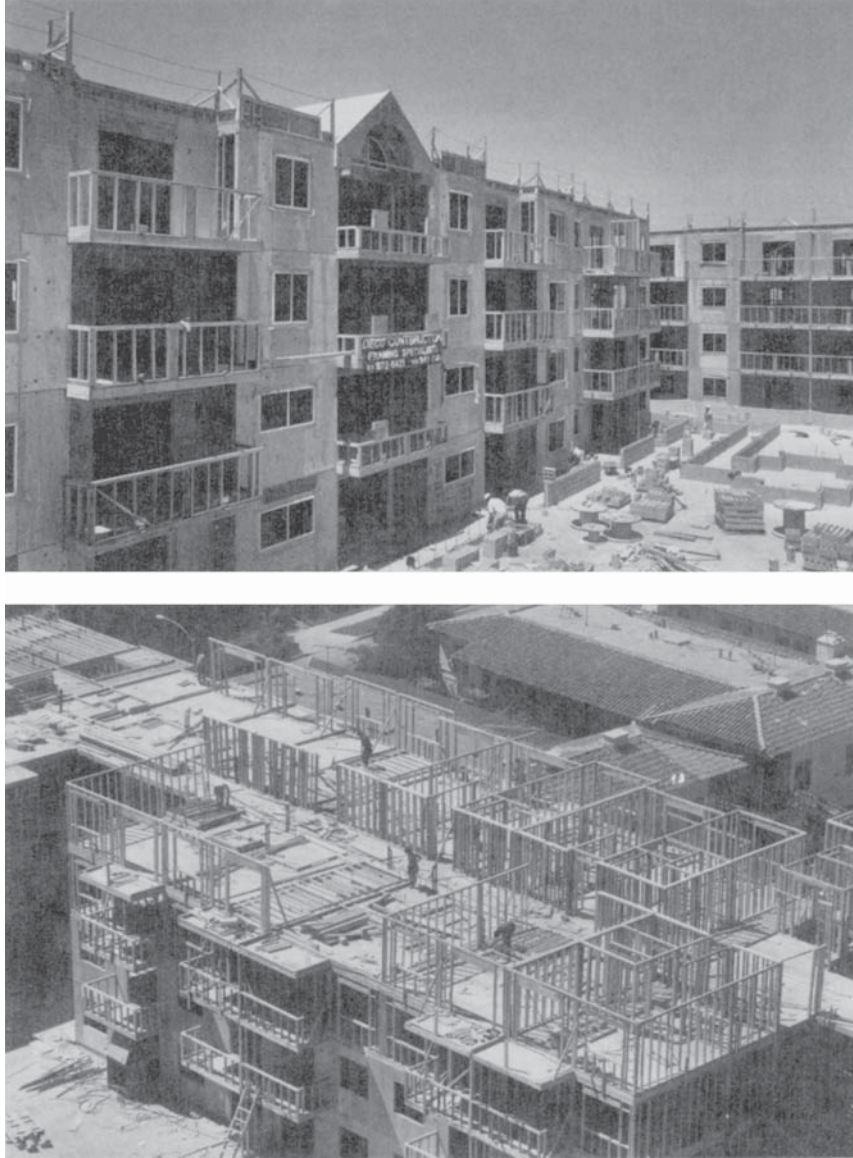
Figure 3.7 Four-story wood-frame building with diaphragms and shearwalls of plywood. (Photo courtesy of APA—The Engineered Wood Association.)
