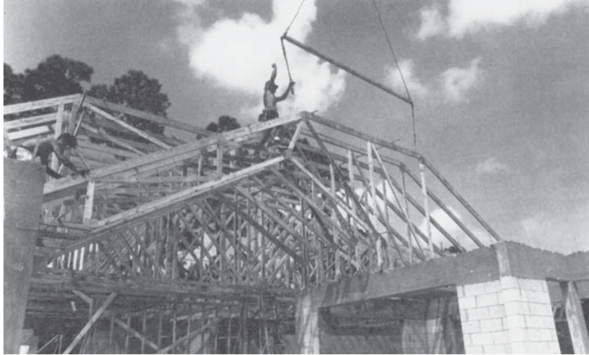
Figure 6.33b Metal plate connected trusses being placed in roof system supported on masonry walls. (Photo courtesy of Alpine Engineered Products, Inc.)
