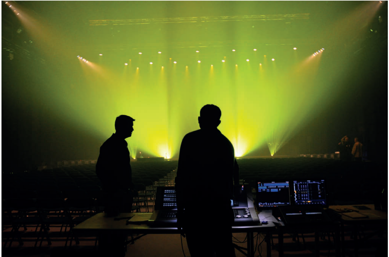
Figure 6.9 Backstage Centre, Purfleet, UK: lighting desk
