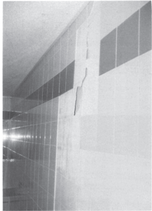
Plate 24. Damaged wall tiling. Wall tiles can be dislodged by differential movement, usually through shrinkage of cast concrete or concrete block backgrounds; normal good practice requires movement joints through the tiling to relieve these stresses.
