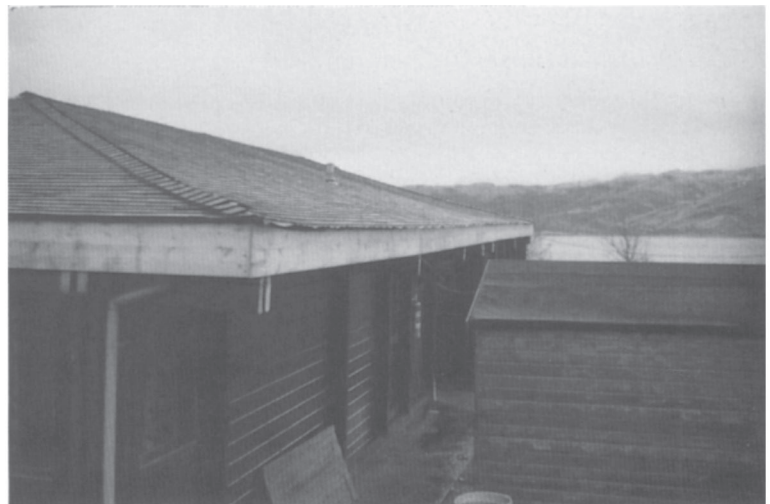
Plate 21. Water penetration in low pitch roofs. Low pitch roofs have poor resistance to rain penetration in windy conditions, even if closely bedded coverings are used such as the western red cedar shingles in this photograph; the sarking felt beneath the covering often gives temporary protection and problems may not develop for several years, usually at the eaves where the sarking felt deteriorates most rapidly.
