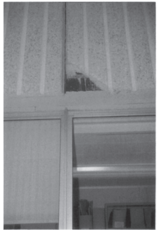
Plate 31. Fractures in concrete cladding. Fractures in concrete cladding are usually caused by reinforcement corrosion through inadequate cover, but in this case the panel was damaged during erection, partly because it was being handled too soon after casting and was rather weak.
