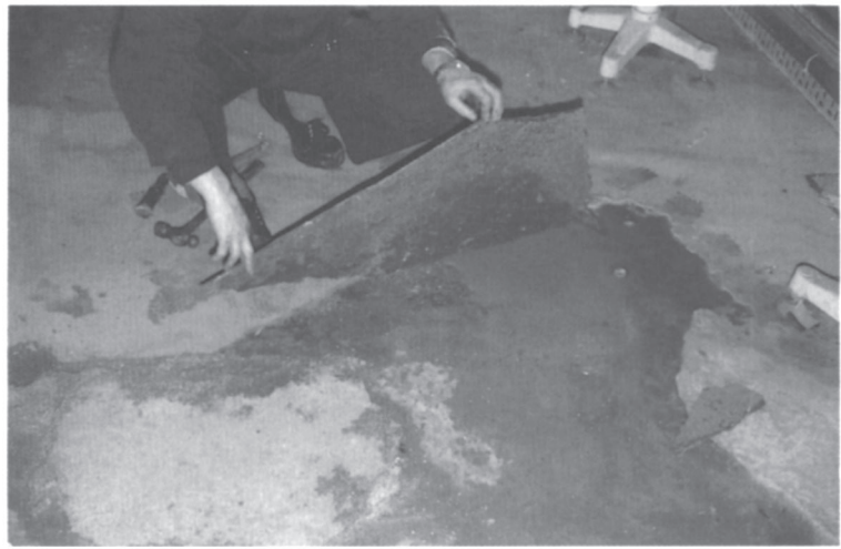
Plate 41. Failure of polymer-modified cement flooring. This polymer-modified cement and aggregate floor topping was laid in a bottling hall without movement joints, stresses causing fracturing and separation from the concrete base, but the floor topping also 'domed' beneath the syrup machines through expansion caused by sugar reaction with cement; cement-based flooring must never be used if sugar contamination is possible.
