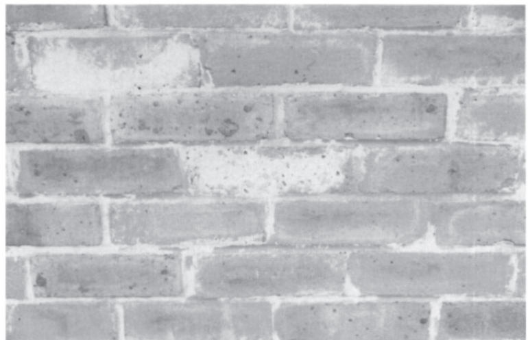
Plate 36. Sulphate efflorescence on bricks. Bricks containing excessive soluble sulphate often suffer from unsightly white efflorescence or crystallization, but the sulphate may react with the cement in the mortar joints to cause expansion and perhaps severe structural damage; sulphate resisting cement should always be used with bricks containing excessive sulphate.
