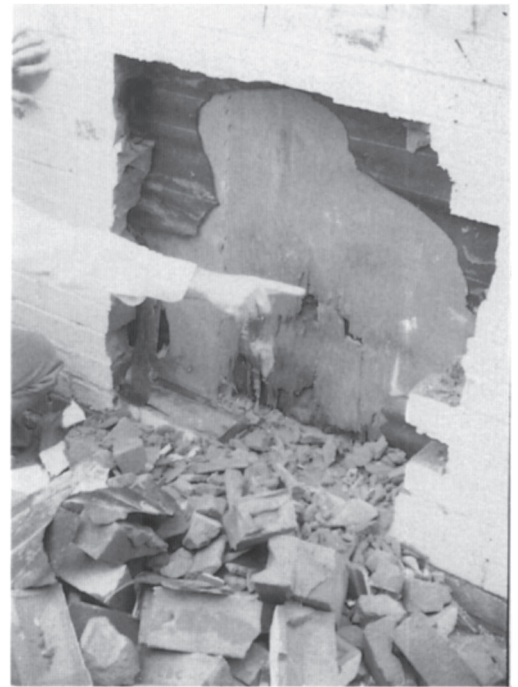
Plate 15. Fungal decay in modern buildings. Decay caused by interstitial condensation in the sheathing plywood on a timber frame house; condensation accumulated because the inner vapour barrier was damaged and the cavity between the sheathing plywood and the external brickwork cladding was unventilated. Decay due to condensation can also develop in floors laid on battens on concrete slabs if the floor space is not ventilated to the exterior; condensation is encouraged if the space is ventilated to the interior.
