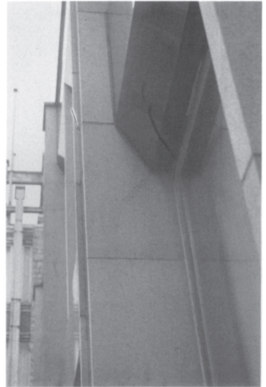
Plate 28. Stone cladding fractures. Fracturing of this granite cladding panel was caused by failure to continue the horizontal movement joint around the adjoining transom feature; the transom granite cladding also fractured.
