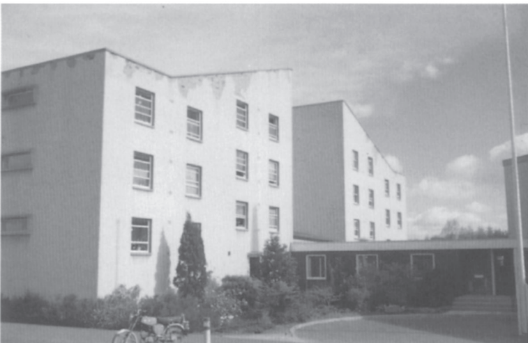
Plate 47. Render failure due to water penetration. The damp-proof course beneath the concrete wall copings was trimmed against the edge of the brickwork before rendering so that it did not protect the top edge of the render; water penetrating through the coping joints accumulated behind the render which became detached during frost.
