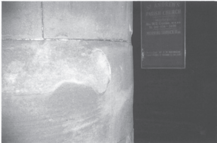
Plate 3. Stone erosion at St Andrew's Church, Glasgow. The carbonaceous sandstone columns absorbed acid rainwater which dissolved the carbonate binder and deposited calcium sulphate within the surface, stresses in the outer surface than causing it to separate from the weakened stone beneath.
