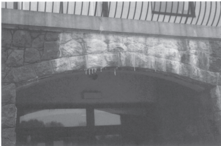
Plate 35. Lime deposits on masonry. These heavy lime deposits were caused by water saturating a semi-dry bed under paving on the flat roof above, the lime solution then emerging from the masonry through failure to provide an edge upturn to the roof damp-proof membrane beneath the paving.
