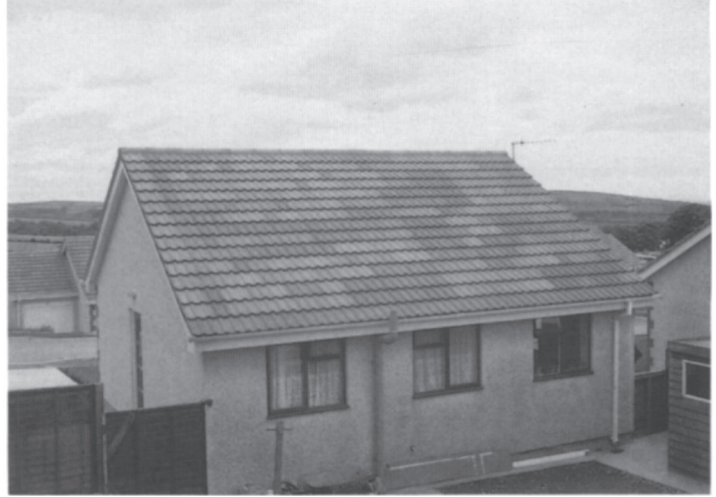
Plate 19. Concrete texture. The colour variation in these concrete tiles was caused by poor control of water content during manufacture, the lighter colour being due to excessive water and cement laitance on the surface.
