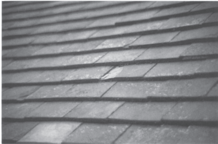
Plate 20. Frost spalling in clay roof tiles. Frost spalling is caused by prolonged retention of water by microporous tiles which are more likely to be saturated in freezing conditions. Microporosity is often associated with light coloured underfired tiles; similar failures occur in clay bricks.
