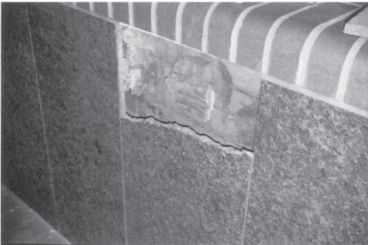
Plate 29. Stone cladding fractures. Fracturing of this granite cladding panel was due to expansion of positioning dabs; gypsum plaster was used to thicken the cement mix, water vapour absorption subsequently causing sulphate attack of the cement, expansion of the dabs and fractures of the cladding.
