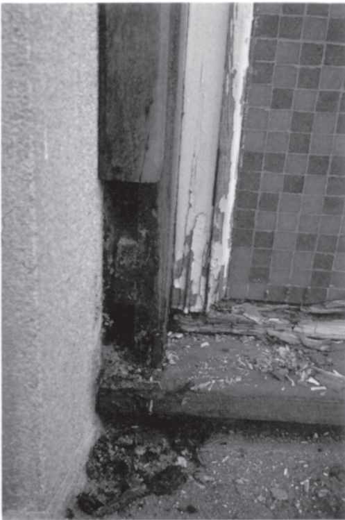
Plate 16. Fungal decay in joinery (millwork). Water absorption through end-grain surfaces can cause decay in untreated wood joinery, decay in susceptible wood often spreading to resistant wood.
