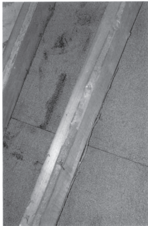
Plate 12. Bark borer damage on a softwood rafter. The Bark borer Ernobius mollis causes damage which is often confused with Common Furniture beetle, but Bark borer is confined to the bark and the wood just beneath it and remains active for only about two years after a tree is felled so that treatment is not required.
