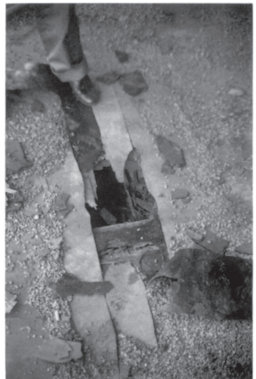
Plate 17. Fungal decay in flat roofs. Interstitial condensation in roof decking often causes fungal decay damage; condensation can be avoided by ventilating the space between the decking and the ceiling insulation in order to disperse moisture diffusing from the accommodation.
