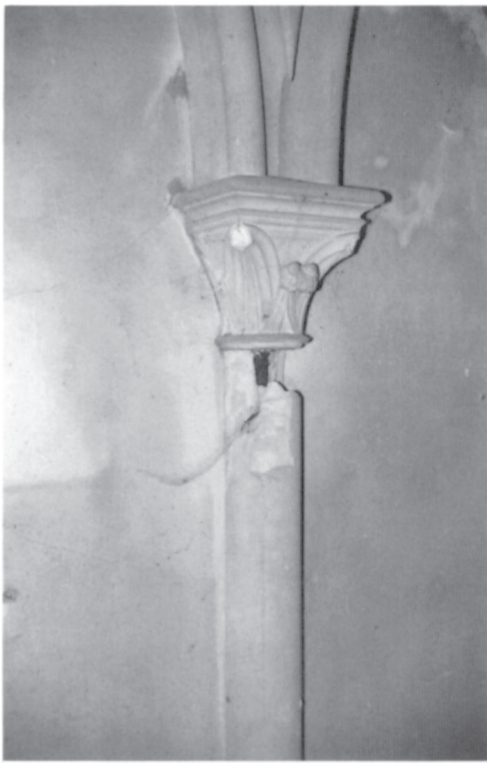
Plate 9. Metal corrosion damage to stone and concrete. Corrosion of ferrous dowels and cramps in masonry and steel reinforcement in concrete causes expansion and spalling damage.
