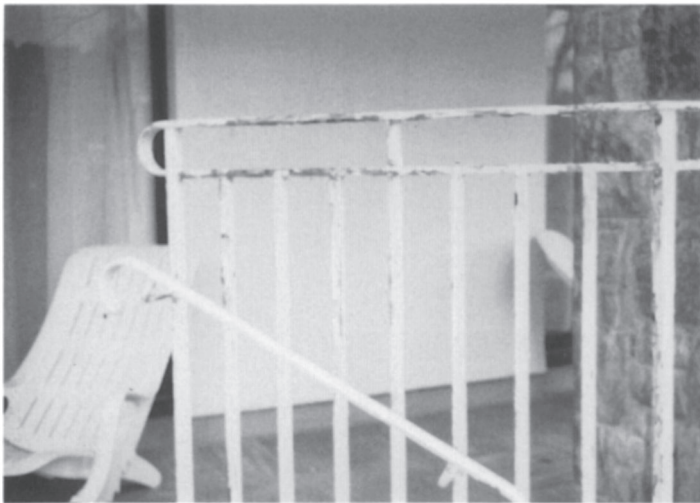
Plate 27. Corrosion of steel railings. Corrosion developed on these steel railings shortly after erection and decoration; a zinc-rich primer had been used to inhibit corrosion but it is only effective if applied to clean steel, and in this case it was applied over mill scale, old red oxide primer and rust.
