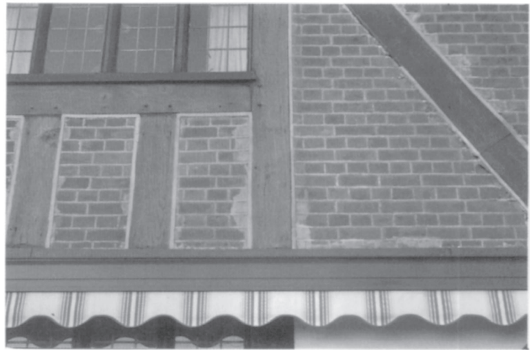
Plate 46. Differential movement between brickwork and wood. In dry weather shrinkage of the wood frame formed a gap which was then pointed with mortar, but subsequent expansion of the wood caused spalling of the adjacent brickwork.
