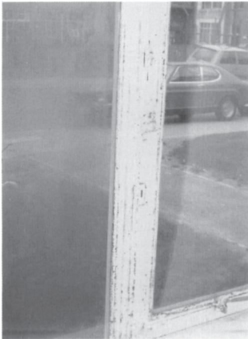
Plate 43. Condensation in sealed doubleglazing. Condensation within these double glazing units was due to defective seals; stepped units were involved and the defective seals allowed warm humid air from the accommodation to enter the units, causing condensation on the inner surface of the outer glass.
