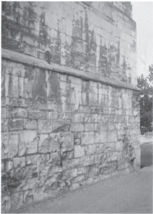
Plate 1. Frost damage affecting stone masonry at Lincoln Cathedral. The stone was normally durable but suffered frost damage where it was affected by rising dampness and therefore had a high moisture content in freezing conditions.
