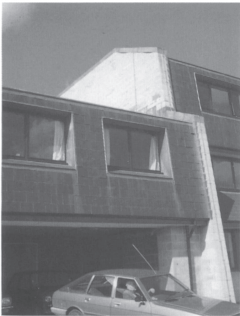
Plate 33. Water penetration in a new cast stone building. Cast stone is usually manufactured using a semi-dry mix to give an interesting surface texture but it is difficult to compact and is often very porous; water penetration into porous cast stone in this case caused flooding of the trays over windows and lower roof extensions with severe dampness internally.
