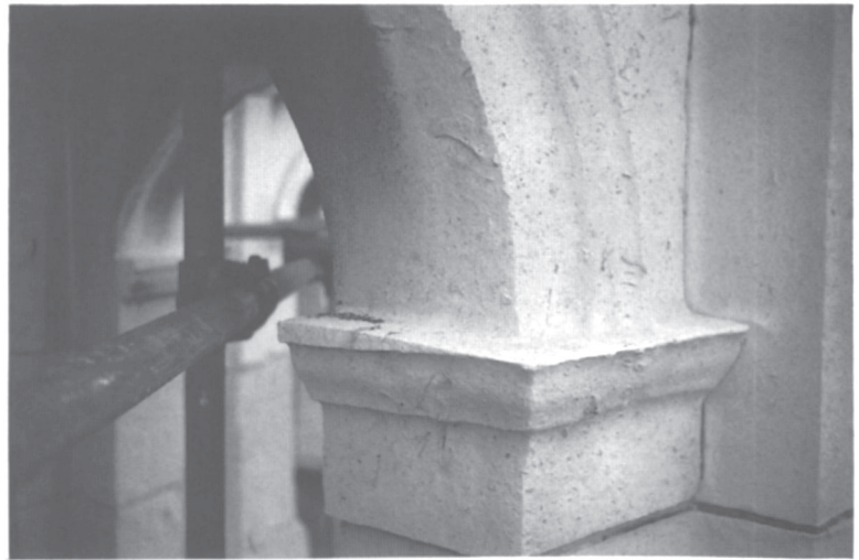
Plate 2. Stone erosion at St Paul's Cathedral, London. The Portland limestone was protected within the arch, but horizontal surfaces were slowly eroded where they were exposed to rainfall containing dissolved pollutant gases.
