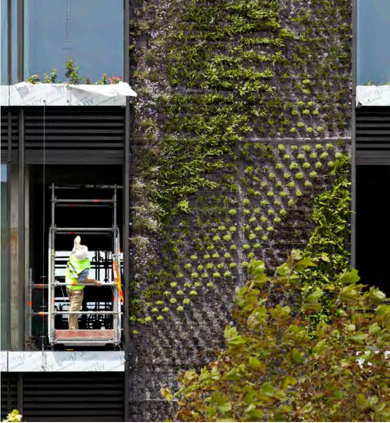
Patrick Blanc, vertical garden for Jean Nouvel's One Central Park under construction, 2013.
